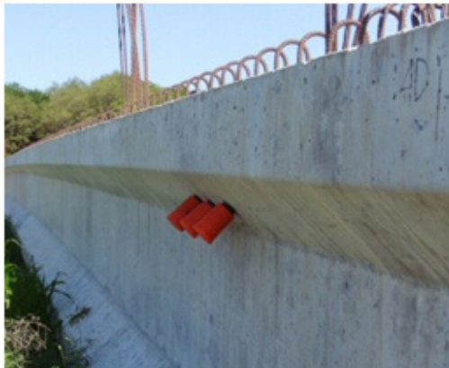
Figure 5. Humidity probes enclosed in plastic covers.
