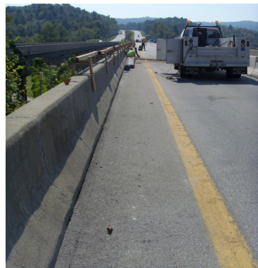
Figure 10. Overview of treatment site.
