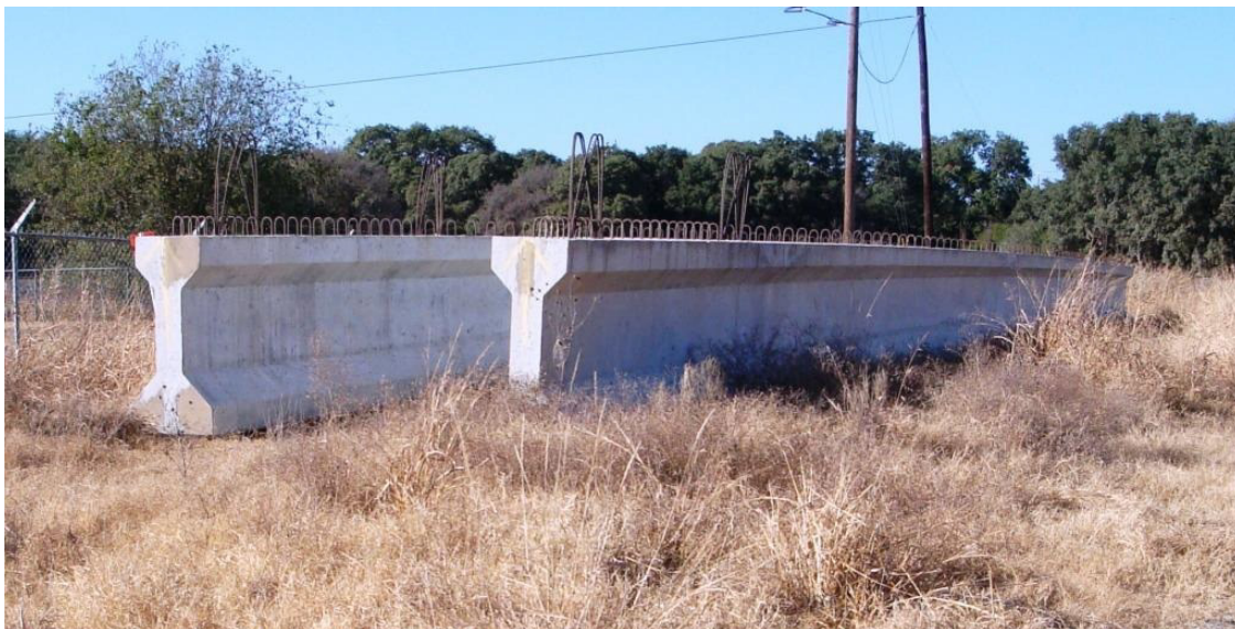
Figure 2. View of precast girders in New Braunfels, Texas, prior to treatment. Only two out of four girders are shown.
