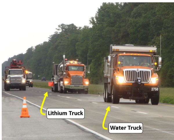
Figure 1. Treatment of concrete pavement in Georgetown, Delaware. Water application (first vehicle) followed by lithium application (second vehicle). Third vehicle with second pass of water not shown.
