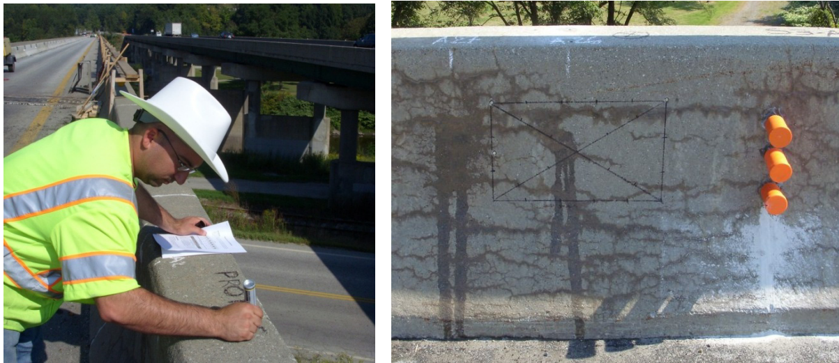
Figure 9. Worker labeling the treatment on the bridge wall (left); instrumentation site with crack mapping, expansion, and humidity sites for data collection (right).
