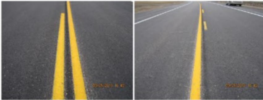
Figure 2 J-Band US 169. Some material loss along joint.
