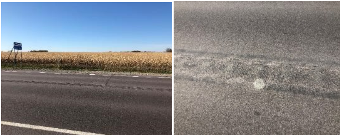
Figure 24. VRAM section on TH 22 between the cemetery near 179th Street and 169th Street
