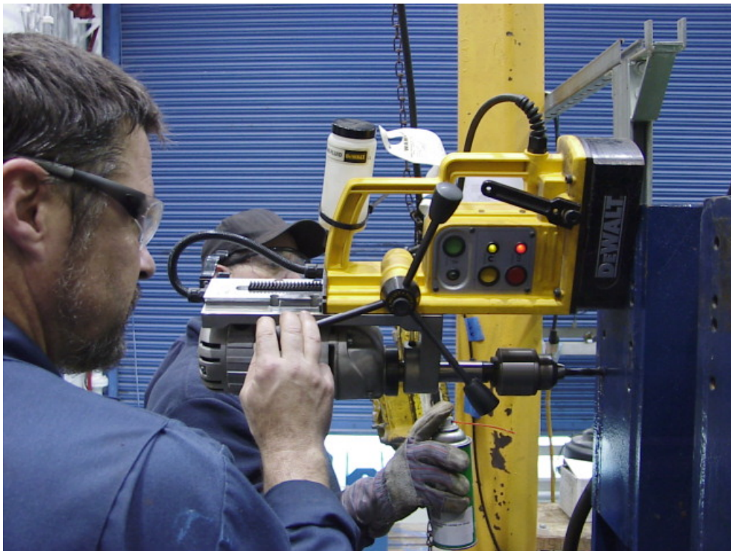
Figure 7. Photo of New Hole Drilling on Axial Load Support Assembly Column Beam
