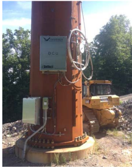
Figure 15. The DCU Installed on Transmission Tower [6]
