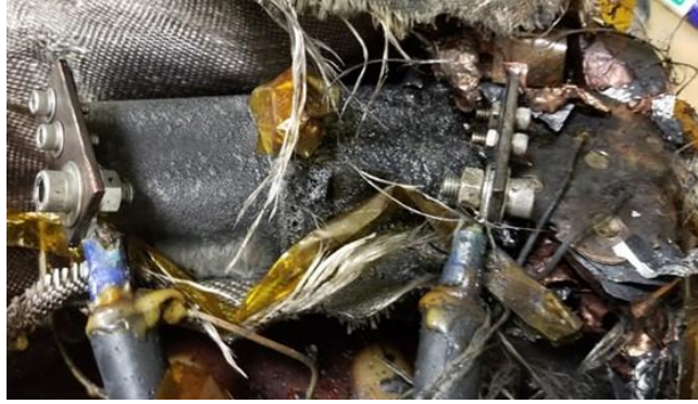
Figure 57. Evidence of venting and fire, in BL battery from external short test
