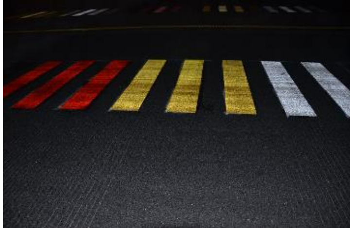
Figure 66. Rubber Deposits on Preformed Thermoplastic Surface Markings One Week After Installation
