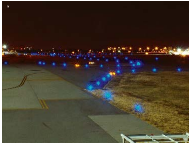
Figure 2. Blue taxiway edge lights installed on both sides of taxiway pavement area (source: http://www.airportsinternational.com , 2017)
