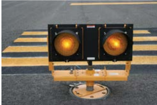
Figure 3. ERGL installed on either side of the taxiway near the holding position sign (source: http://www.lrc.rpi.edu )
