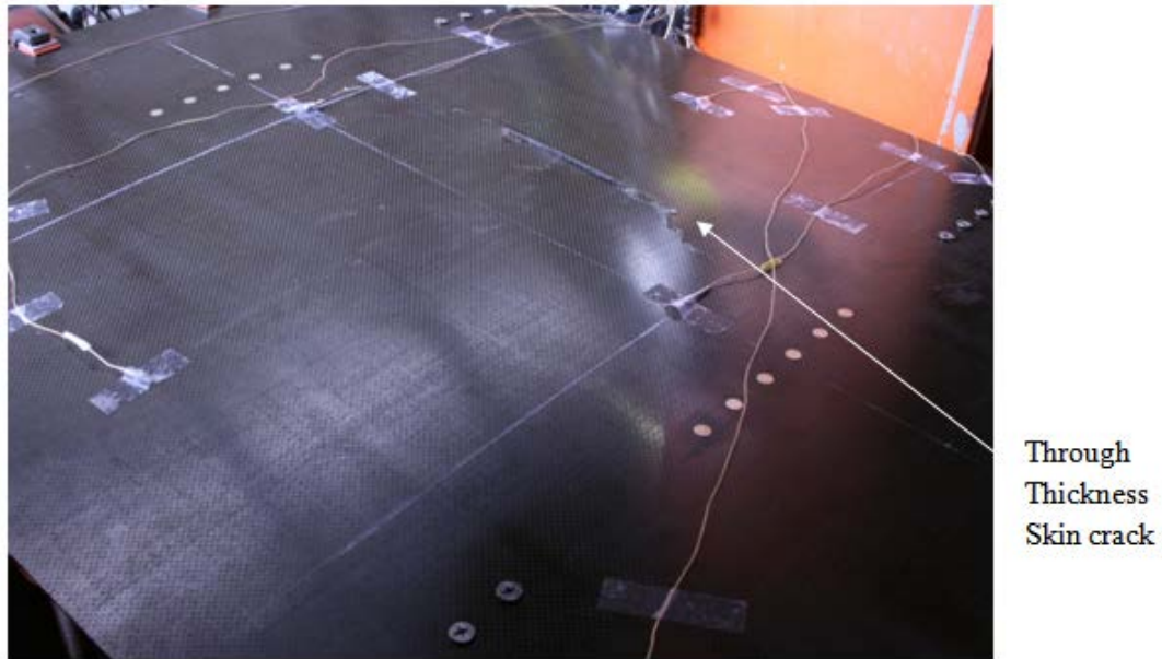
Figure 32. Post-test state of Stringer05 showing surface cracks along the skin-stringer connection at the impact location
