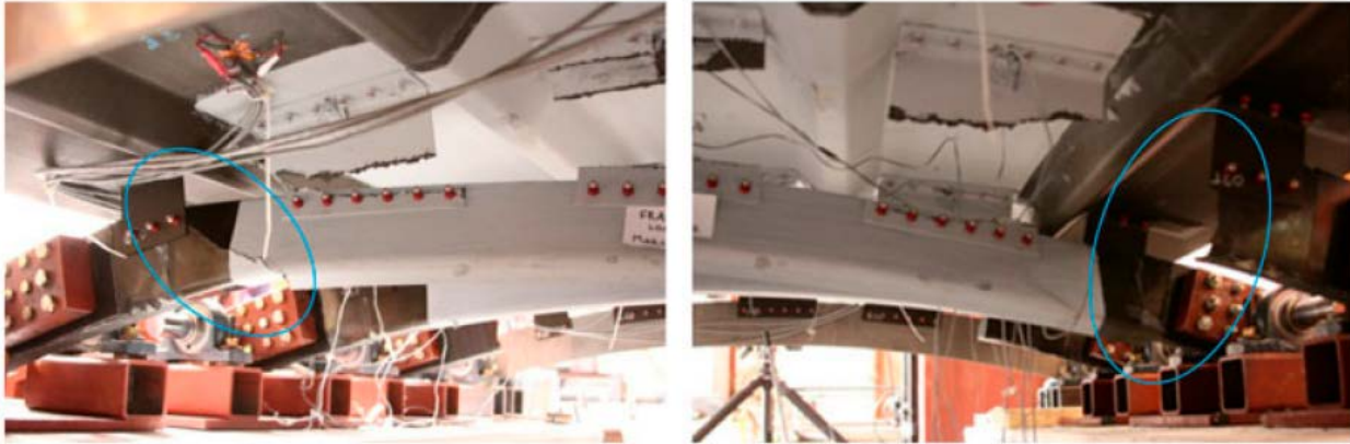
Figure 49. Frame03 C-frame fracture failures near boundary supports
