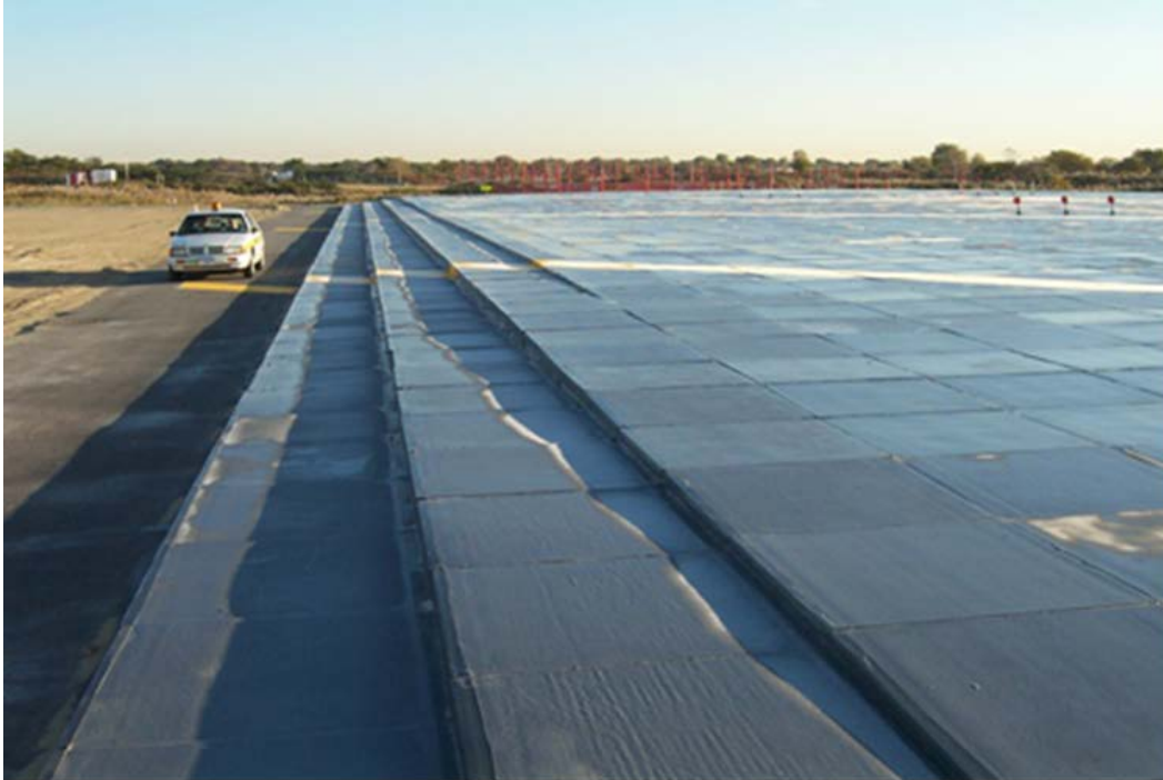
Figure 46. The JBR EMAS Replacement at JFK
