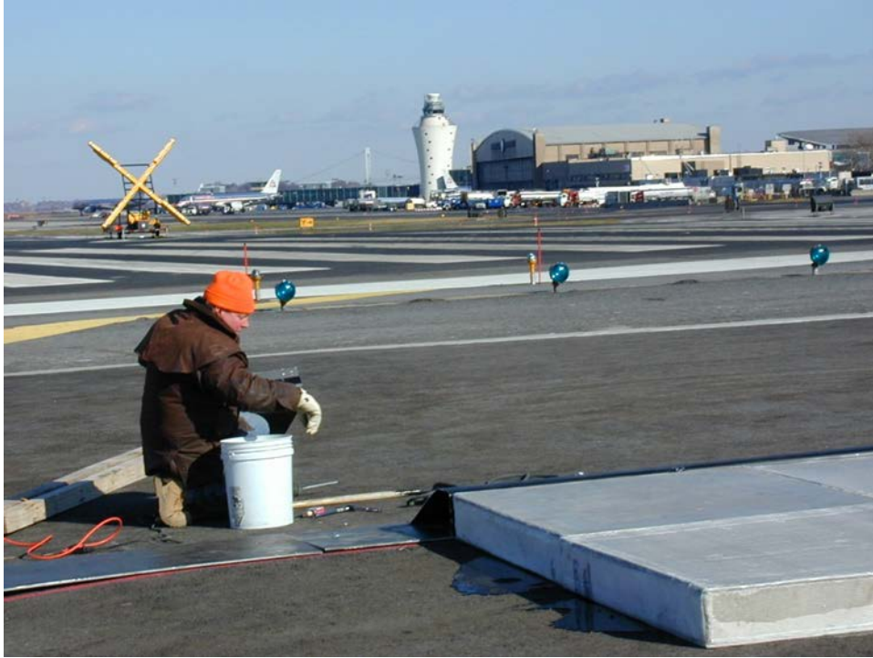
Figure 37. Leading Edge of JBR Blocks Were 75-ft From Departure End of LGA Runway 4
