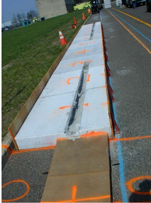
Figure 44. Wheel Ruts From the Small-Wheel Test Through the JBR Blocks
