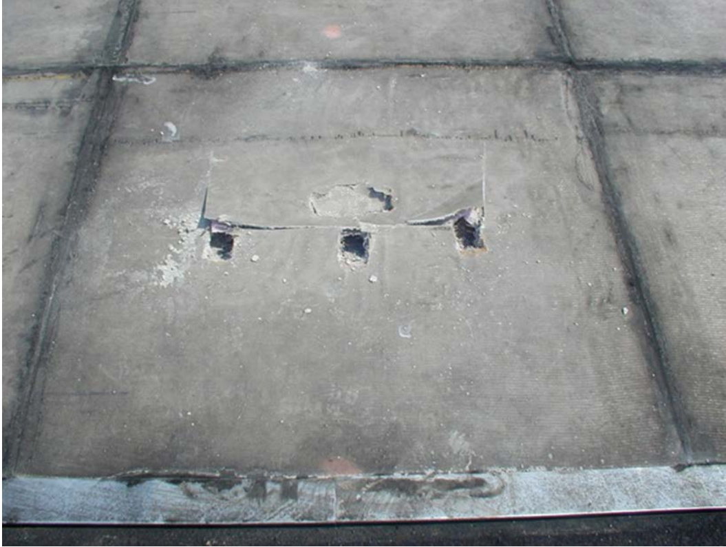
Figure 42. Intentional Damage to JBR System
