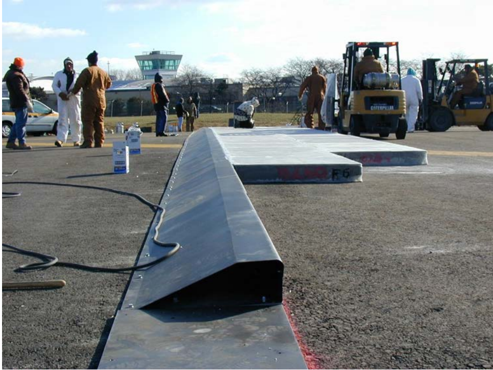
Figure 35. Aluminum Debris Deflector at Leading Edge of JBR Blocks at LGA
