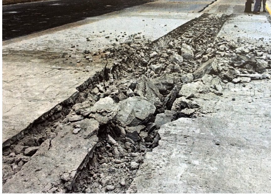
Figure 4. Foamed Concrete Test Bed Mode of Failure
