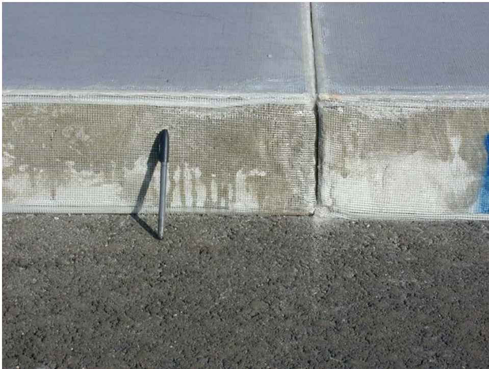
Figure 36. Typical 8-in.-Deep JBR Block Showing Rigid Boards at Top and Bottom and Mesh Scrim
