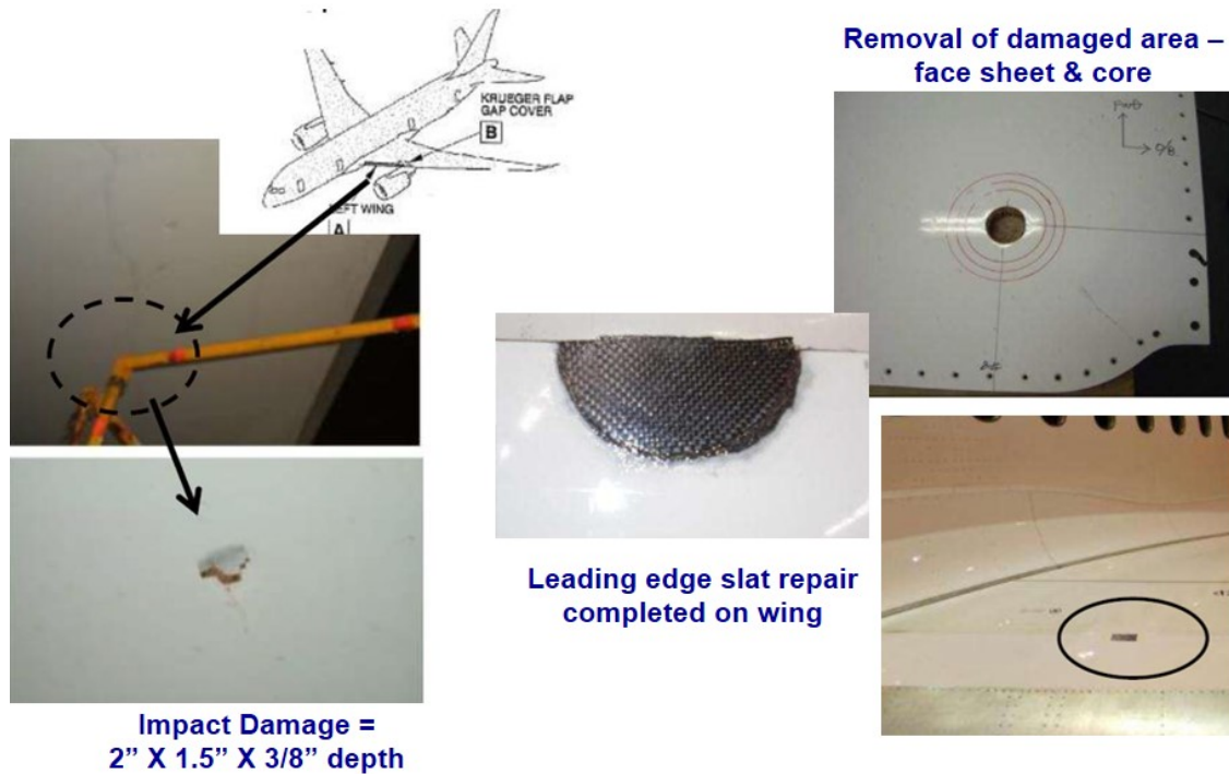
Figure 210. Accidental damage from ground handling equipment
