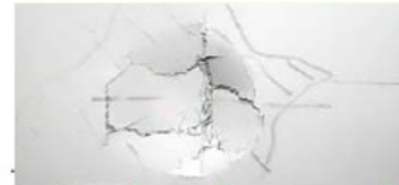
Dent and surface cracking
