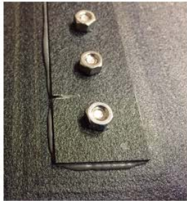
Grinder Cut *Cracked or broken substructure
