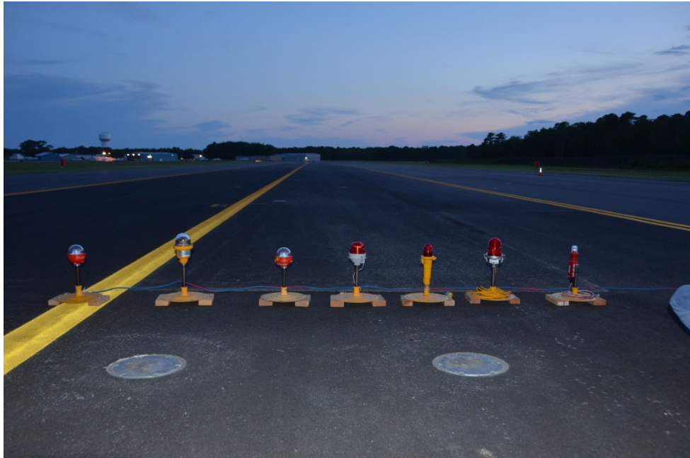
Figure 13. The L-810 Fixtures Evaluated at WWD
