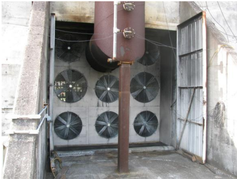
Figure 7. Airflow Exiting Hangar Through Fans
