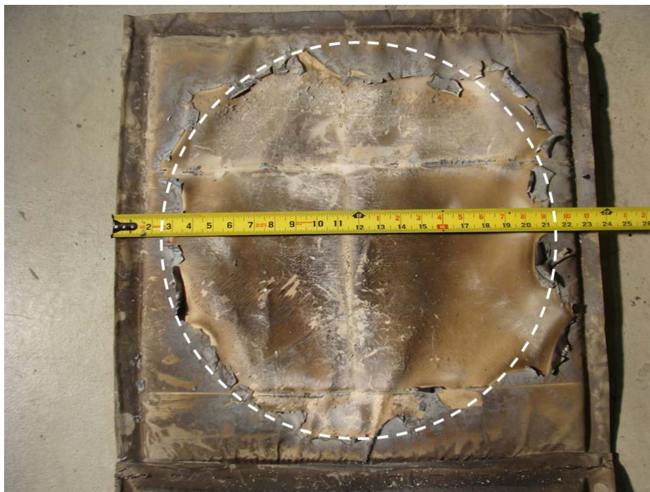
Figure 45. The damage area is shown for the white material: diameter of damaged area = 19" = 48.26 cm, radius = 24.1 cm
