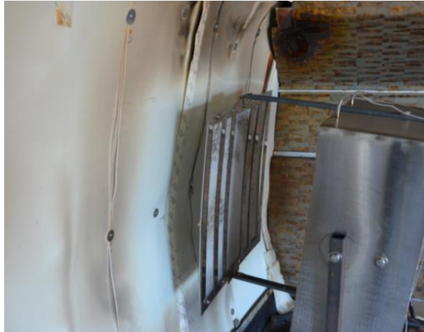
Figure 44. Damage to Interior: Test 6
