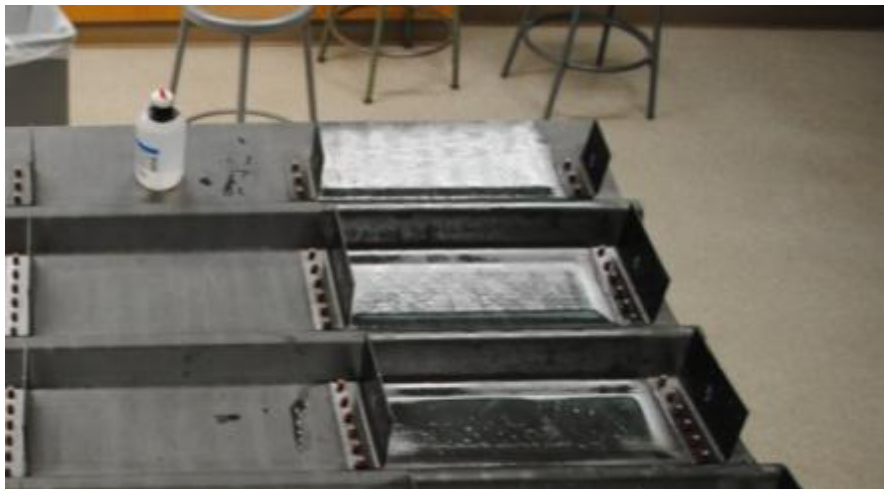
Figure 44. Conditioning and neutralizing the backside of the panel for bonding FO lines
