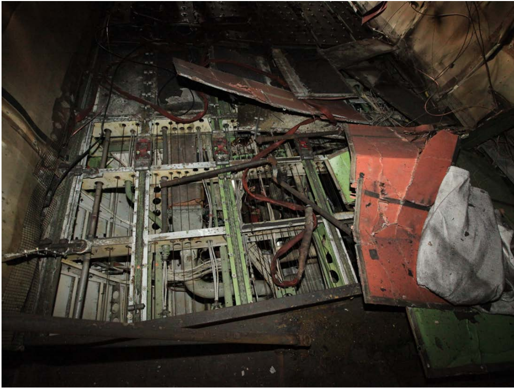
Figure 20. Hole in floor above the mix bay
