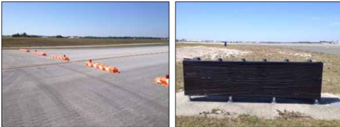
Figure 9. Barricades on Taxiway and Sign Wrapped in Black Visqueen Screen
