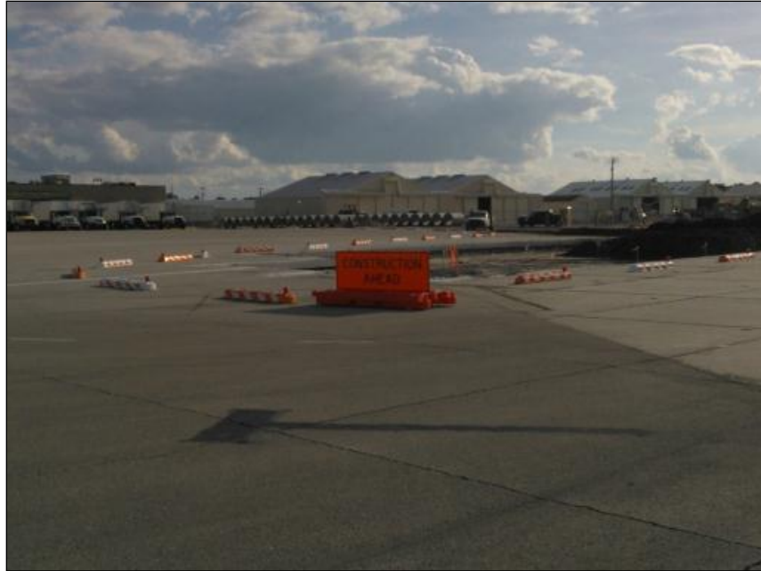
Figure 57. CONSTRUCTION AHEAD Sign on North Side of the Terminal Apron at SFB
