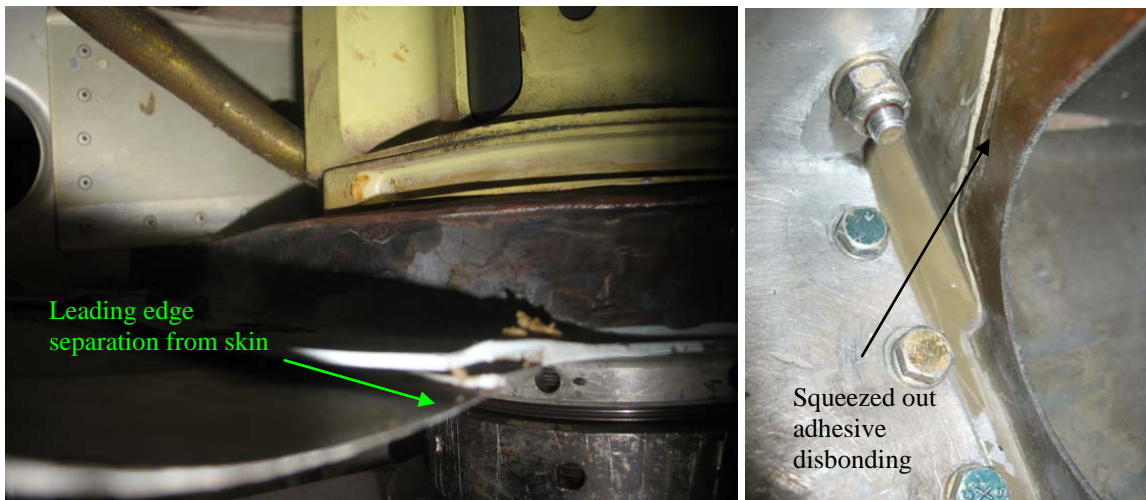
Local buckling of leading edge between rivets ruptured filler material (orange color)
