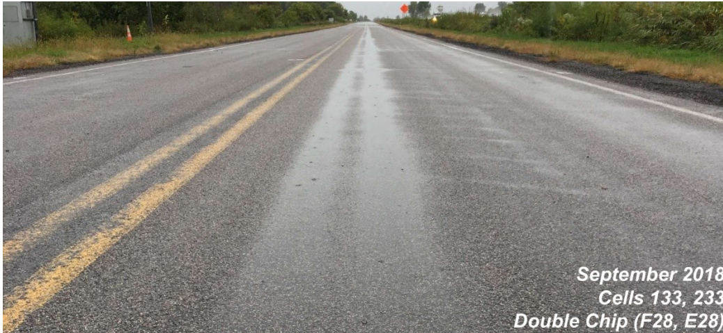
Figure 31. Condition photo showing rutting in double chip sealed CCPR sections at MnROAD
