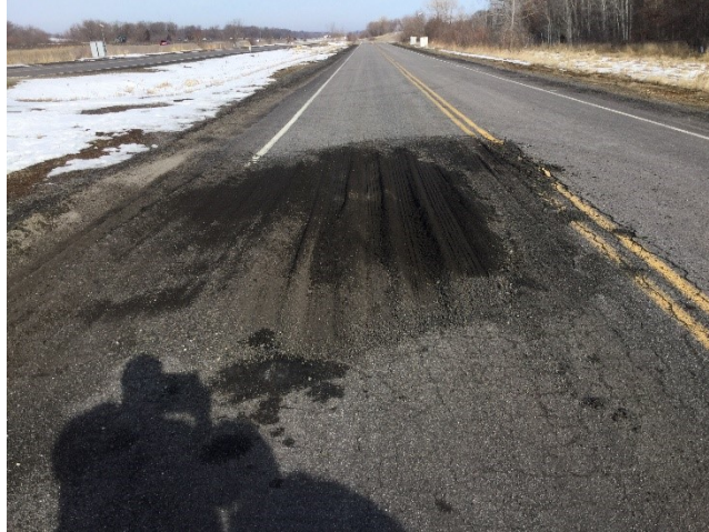
Figure 28 Failed pavement in MnROAD Cell 233 due to potential subgrade/culvert issues
