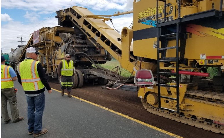
Figure 5 CIR process from project along County State Aid Highway (CSAH) 11 in Chisago Co., MN
