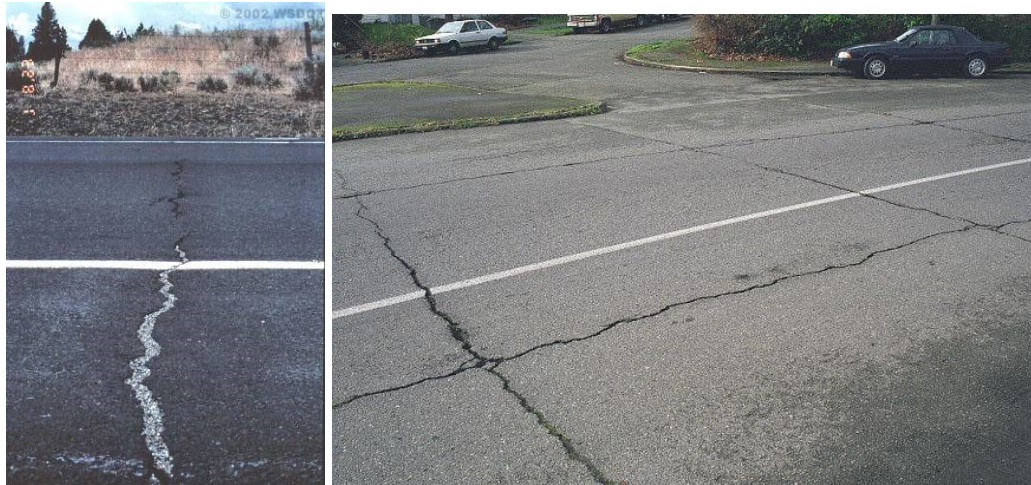
(a) Thermal Cracking
