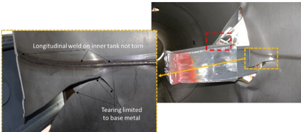
Figure 23. Interior View of Tank from East Side with Inset Showing Longitudinal Weld on Inner Tank (Prior to Impactor Removal)
