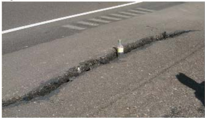
Figure 3 – Settlement Cracks in Shoulder
