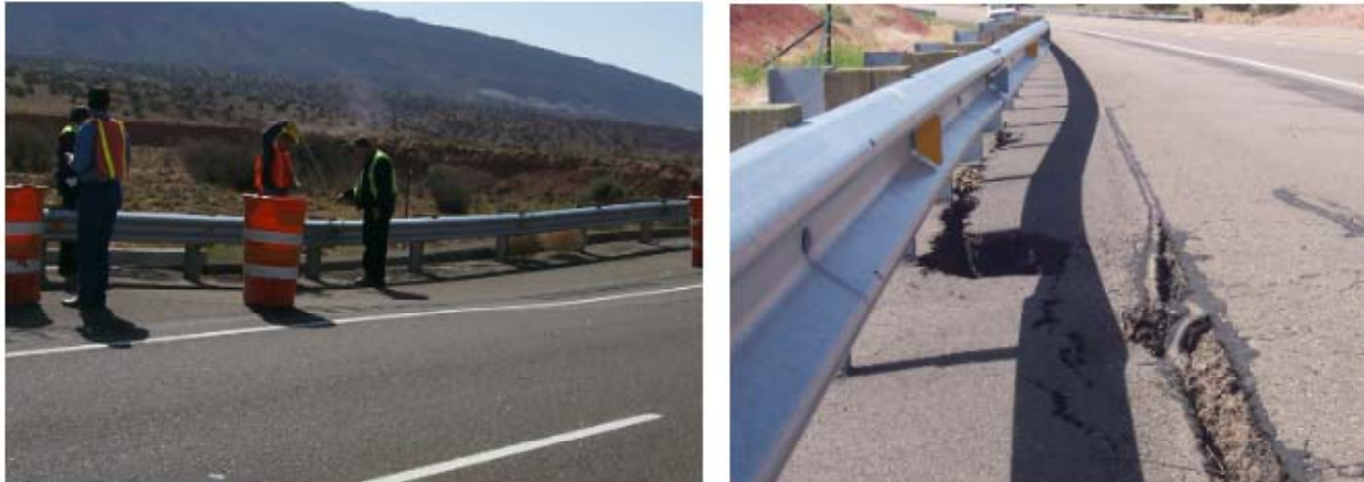
Figure 4 - Settlement at Culverts, Slope Failure
