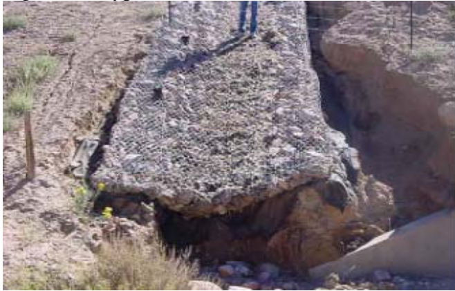
Figure 1 – Typical Erosion at Rundowns
