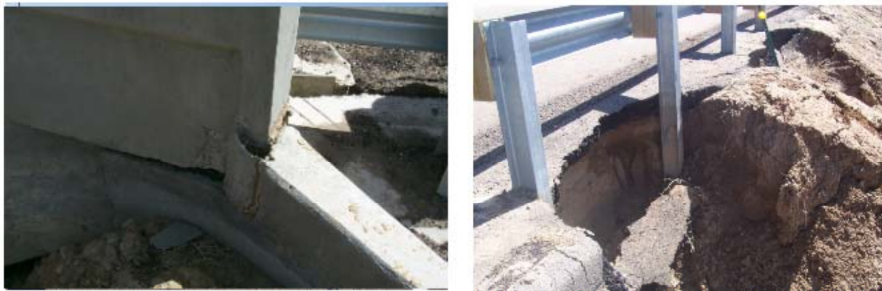
Figure 5 – Erosion at Bridge and Embankment
