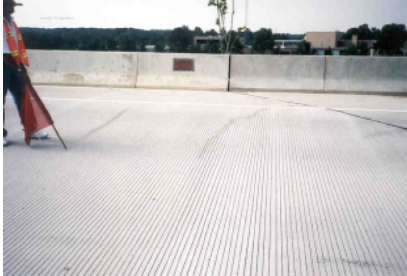
Figure 103. Wide view of deck cracks at the bridge end (Bridge No. 1143-466).
