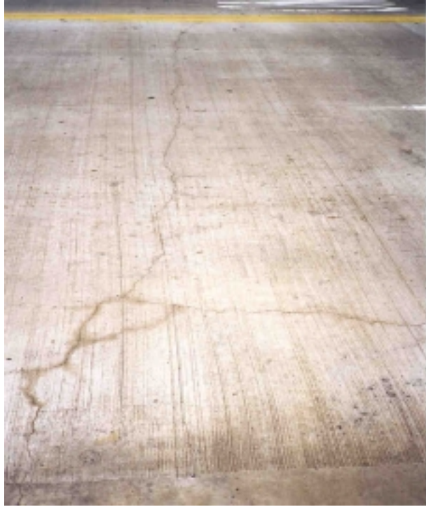
Figure 100. Transverse cracks on the deck (Bridge No.1130-153).
