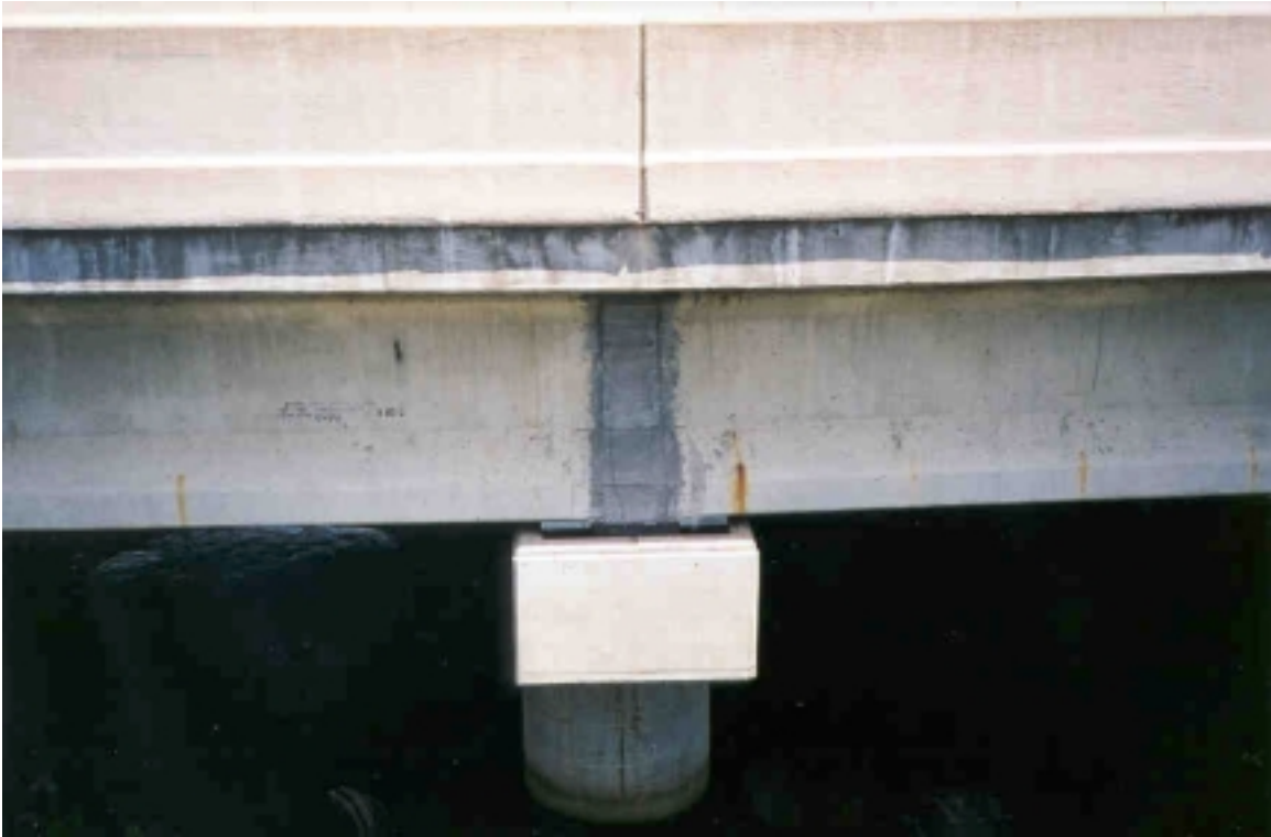
Figure 17. Watson Creek Bridge (West Bound): Cracked continuity joints (bridge No.1130-152).
