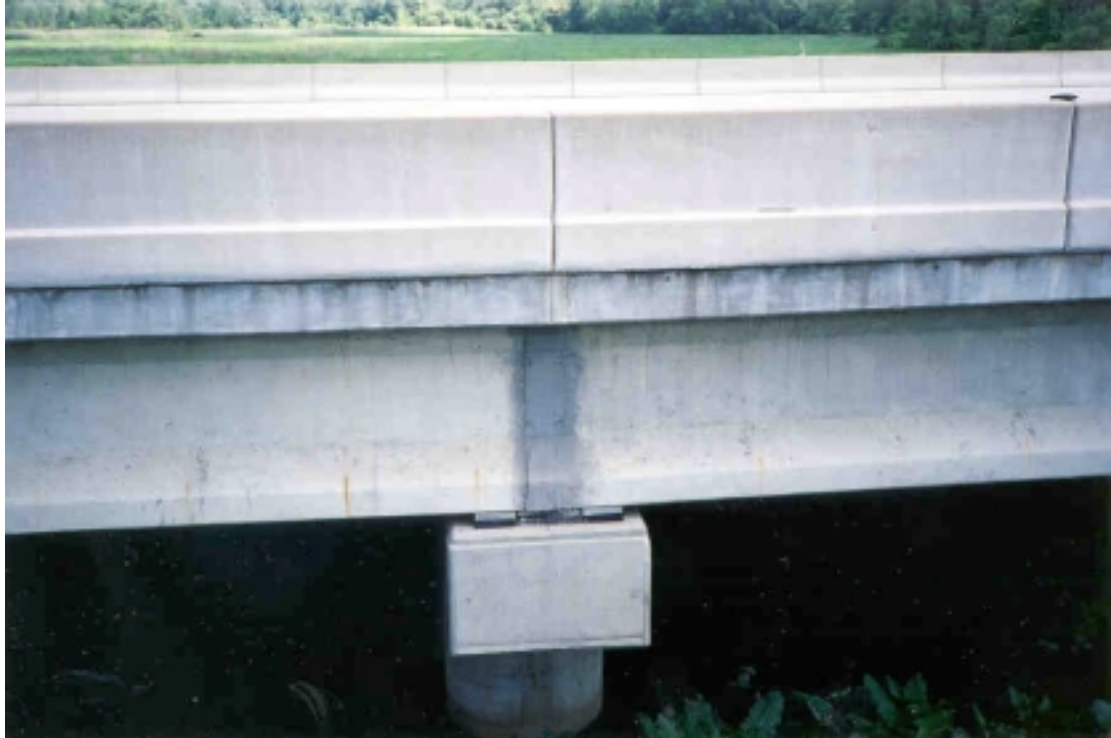
Figure 97. Cracked continuity joint (Bridge No. 1130-152).
