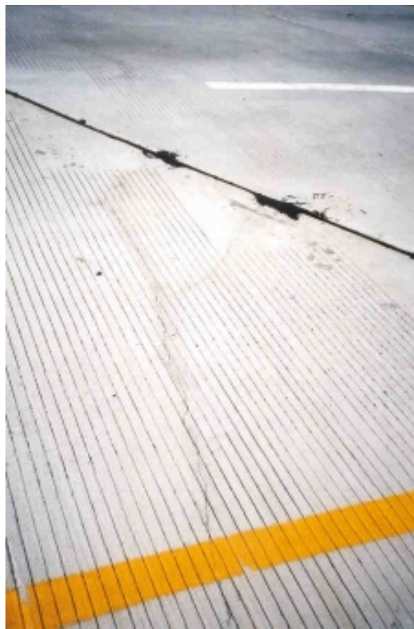
Figure 104. Close view of a crack (Bridge No. 1143-166).
