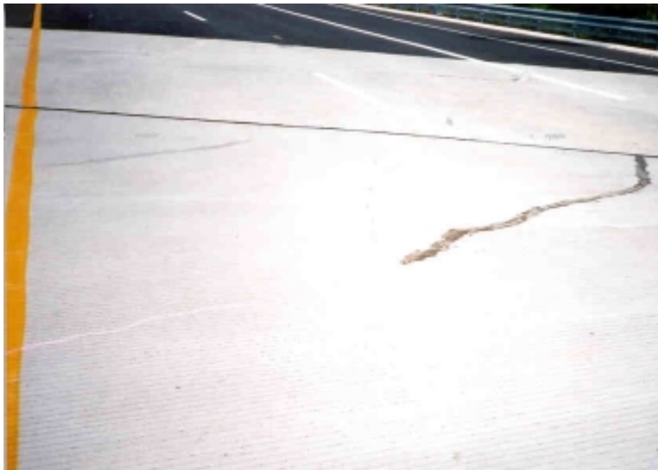
Figure 110. Cracks on the deck (Bridge No.1143-171).
