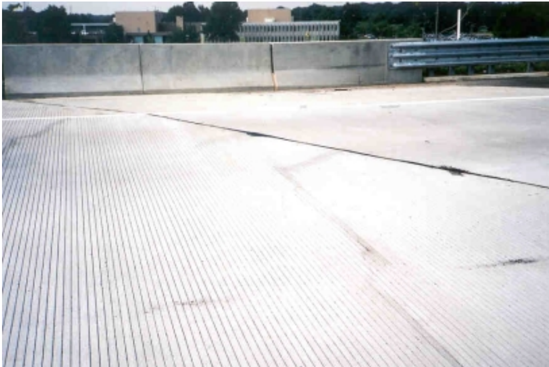
Figure 102. Deck cracks at the bridge end (Bridge No. 1143-466).
