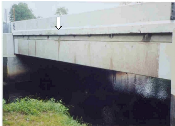
Figure 1. Corrosion due to transverse deck cracks in a bridge in New Jersey.
