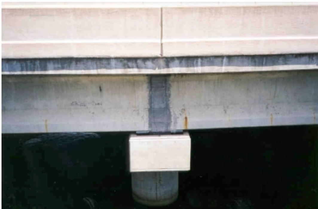
Figure 98. Another cracked continuity joint (Bridge No.1130-152).
