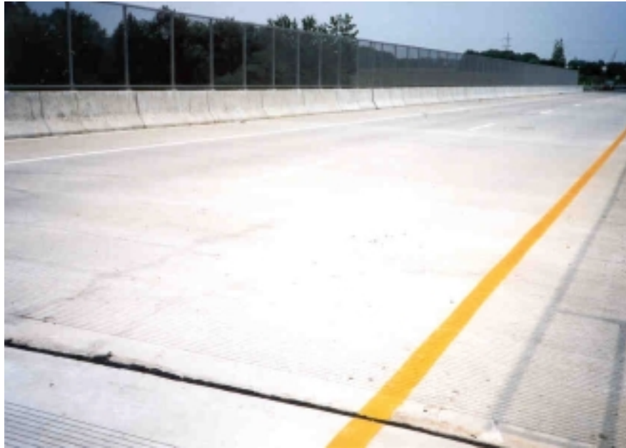
Figure 116. Transverse (and longitudinal) cracks on deck (Bridge No.1143-177).
