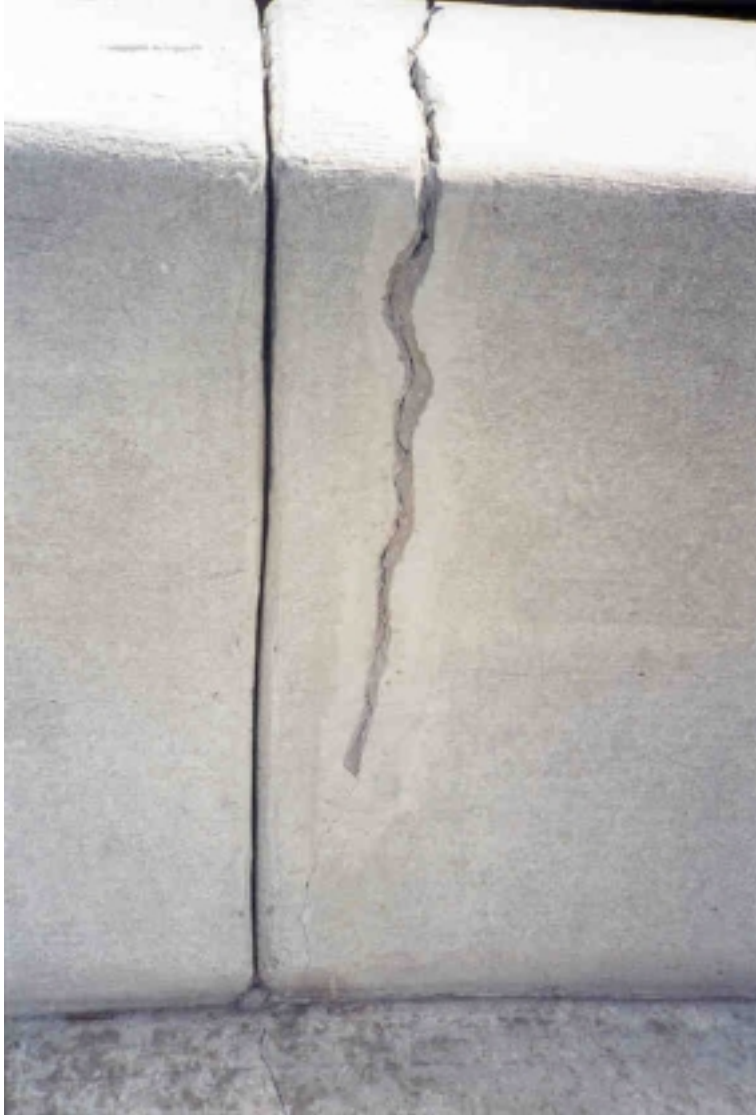
Figure 94. Crack on deck and parapet (Bridge No. 0173-151).
