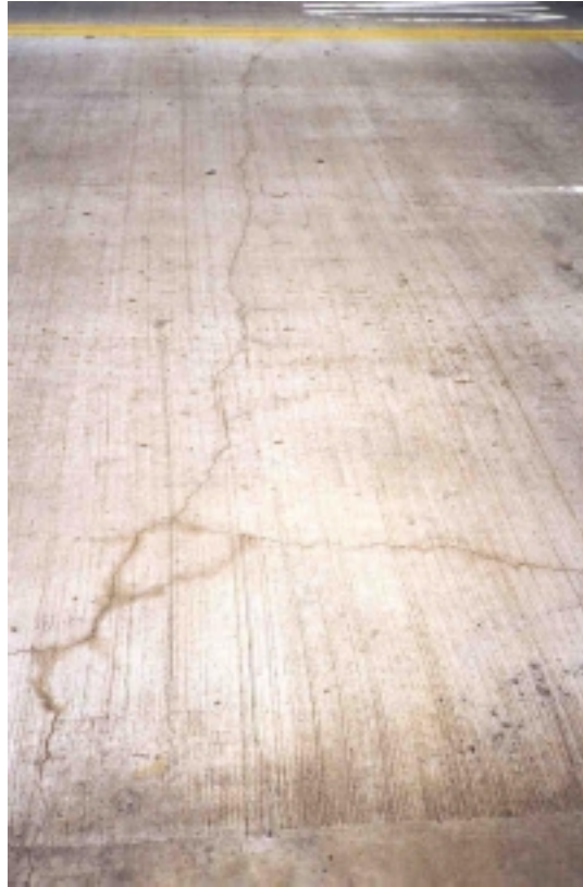
Figure 2. Transverse deck cracks on a bridge deck in New Jersey.
