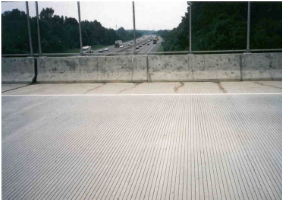
Figure 115. Transverse deck cracks on Bridge No.1143-176 (NJ Turnpike in the background).
