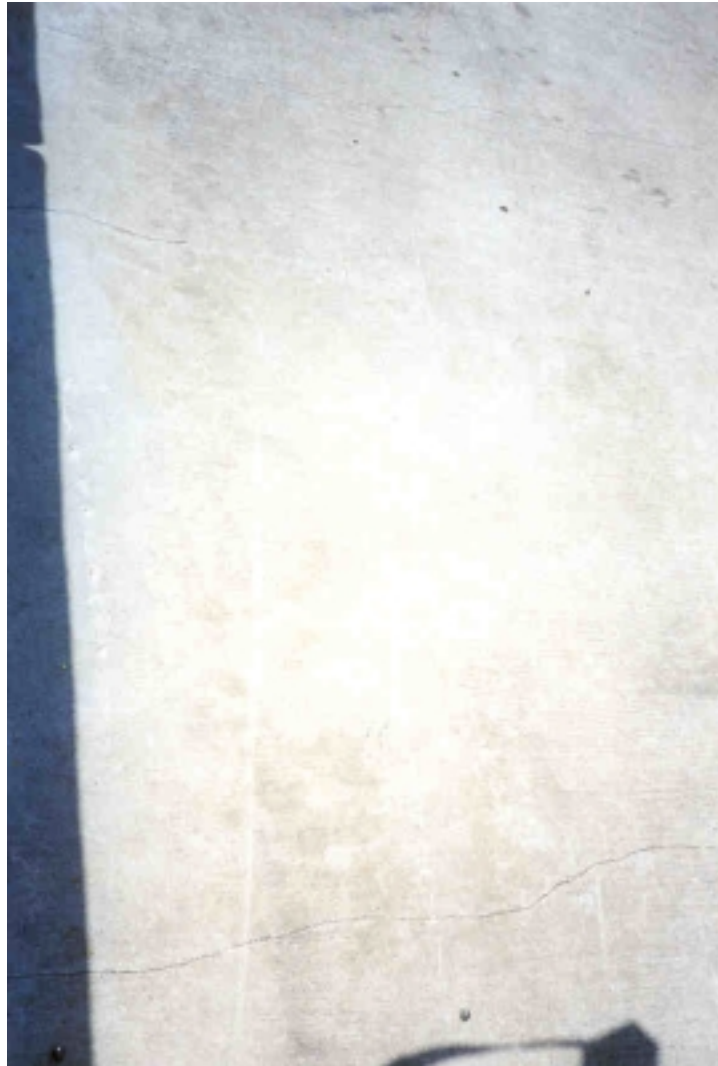
Figure 90. Crack on the deck (Bridge No 0713-151).
