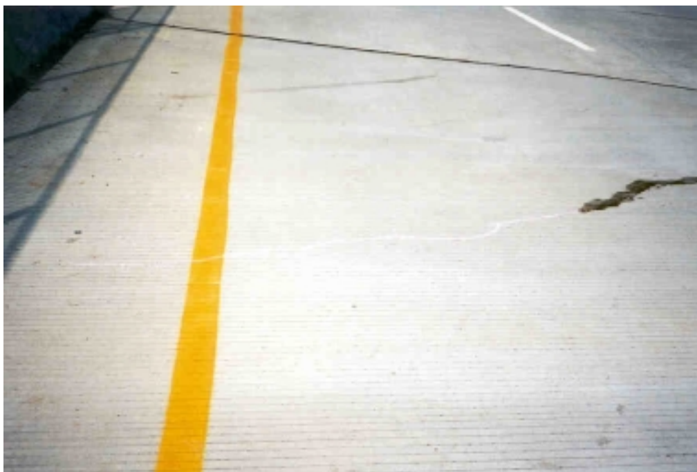
Figure 111. Another marked crack on the deck (Bridge No.1143-171).
