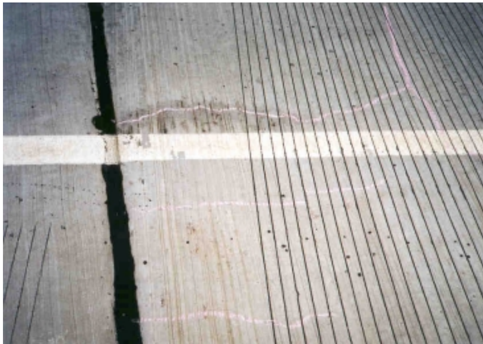
Figure 112. Close up view of deck cracks at the ends (Bridge No.1143-172).
