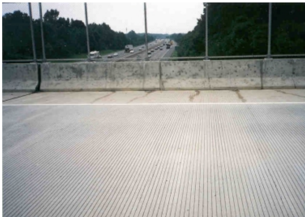
Figure 16. Rt. 133 bridge deck crack.
