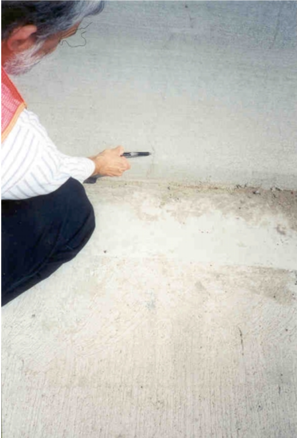
Figure 93. Crack extending into the parapet (Bridge No. 0713-151).
