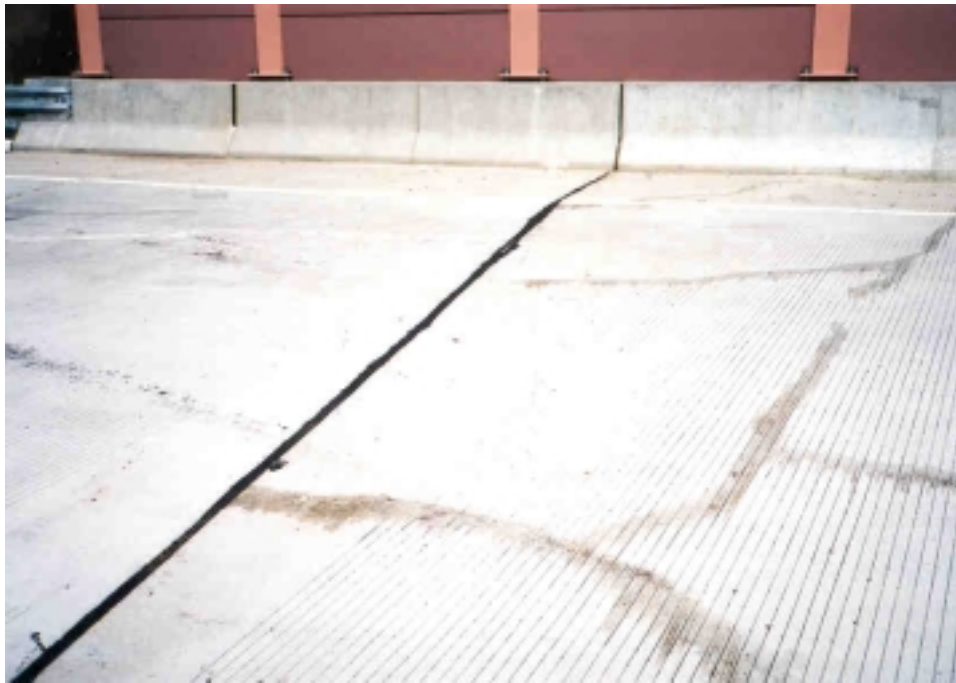
Figure 107. Transverse cracks on bridge deck (Bridge No. 1143-169).
