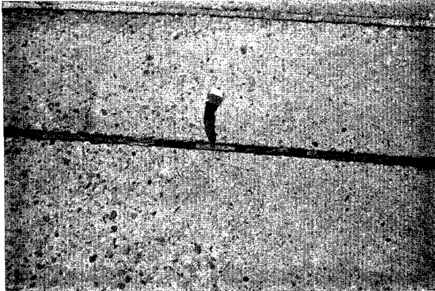
Figure 1. Typical anode grout distress.
