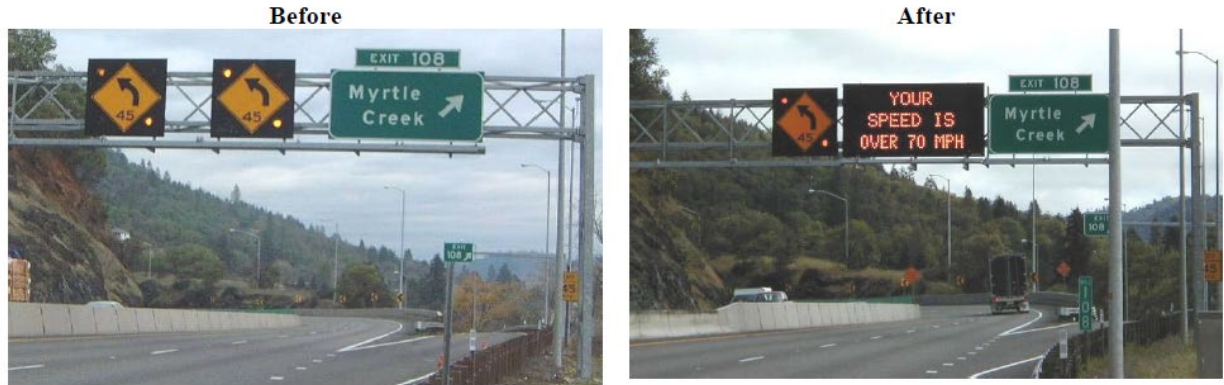
Figure 29. Curved section DSFS. (Before on left; after on right). (Bertini et al., 2006)
