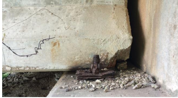
Figure 2.104. Bearing plate corrosion and spalling at the prestressed beam end
