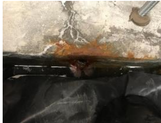
Figure 310. Visible confirmation of reinforcing bar corrosion during week 1
