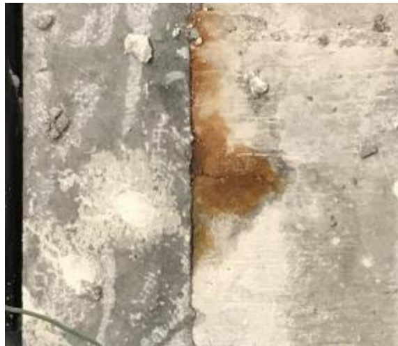
Figure 304. Joint corrosion in Ductal ® large-scale corrosion testing specimen during week 2 of testing (Ductal ® on left side of image)
