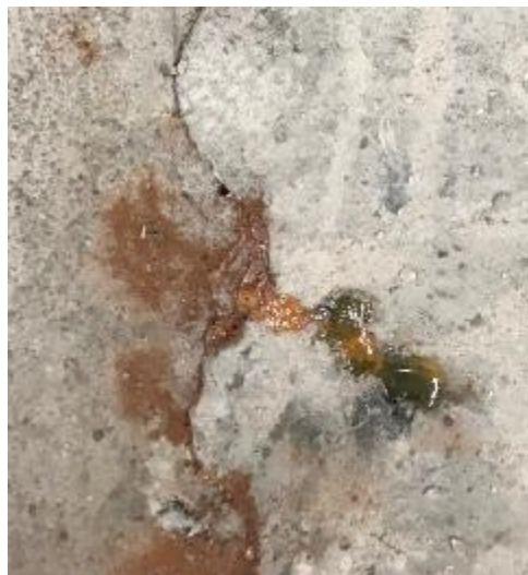
Figure 309. Green liquid in joint of Ductal® large-scale corrosion specimen during week 10 of testing
