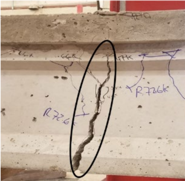
Figure 201. Flexural crack where the prestressing strands ruptured under the load point on the NC1-S girder, indicated by a dark oval
