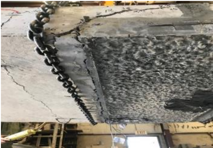
Figure 144. Cracks extending across the entire width of the slab at the joint and in the conventional concrete
