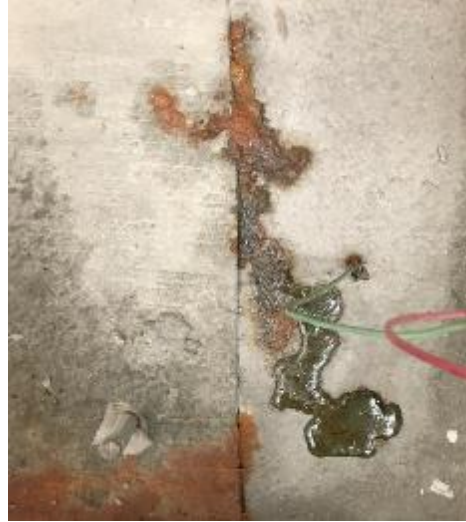
Figure 308. Green liquid in joint of Phoscrete large-scale corrosion specimen during week 10 of testing
