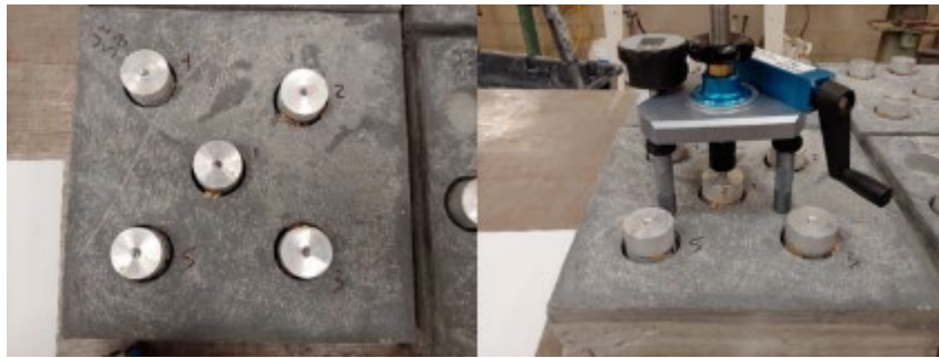
Figure 62. Pull-off tests for J3 with overall layout (left) and test setup (right)
