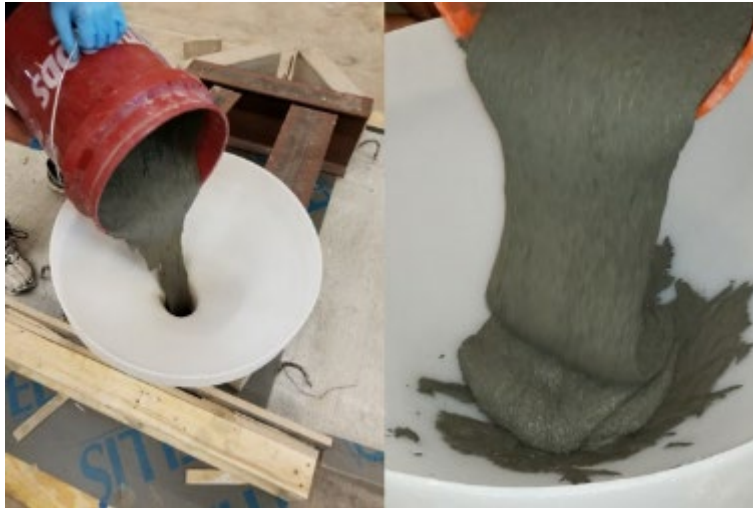
Figure 48. Placement of UHPC into the formwork for the first set of slab joints
