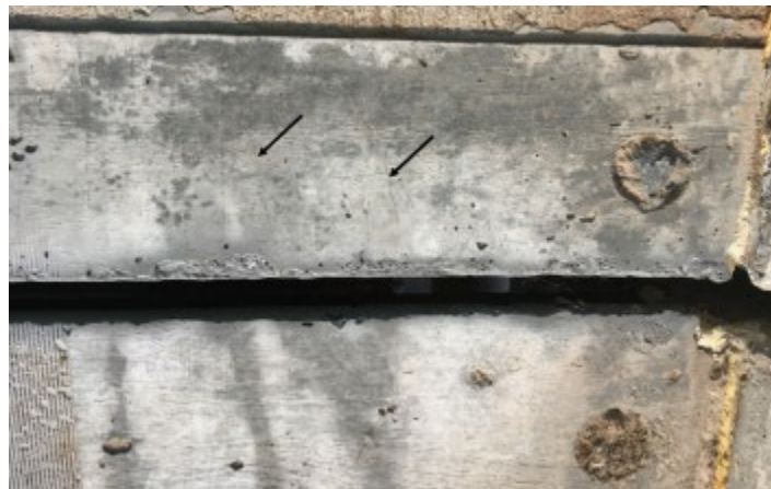
Figure 337. UHPC joint headers on SH-3E bridge before joint sealant was placed and showing hairline cracks
