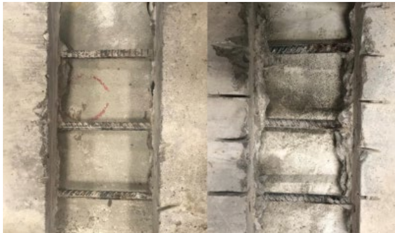
Figure 292. Corrosion state of rebar reinforcing at joint of ODOT Class AA small-scale corrosion specimens with 4% NaCl (left) and 8% NaCl (right)
