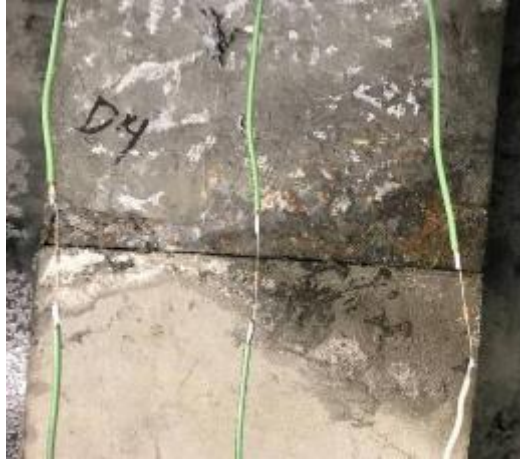
Figure 291. Initial joint corrosion in Ductal® small-scale corrosion testing specimen - corrosion spotting
