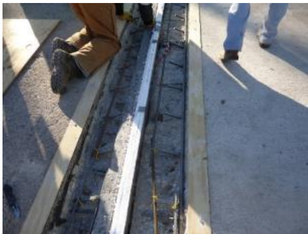
Figure 330. Joint after removal of existing concrete and before placement of the top form
