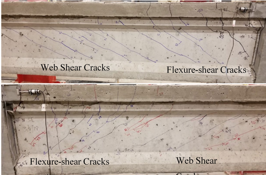
Figure 223. NC3-N girder with flexure-shear and shear cracks top and NC3-S girder with flexure-shear and shear cracks (bottom).
