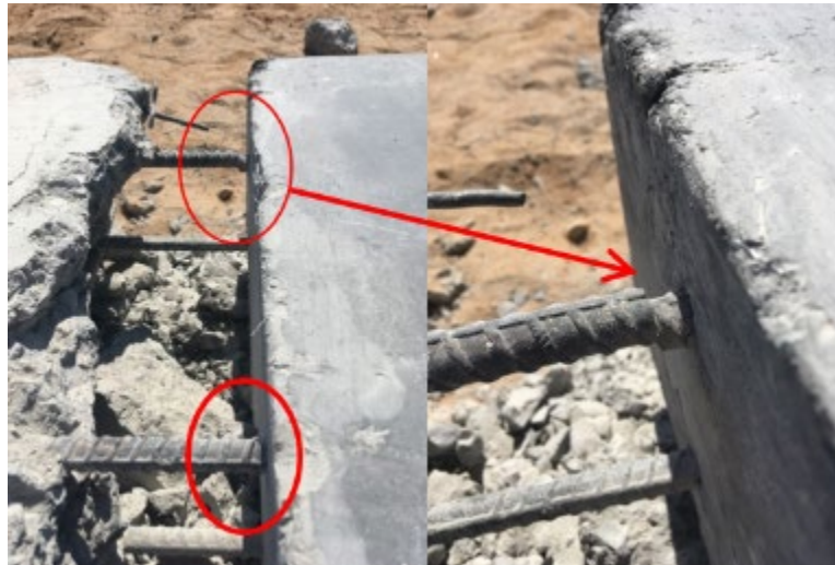
Figure 118. Fractured tension reinforcing bars after fatigue failure of slab joint (note that the slab has been flipped relative to the testing orientation)
