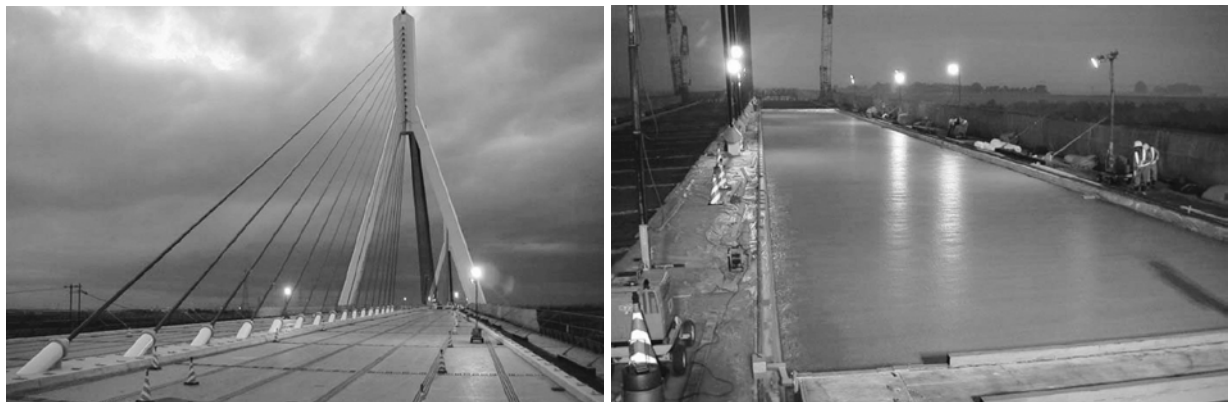
Figure 5-5 Construction of ECC Steel Composite Bridge Deck at Mihara Bridge in Hokkaido, Japan
