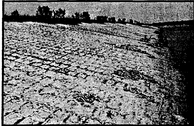
Figure 2.4 Soil Cement placed in the plating method parallel to the slope (PCA)
