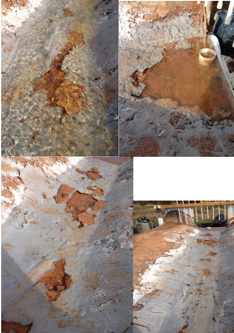
Figure 27. Failures, and resulting erosion, in the hydraulically applied concrete product after poor application to a test ditch.
