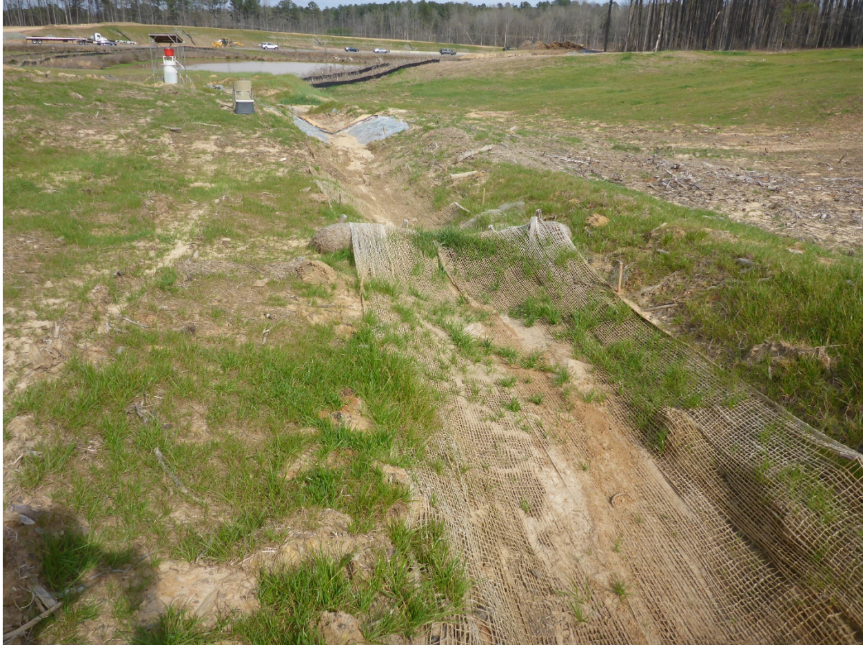
Figure 55. Vegetation establishment around the jute-lined ditch at the Durham location, at the time of the March 2 survey.
