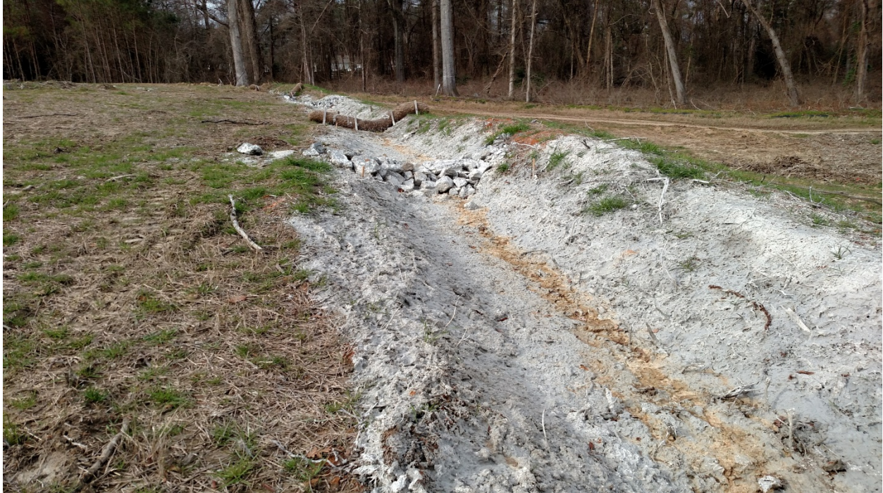
Figure 12. Diversion ditch lined with Posi-Shell after several flow events.
