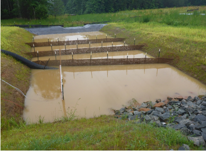
Figure 16. Sediment basin which has Posi-Shell applied to the two diversion ditches leading to its inlet.
