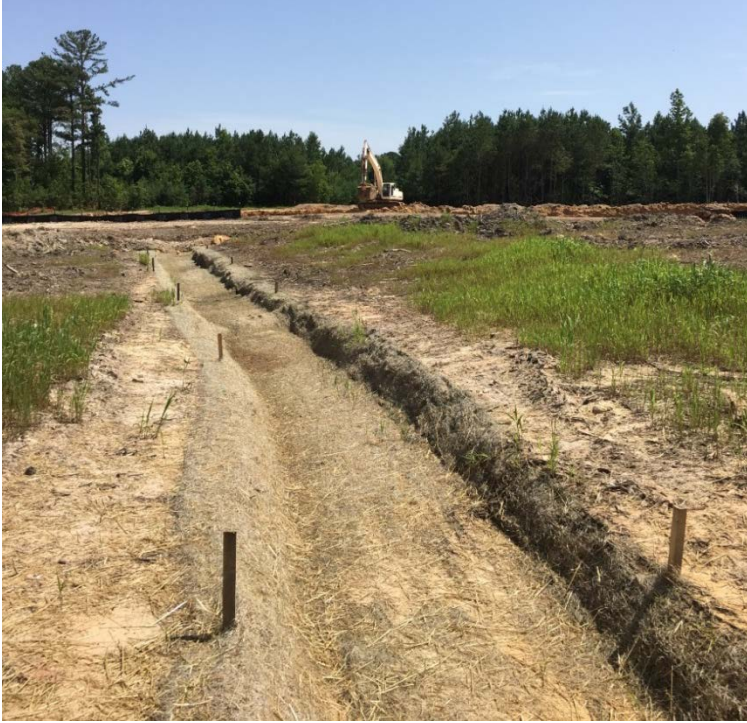
Figure 10. Excelsior-lined ditch at the Apex site after flow was cut off to it during grading. Stakes along each side are level across the ditch so the pin tool could be laid on them to measure changes in the cross-section.
