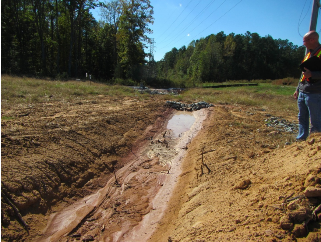
Figure 15. Unlined ditch in September 2017, showing no vegetation and eroding side walls.
