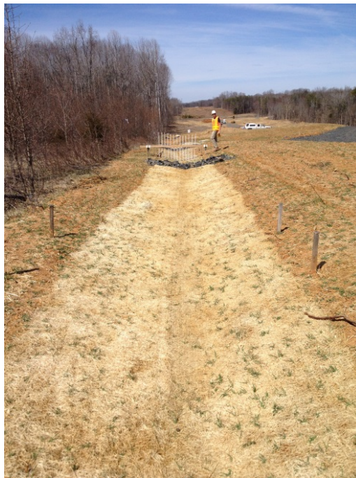
Figure 8. The rolled erosion control blanket (excelsior) treated section of Ditch 2 shows very few signs of erosion.
