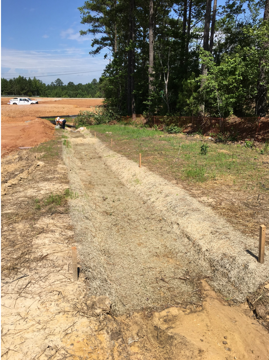
Figure 34. Excelsior-lined ditch in Apex showing the pin stations (stakes) and the V-notch weir at the outlet. Picture was taken July 6, 2016.
