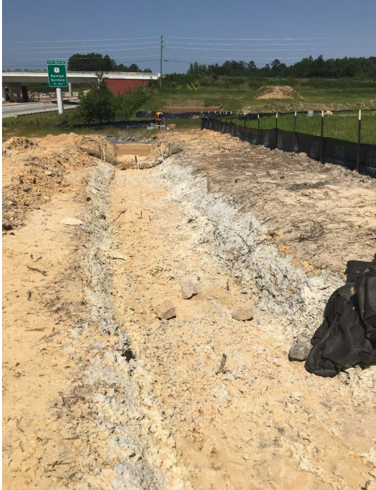
Figure 11. Posi-Shell-lined ditch at the Apex site showing erosion due to poor distribution of the material as a result of inadequate pressure in the hydroseeder.
