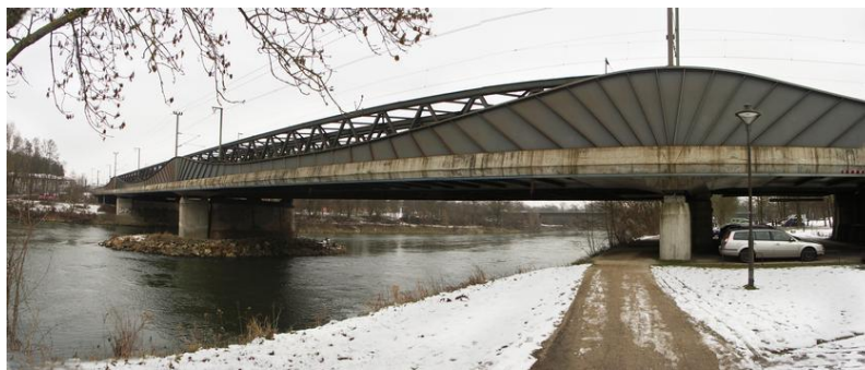
Figure 3.8. The Ingolstadt Rail Bridge, which is a composite trough bridge (Image credit: Janberg (Janberg 2020))
