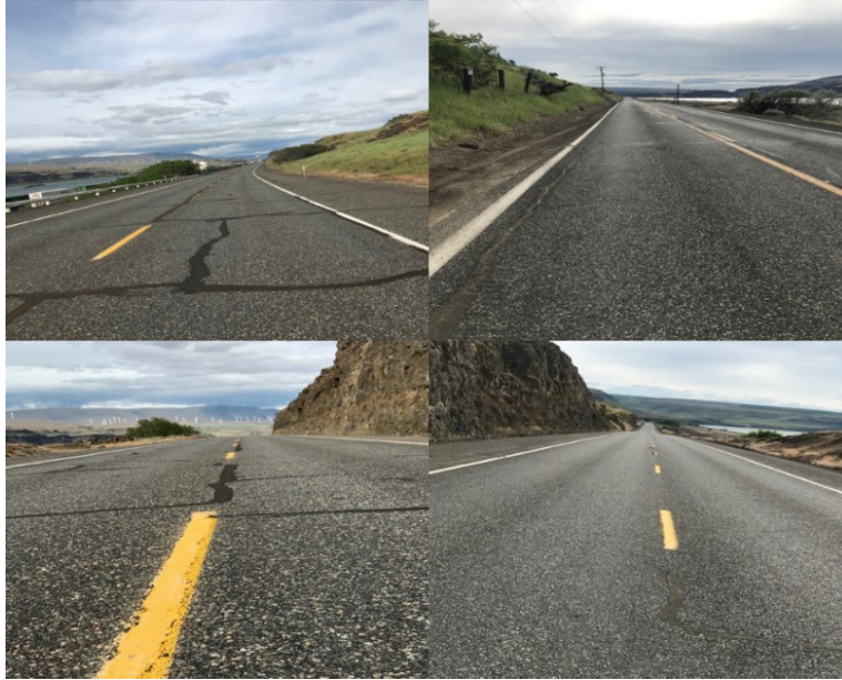
Figure 9.2. Road condition before chip sealing on Oregon 206
