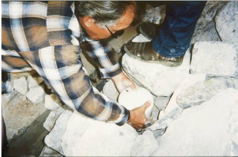
Figure 7.18. Installation of a float out device by Nevada DOT to monitor riprap stability.
