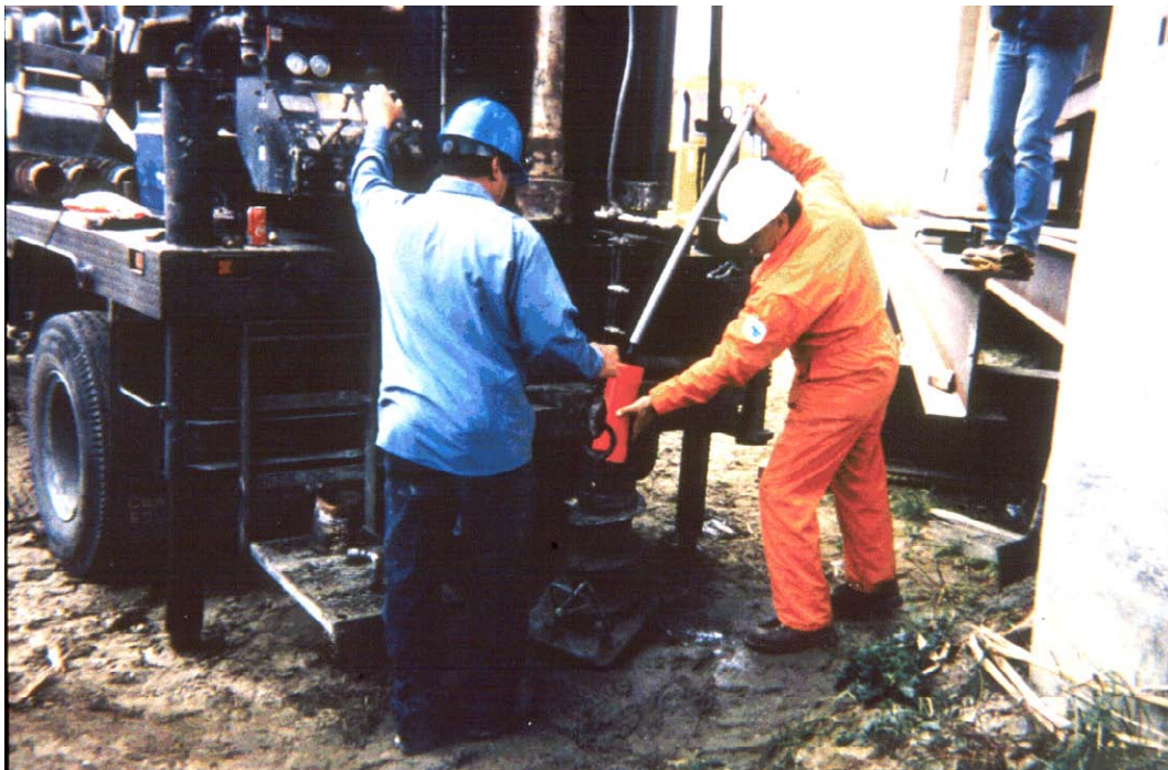
Figure 7.16. Installation of float out device on Salinas River bridge near Soledad, CA.
