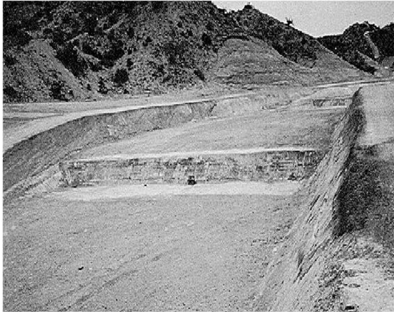
Figure 2.4. Soil cement bank protection and drop structures in Laughlin, NV. (7)
