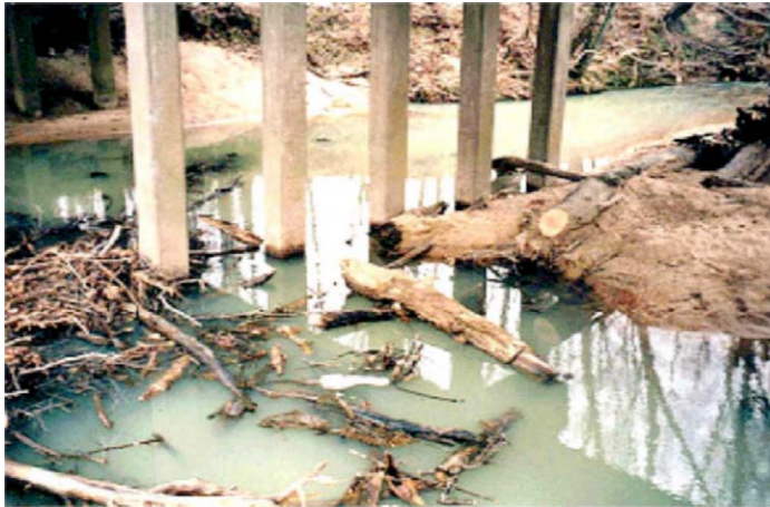
Figure 6.13a. Scour hole debris at Bridge 133, Graves County, KY
