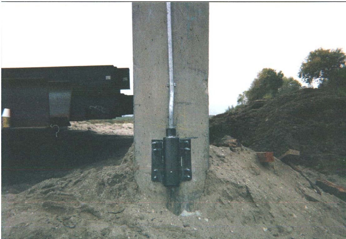
Figure 7.14. Close up of sonar scour monitor on Salinas River bridge near Soledad, CA.
