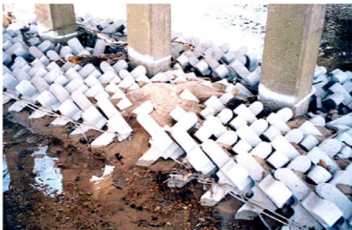
Figure 6.13c. Close-up of armor units after several flow events at Bridge 133, Graves County, KY
