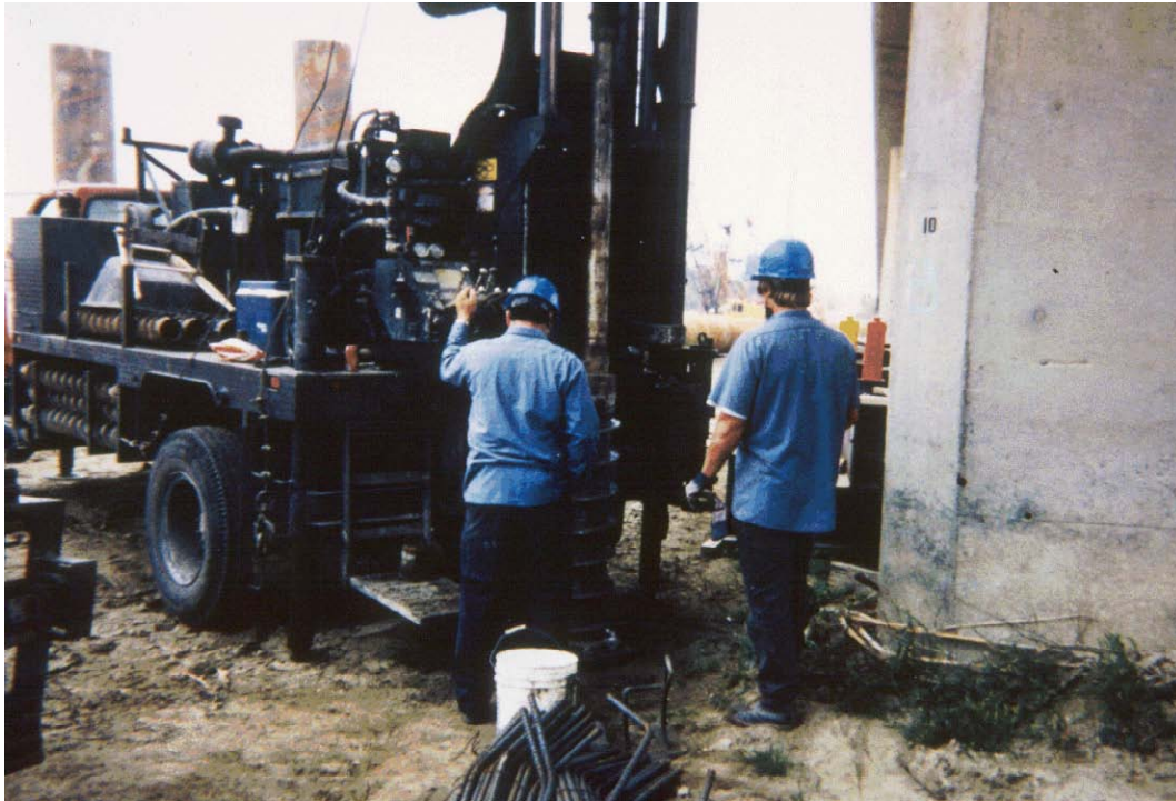
Figure 7.15. CALTRANS drilling with hollow stem auger for installation of float out devices at Salinas River bridge (Highway 101) near Soledad, CA.
