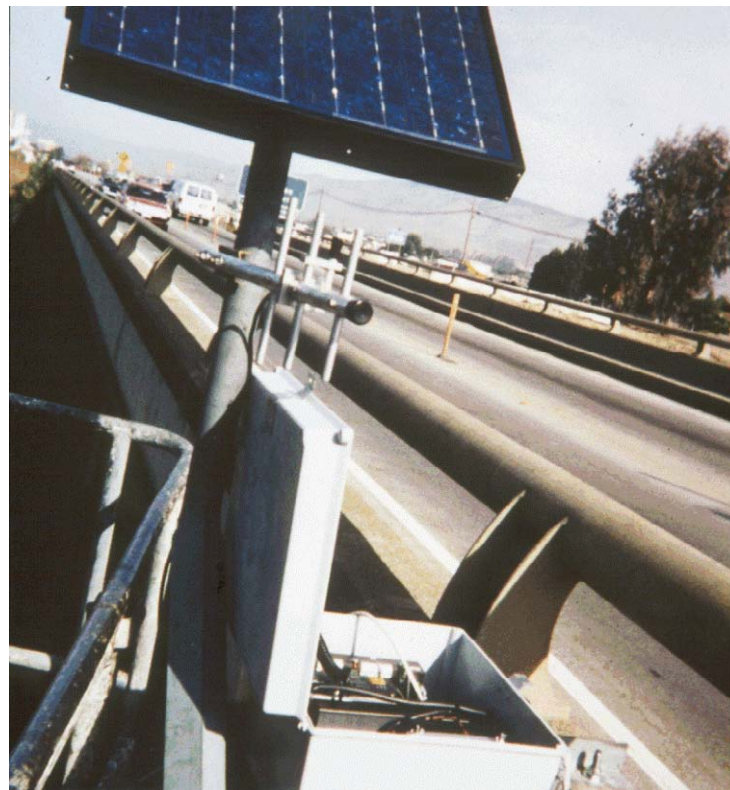
Figure 7.17. Typical instrument shelter with data logger, cell-phone telemetry, and a solar panel/gel-cell for power.
