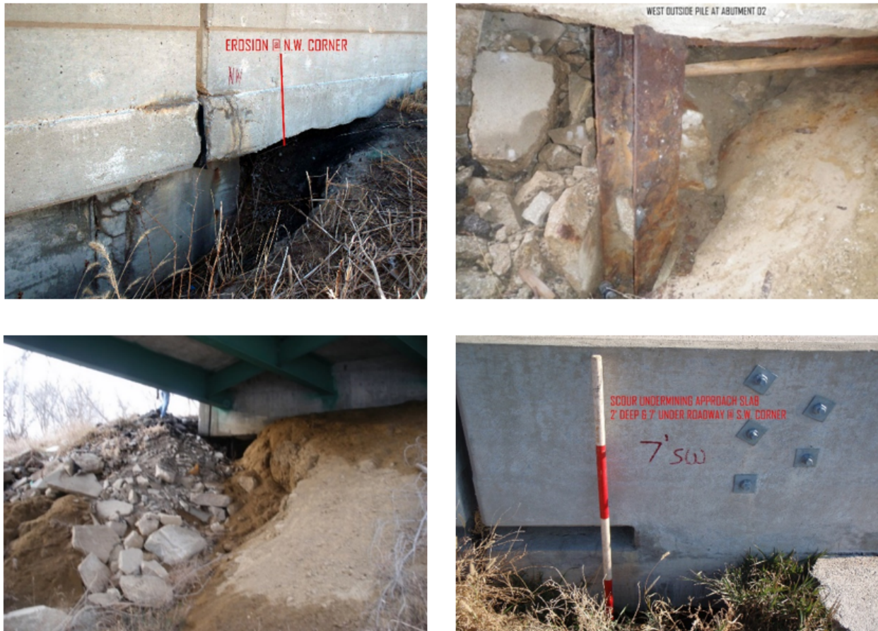
Figure 2.11 An example of soil erosion problems observed at some of the surveyed bridges in Nebraska that were built with the current design policy.
