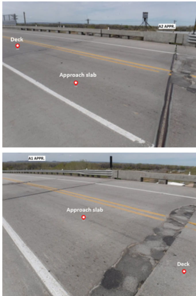
Figure 2.9 An example of minor problems encountered in the approach slab with the new design in Nebraska.
