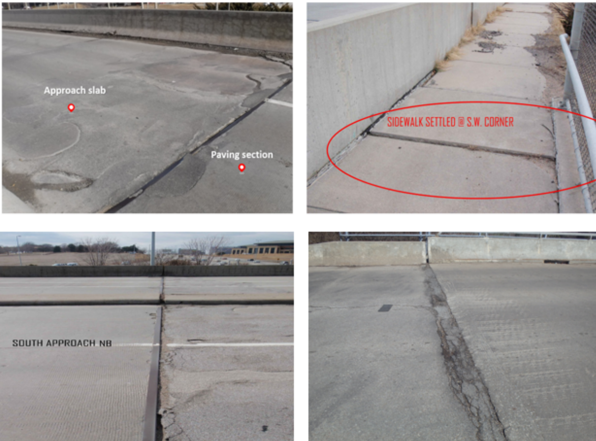
Figure 2.2 An example of the bump problems encountered near the end of approach slab of bridges built with the old design in Nebraska.
