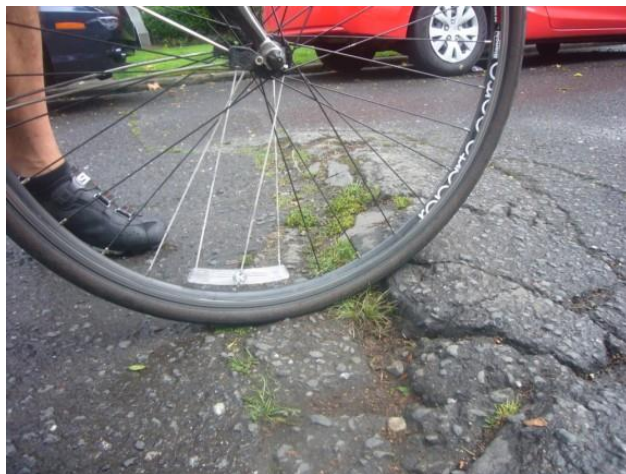
Figure 3.9: Pavement Condition (source: Seattle Bike Blog)
