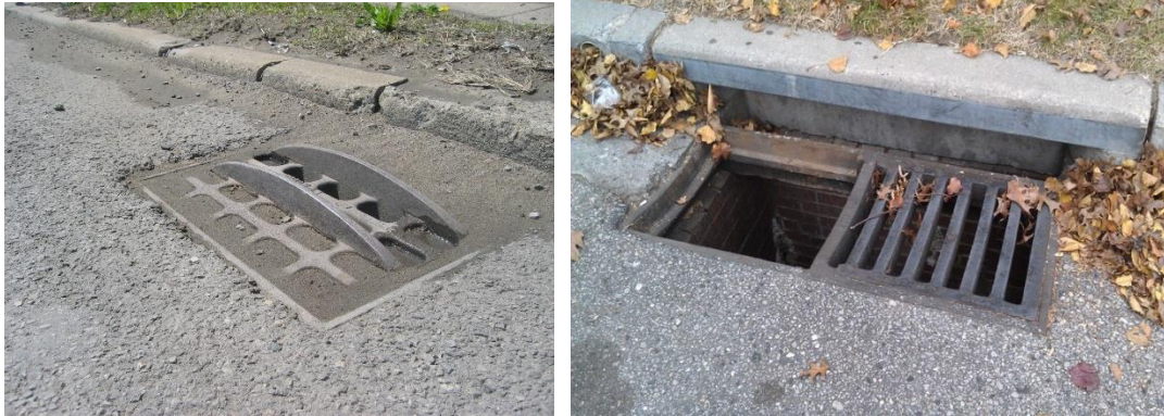
Sewer Grate Road Hazard (source: m-bike.org ) Uncovered Storm Drain (source: SeeClickFix )
