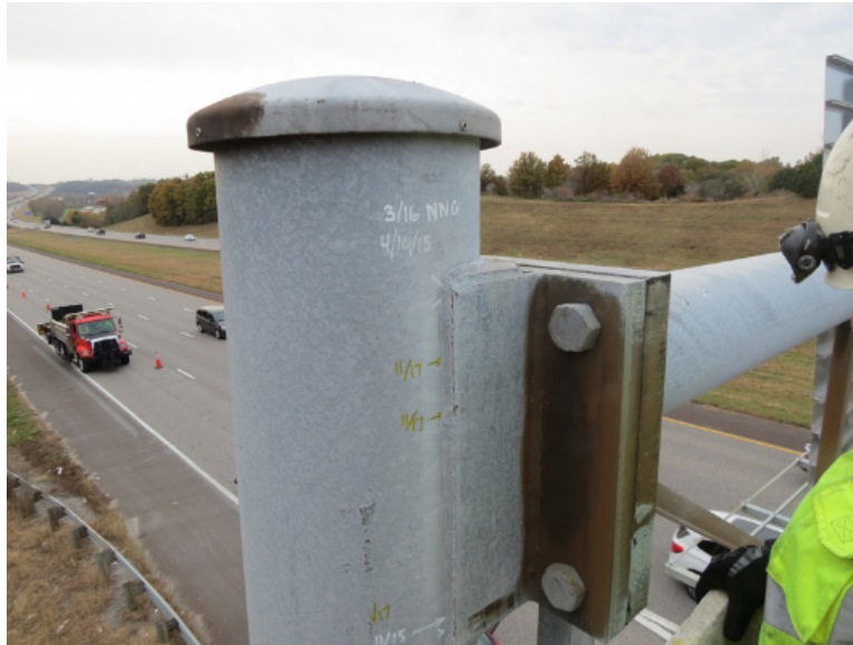
Figure 1.2: Typical crack monitoring at the box connection of a two-chord COSS
