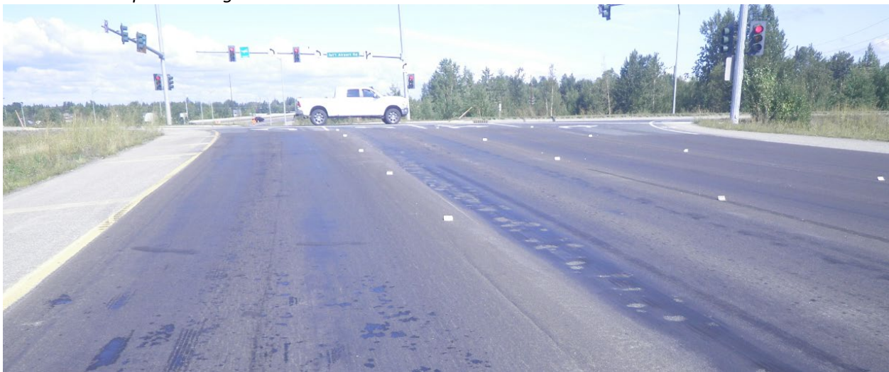
Photo 16 - Ramp 2 Flushing Distress
