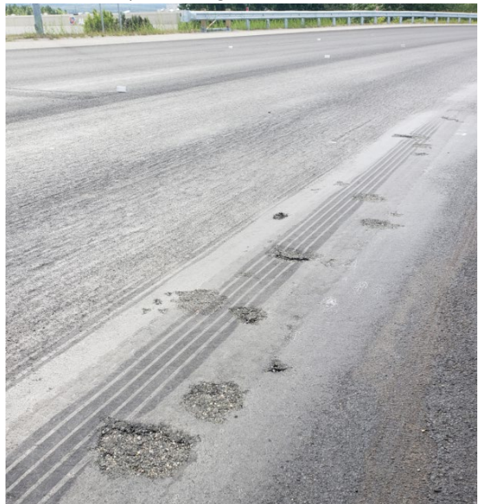
Photo 15 - Ramp 2 Flushing Distress
