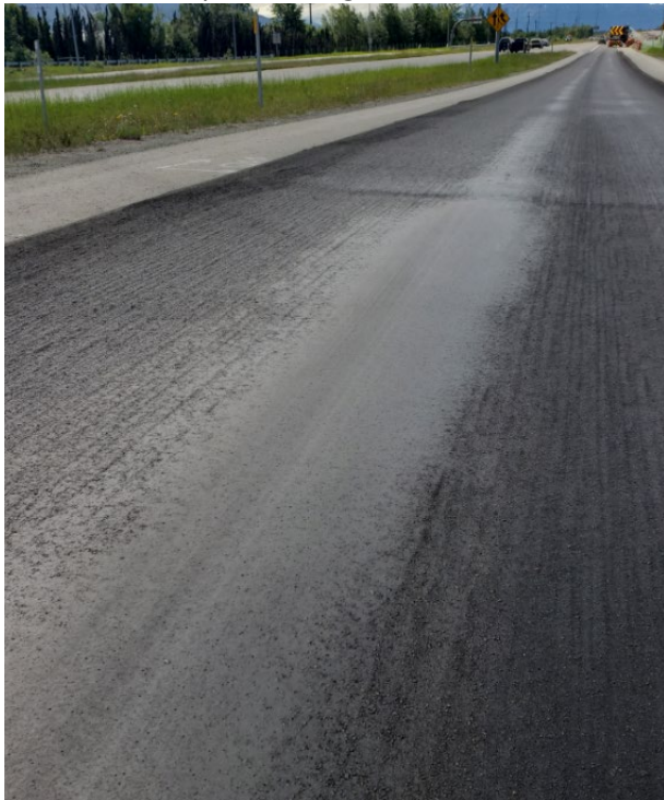
Photo 14 - Ramp 1 Flushing Distress
