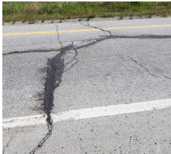
Photo 6 - Ramp 12 - Cracks after Surface Preparation
