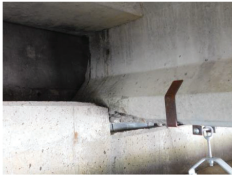
(a) Bottom Flange Deterioration
