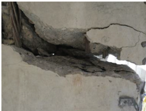
Figure 5.11 Fractured prestressing strands in bottom flange after testing.
