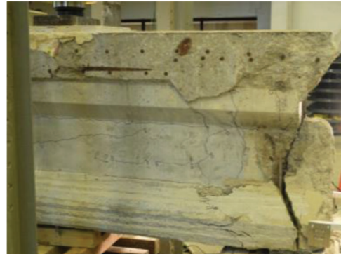
Figure 5.15 NSM FRP specimen after failure.
