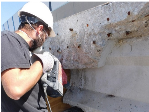
(a) Removing Delaminated Concrete
