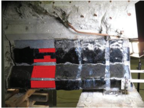
Figure 5.10 Externally bonded FRP specimen after failure.
