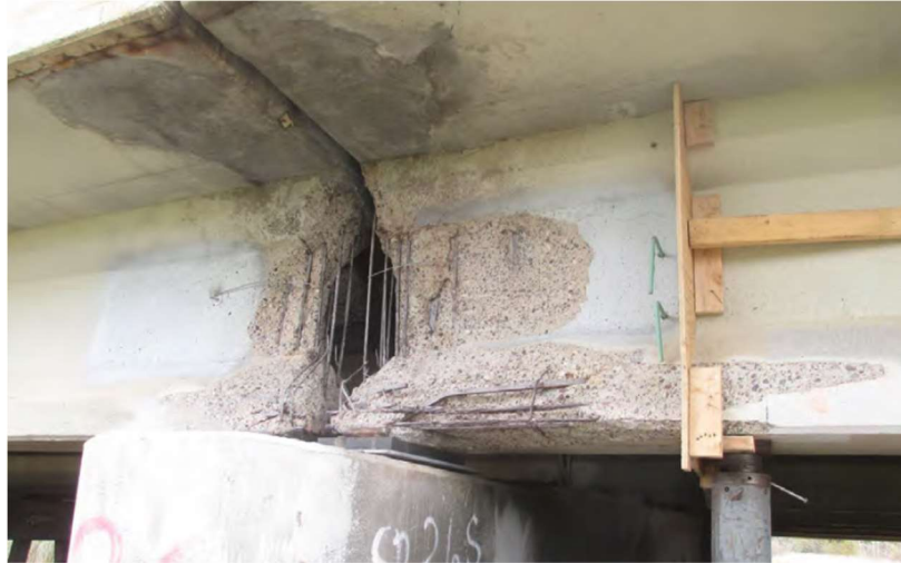
(a) Condition of the Girder Following Removal of Delaminated Concrete
