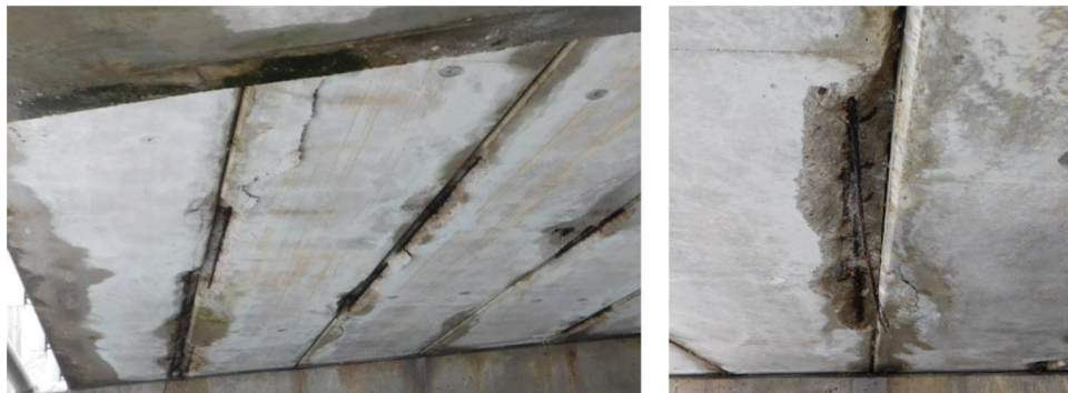
Figure 1.2 Common deterioration patterns (Elkhart, Indiana, Bridge No. 102 CR 35 over Little Elkhart River).
