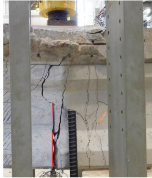
Figure 5.12 Critical flexural crack of externally bonded FRP specimen after failure.
