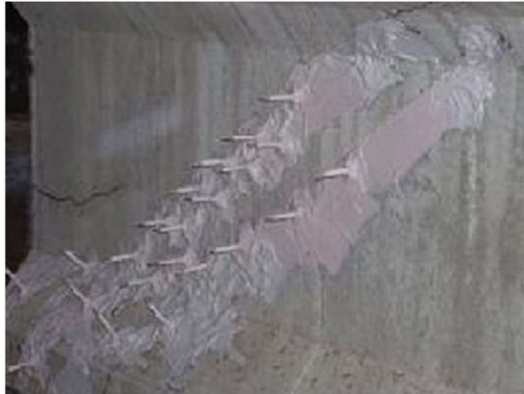
(c) Epoxy-Injected Cracks
