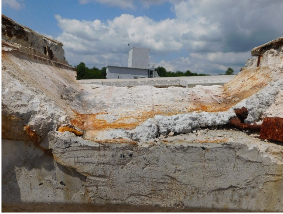
(a) Void Left After Drain Removal
