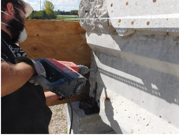
(a) Removing Delaminated Concrete
