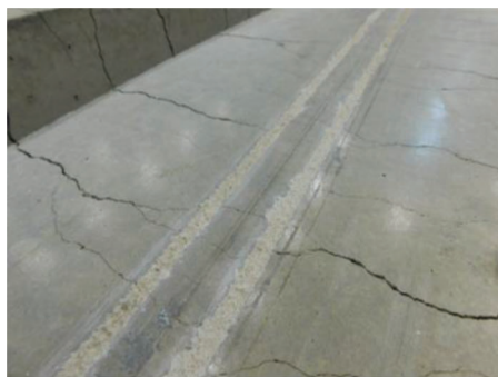
(a) After Failure
