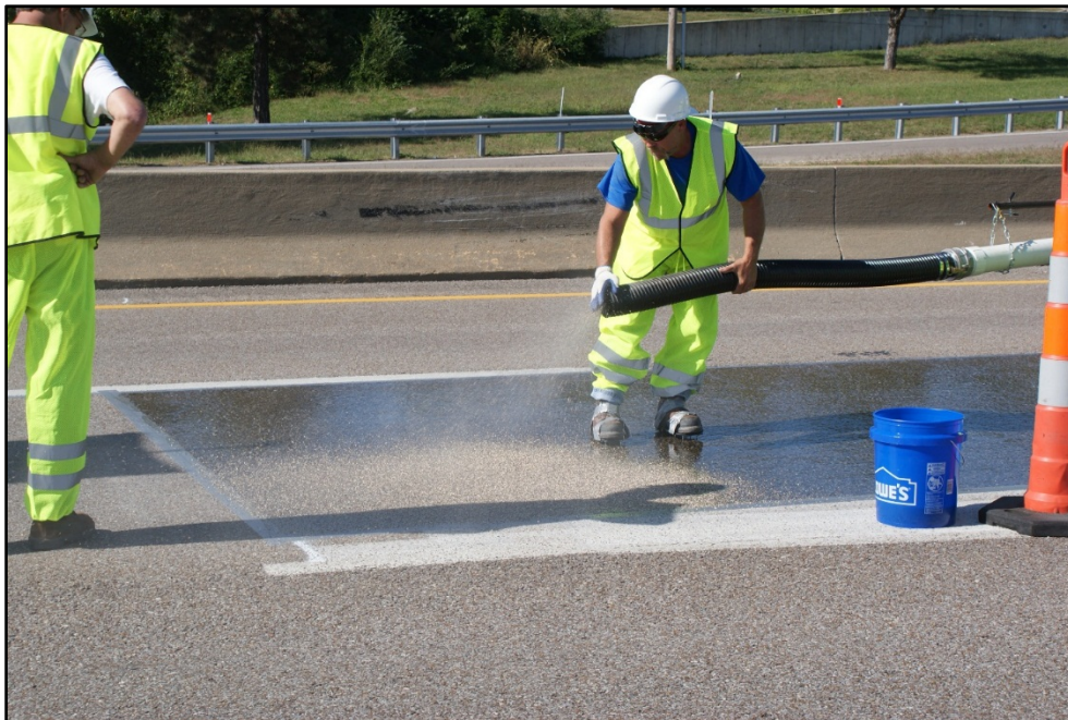
Figure 2.4. Example of blower used to place aggregate onto fresh epoxy for HFST surface.
