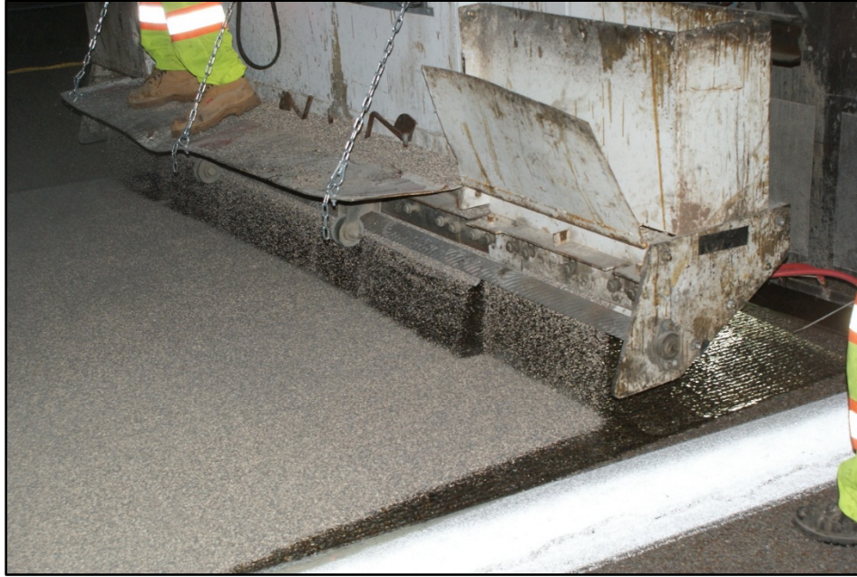
Figure 2.3. Example of machine used to place aggregate onto fresh epoxy for HFST surface.
