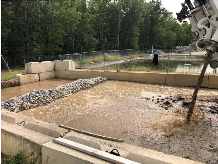
Figure 5. A Typical Dewatering Pad Used to Drain Material Collected During Storm Drain and Pipe Clean-Outs
