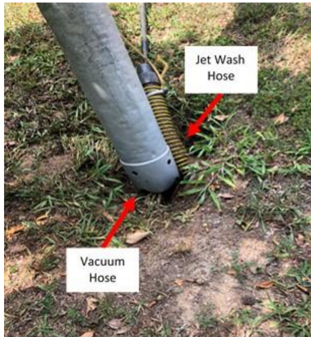
Figure 4. Clean-out of the Driveway Pipe Shown in Figure 3. Here the jet wash hose is used to loosen and flush out material although the vacuum hose collects it.
