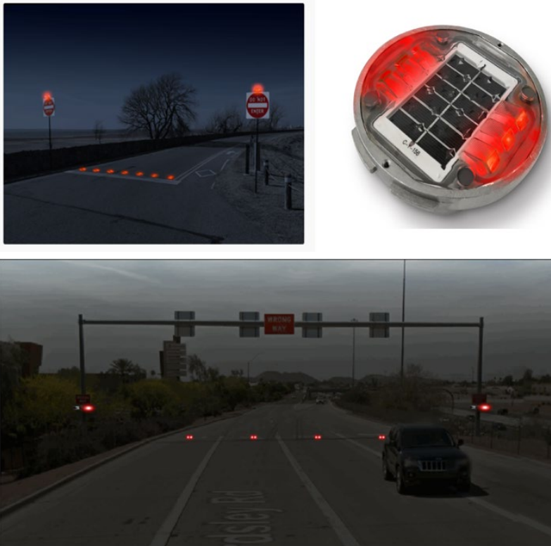
Figure 2-2 In-Pavement Flashing Light Examples
