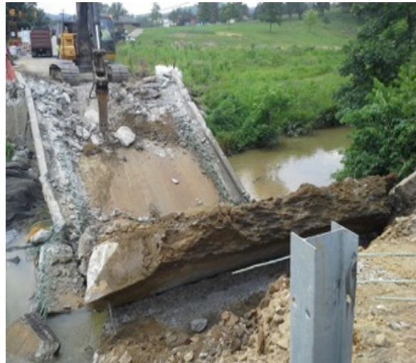
Figure 1. Demolition of a bridge in Pennsylvania. The state has the highest number of structurally deficient bridges. [PennDOT 2009]
