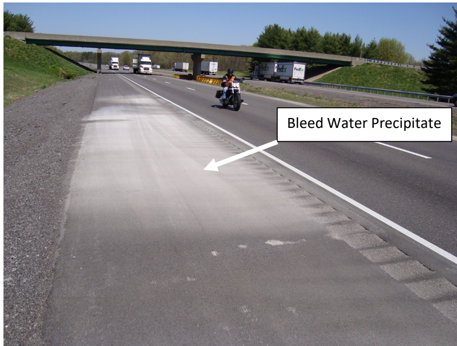
Figure 8. Photo. Bleed water precipitate—April 2010.
