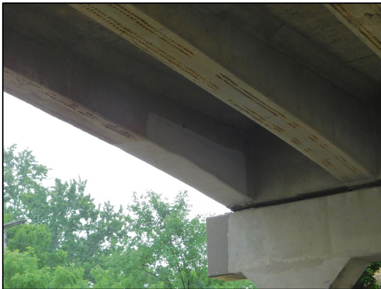
Figure B.34 Close-up of FRP-repaired beam end at western end pier.
