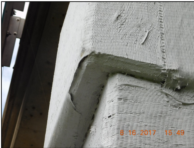
Figure B.137 Poor detailing at pier cap-to-column intersection.
