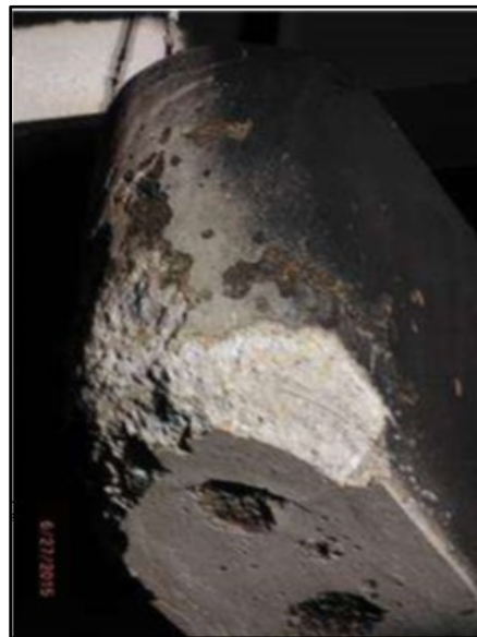
Figure B.124 Scaling of the north end of bent cap (from Mickler (2015a) inspection report).
