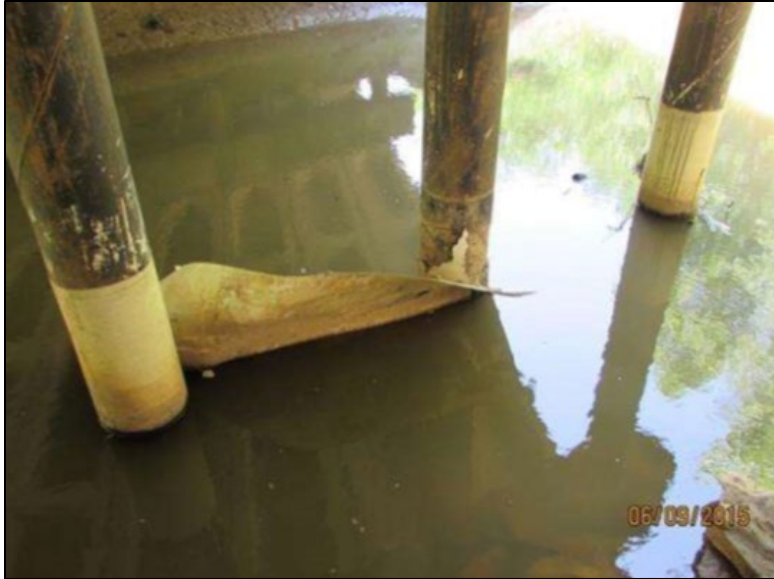
Figure B.149 Column wrap damage at eastern pier (from Olson (2015) inspection report).
