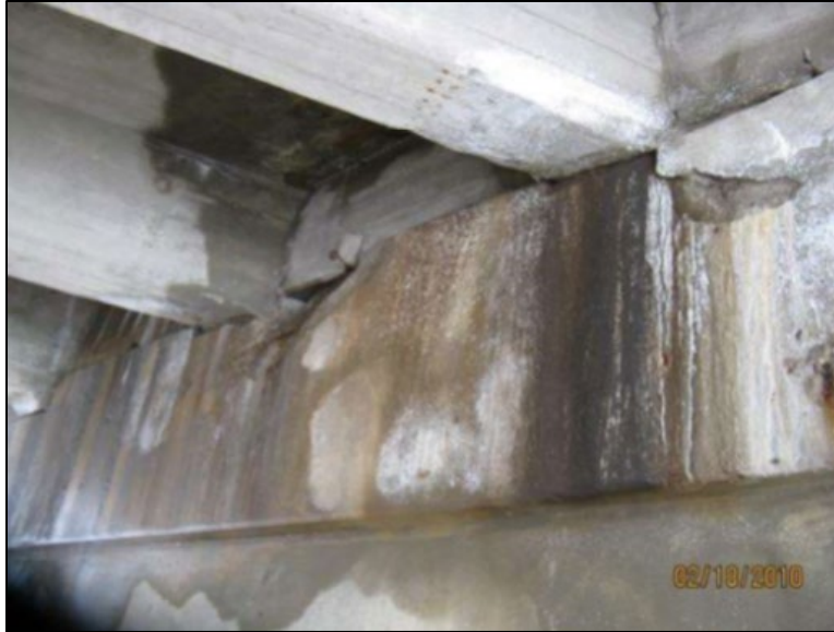
Figure B.79 Wet pier at leaking joint in eastbound bridge (from Smith (2010a) inspection report).
