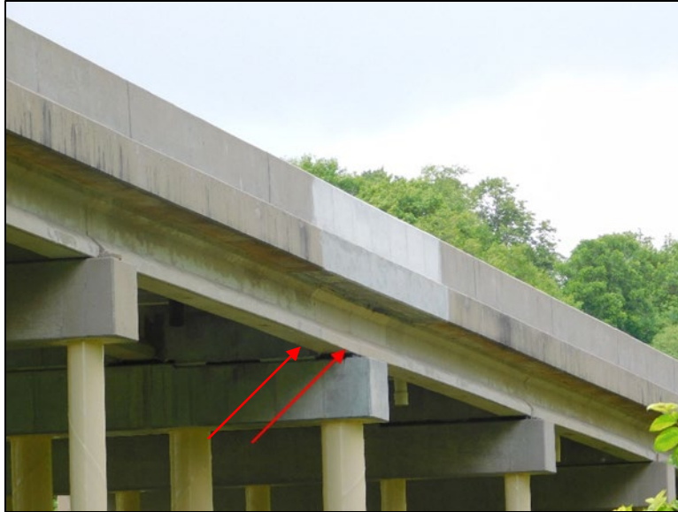
Figure B.58 Beam end repair at Pier 7 at expansion joint (from the southeast).
