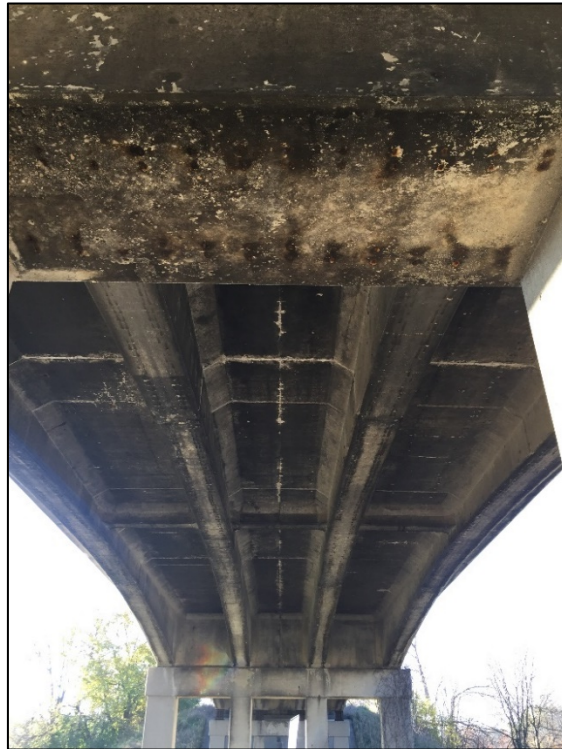
Figure B.139 Fire-damaged northern spans.
