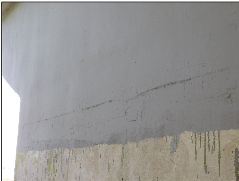
Figure B.43 Paint/epoxy runoff on sheets and onto concrete.
