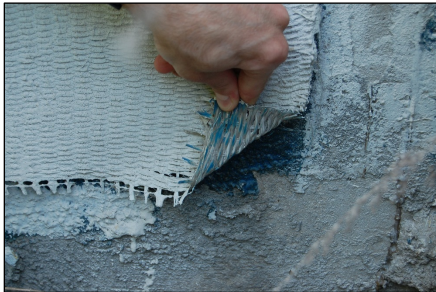
Figure B.23 Debonding at easternmost column of Bent 5.
