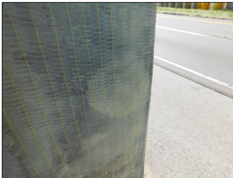
Figure B.171 Possible void or excess epoxy in repair region.
