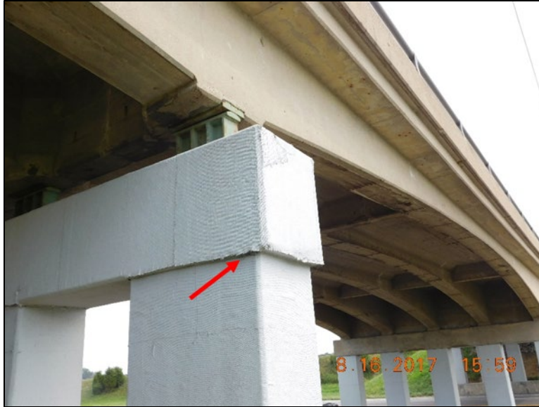
Figure B.136 Poor detailing at pier cap-to-column intersection.
