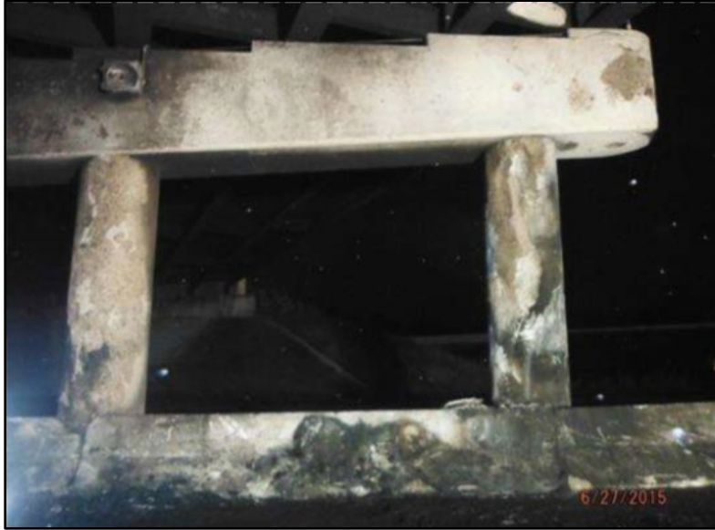
Figure B.123 Fire damage to Bent 2 (from Mickler (2015a) inspection report).
