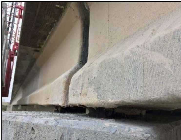
Figure B.64 Fiber wrapped beam ends at Pier 4 (from Schamberger (2016b) inspection report).
