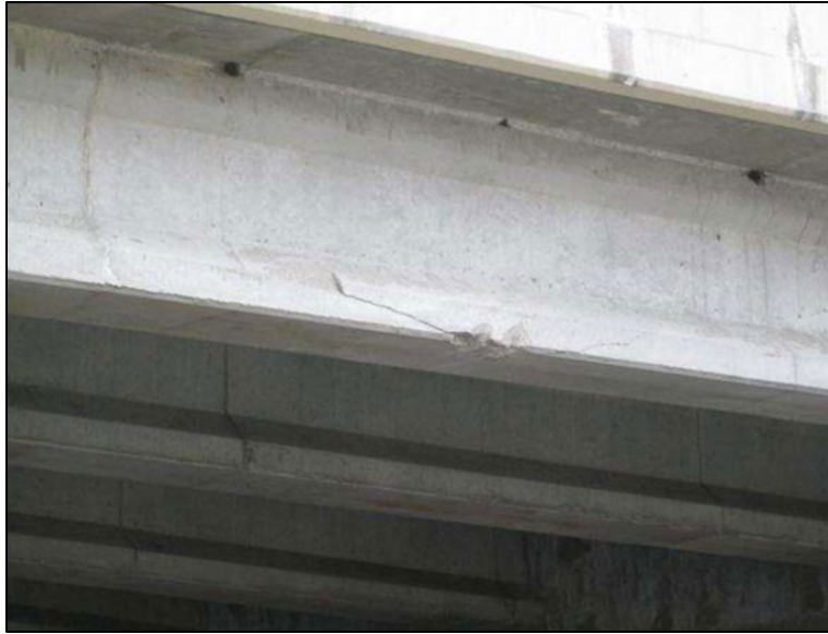
Figure B.103 Impact-damaged girder prior to FRP Repair (from Post (2013) inspection report).
