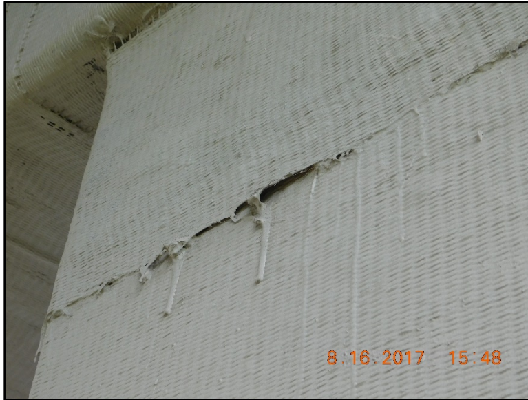
Figure B.134 Local debonding of column wrap.
