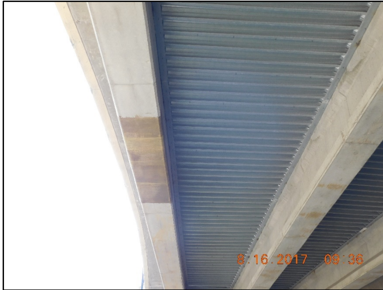
Figure B.106 Impacted fascia girder and undamaged adjacent girder.
