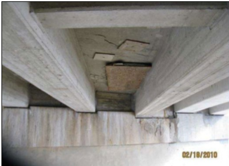
Figure B.80 Patching of deck underside of eastbound bridge (from Smith (2010a) inspection report).
