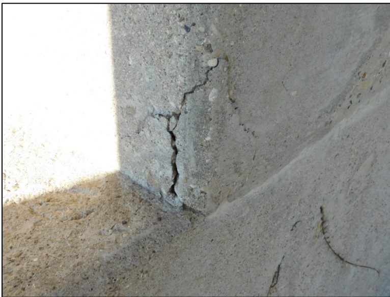
Figure B.175 Spalling of Pier 3.
