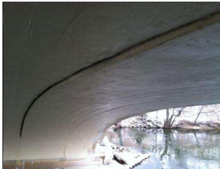
Figure B.8 Arch separation (from Dittrich et al. (2013) inspection report).
