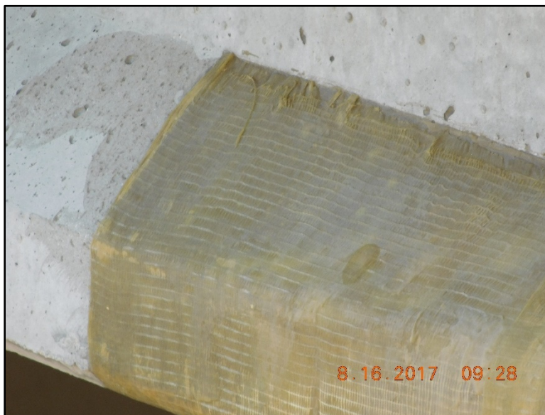
Figure B.105 Minor frayed edges at termination along web.
