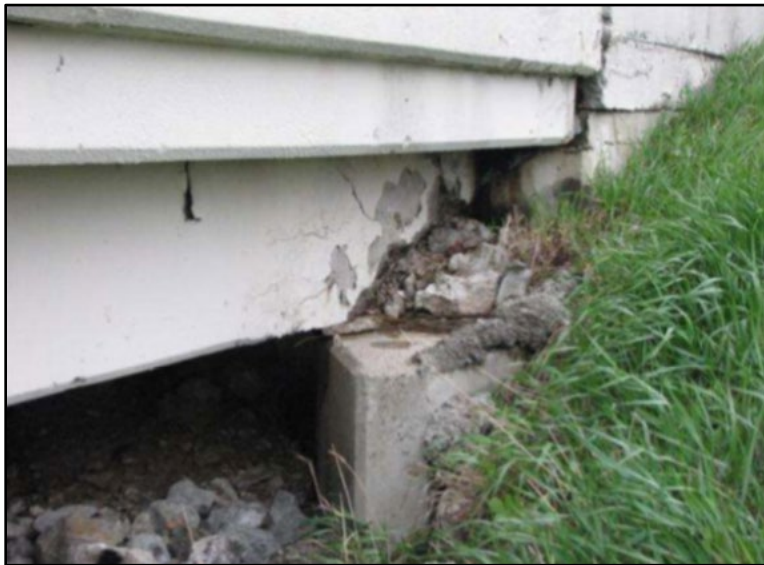
Figure B.90 Crumbling west girder at southwest corner of southern abutment (from Bewley (2011a) inspection report).
