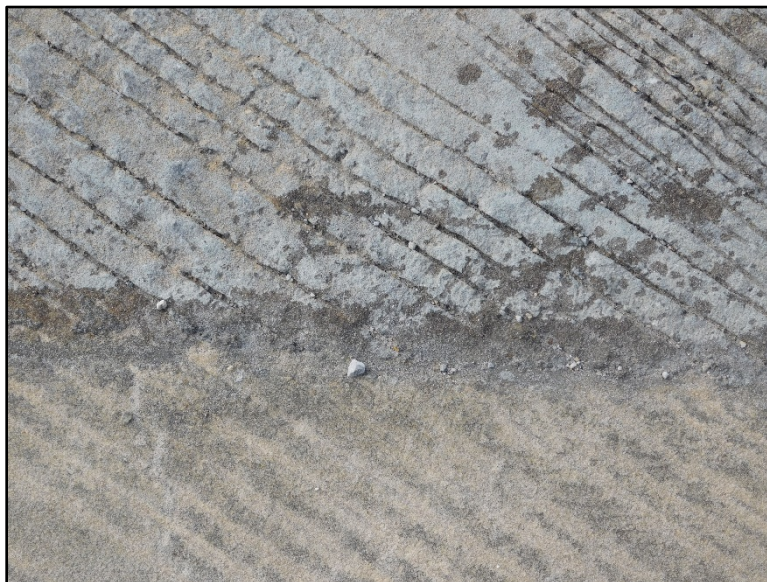
Figure B.66 Sand Layer on top of deck above the abutment diaphragm.
