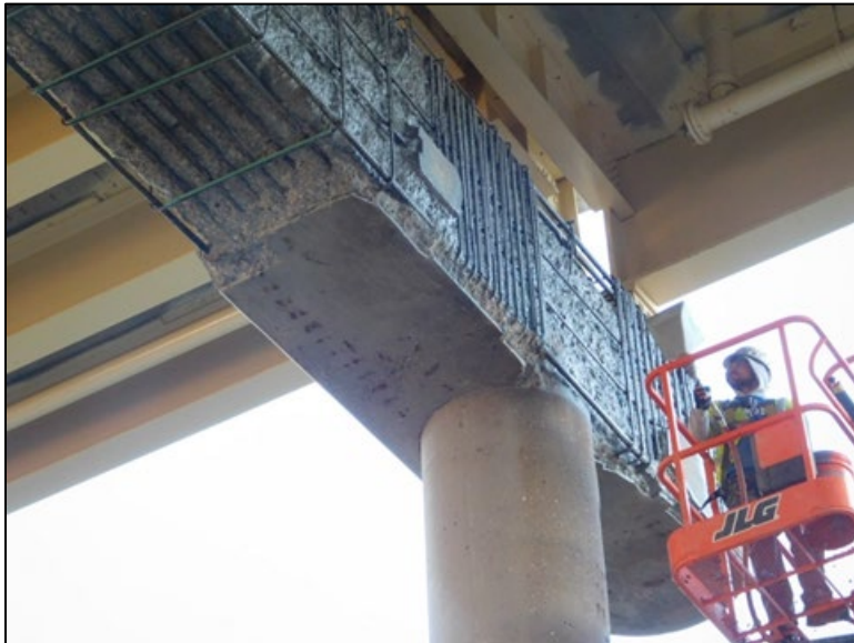
Figure B.182 Cleaned steel and removed concrete substrate prior to shotcrete application.
