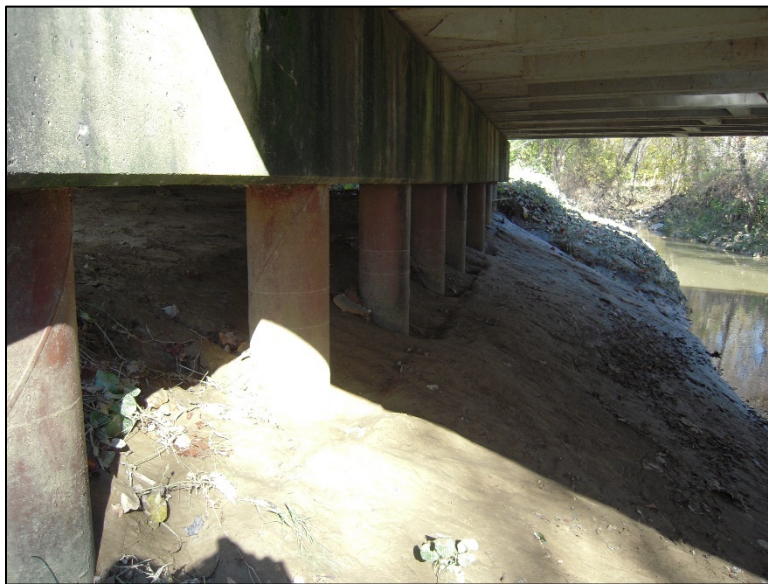
Figure B.153 Unwrapped columns at western pier.
