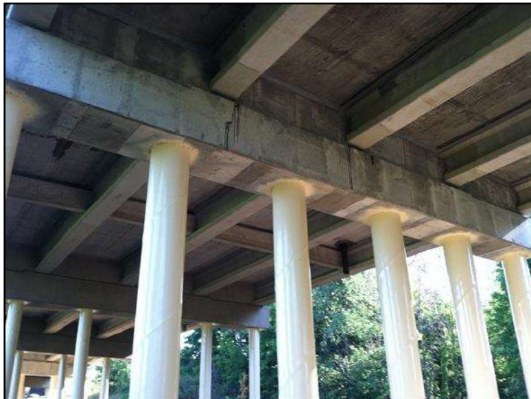
Figure B.52 Repaired beam ends, new bent cap, and encased piles at Bent 4 (from Biller & Gimbel (2014) inspection report).
