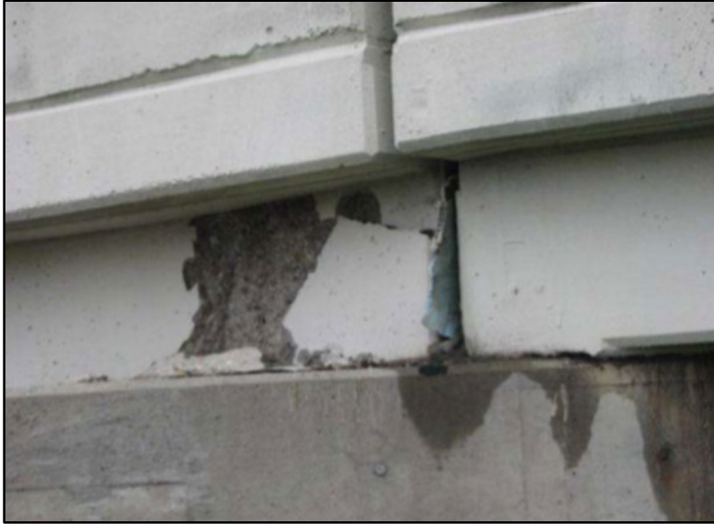
Figure B.89 Spalled east girder with exposed steel above Pier 2 (from Bewley (2011a) inspection report).
