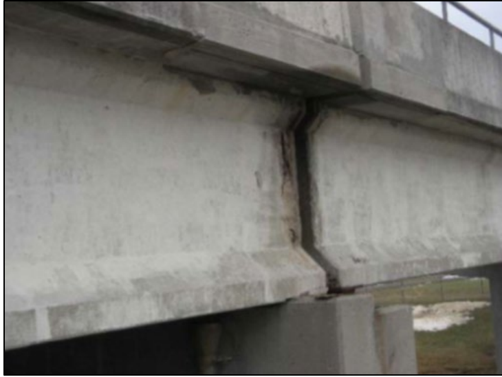
Figure B.157 Beam end deterioration at Pier 28 (from Everman (2010) inspection report).
