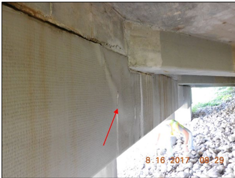
Figure B.100 Large void and discoloration on wrapping at Pier 4.
