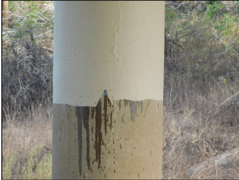
Figure B.74 Epoxy runoff and sheet bubbling.
