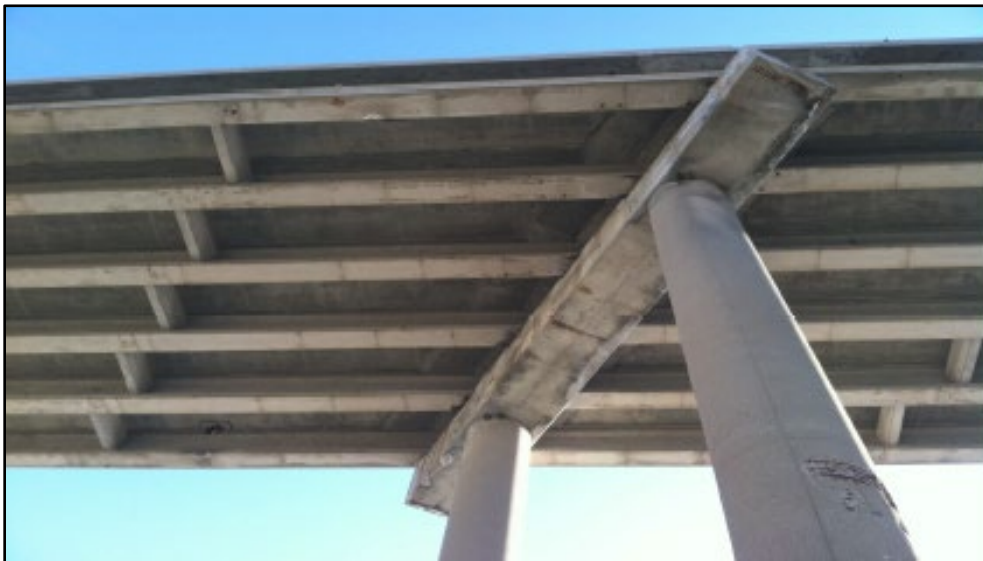
Figure B.62 Column spalling and cap deterioration at northbound Pier 4 (from Biller (2014a) inspection report).
