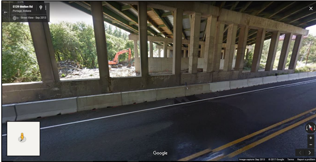
Figure B.20 Spalling and steel exposure of Bent 4 prior to FRP installation, September 2013 (Google, 2013).
