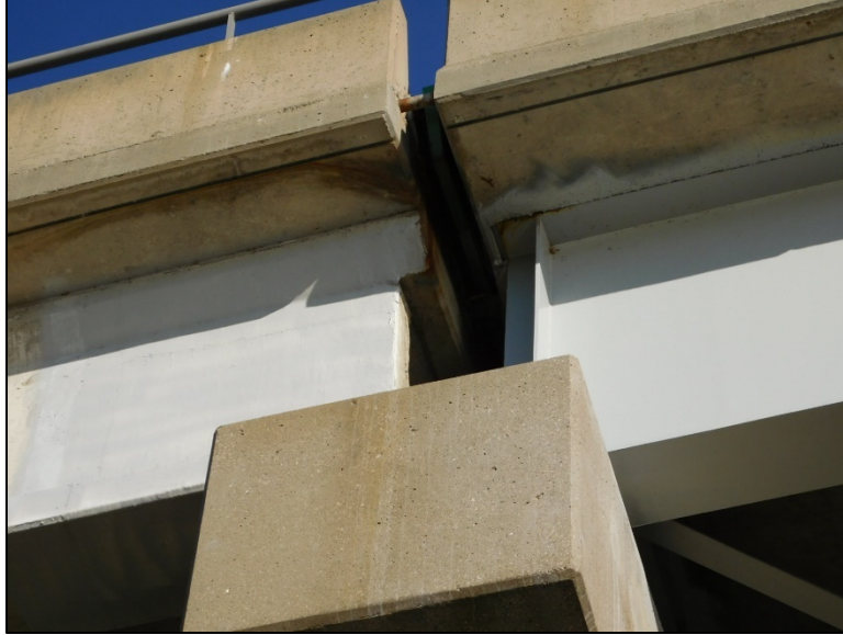
Figure B.167 Beam end repairs at Markland Dam joint.
