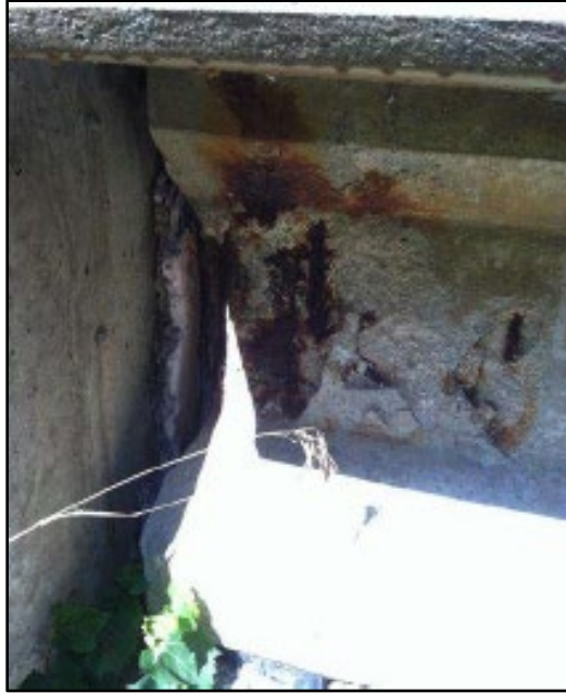
Figure B.49 Deterioration at Beam 5 in Span A (from Biller (2013) inspection report).
