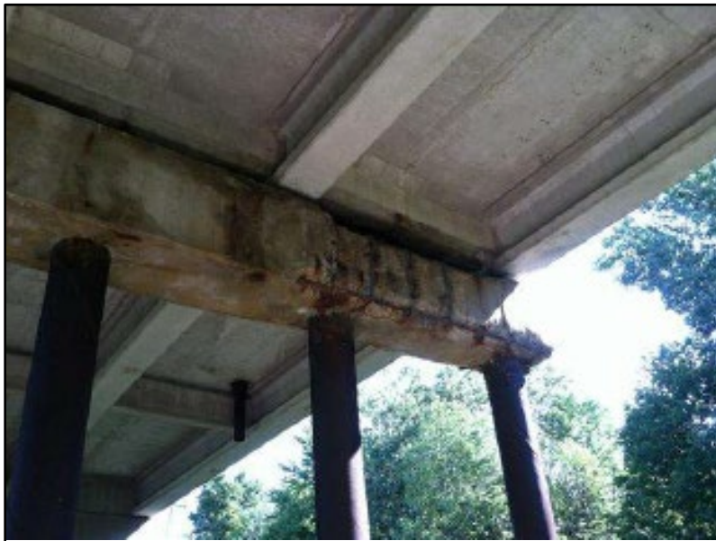
Figure B.50 Deterioration at Pier 4 bent cap (from Biller (2013) inspection report).
