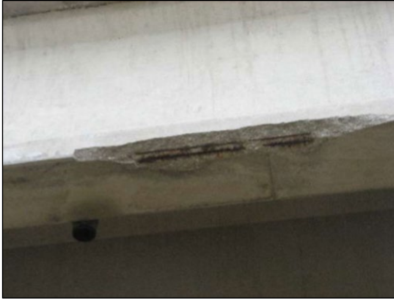
Figure B.159 Midspan spalling and exposed steel (from Everman (2010) inspection report).
