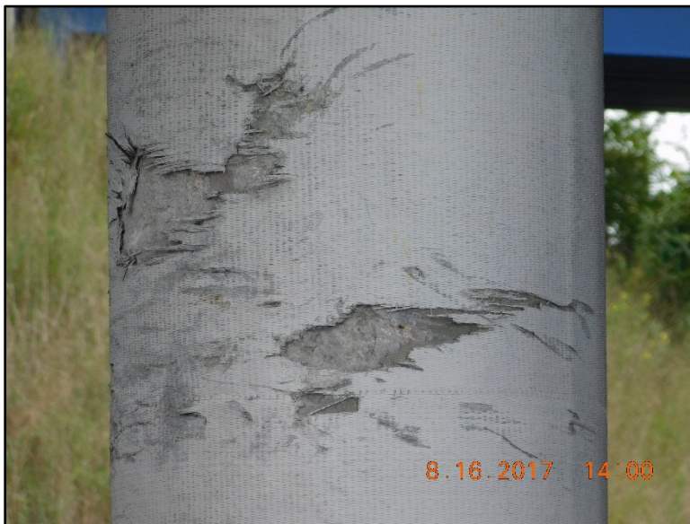
Figure B.126 Damage to northernmost column with exposed concrete.
