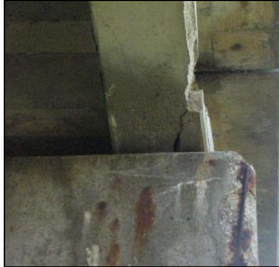
Figure B.47 Spalling of fascia beam and deep crack (from Atkinson (2011) inspection report).
