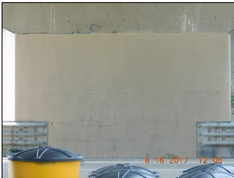
Figure B.121 Inconsistent layers and sagging of sheets.
