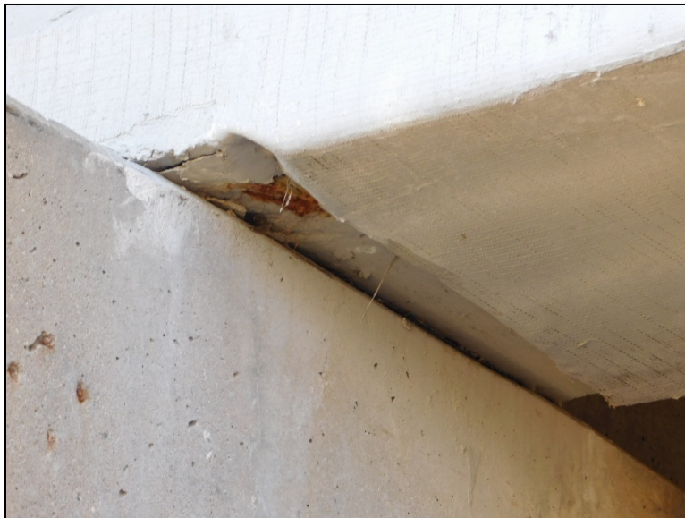
Figure B.164 Premature termination of FRP wrap at support location.
