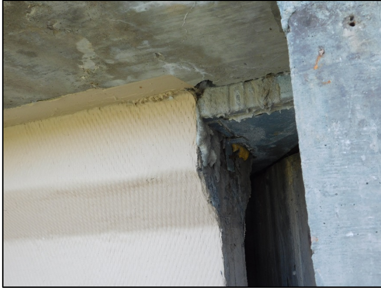
Figure B.70 Sheet termination at bottom of deck.
