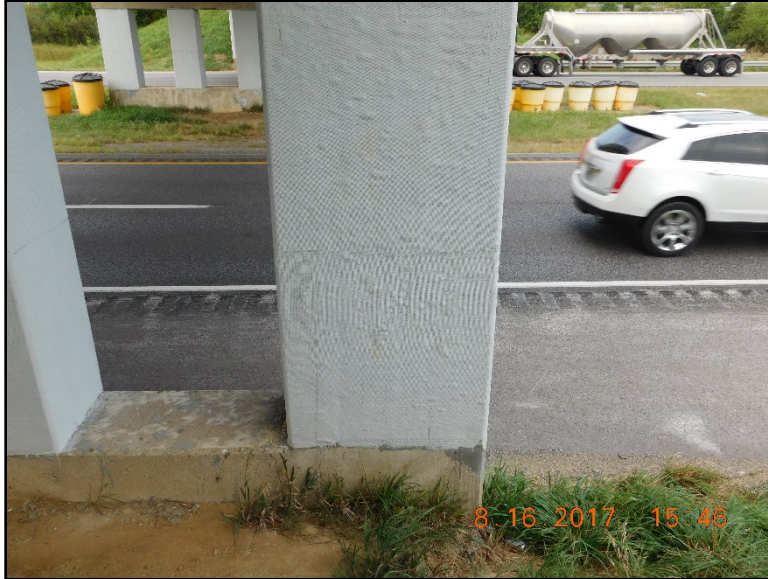
Figure B.132 Multiple voids in column wrap.
