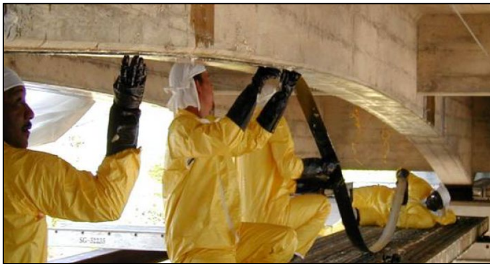
Figure B.4 FRP application to Uphapee Creek Bridge Girder (from Carmichael & Barnes, 2005).
