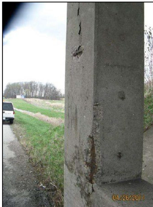
Figure B.29 Spalling and delamination at Pier 4, Span C (from Smith (2011) inspection report).
