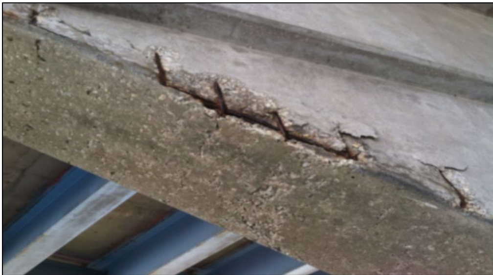
Figure B.39 Pier 2 north hammerhead spalling and exposed steel (from Biller (2015a) inspection report).
