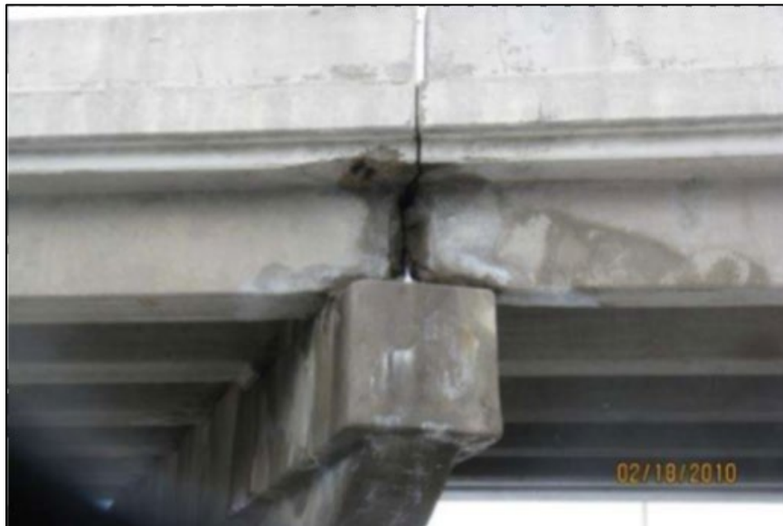
Figure B.78 Beam end deterioration at eastbound bridge (from Smith (2010a) inspection report).
