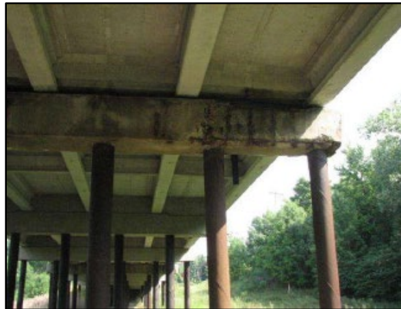
Figure B.46 Deterioration at Pier 4 (from Atkinson (2011) inspection report).
