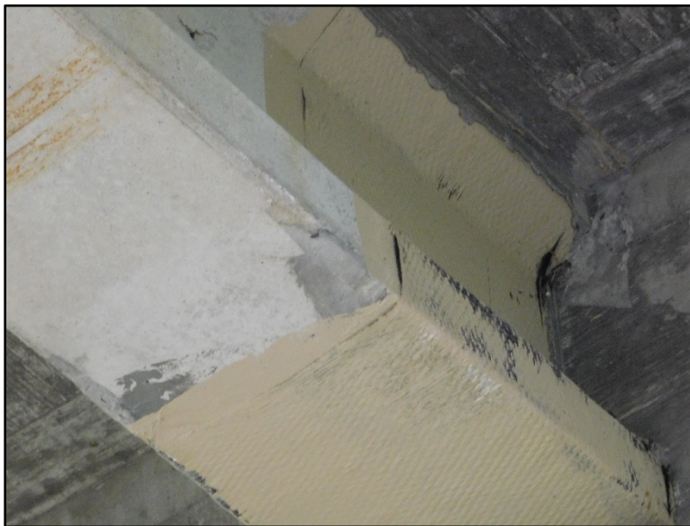
Figure B.59 Local debonding at beam ends at Pier 7.
