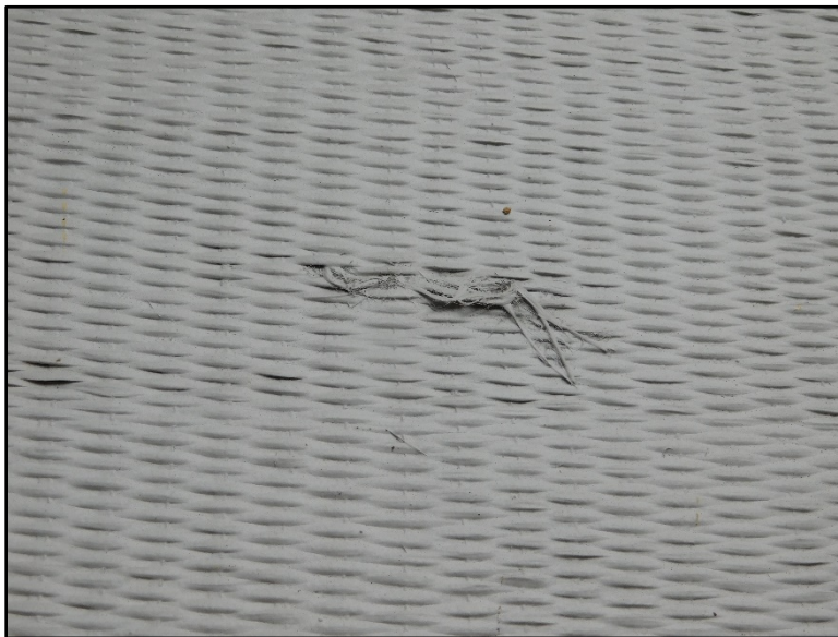
Figure B.85 Damaged and hanging fibers.
