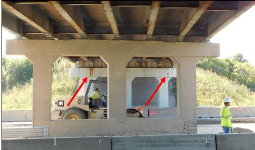
Figure B.113 Rust staining and other discoloration at southeastern pier.
