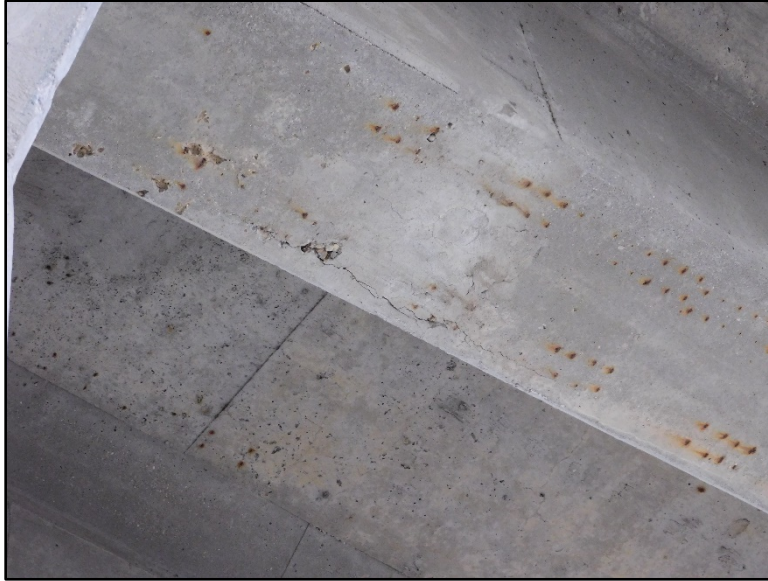
Figure B.37 Cracking along middle beam.
