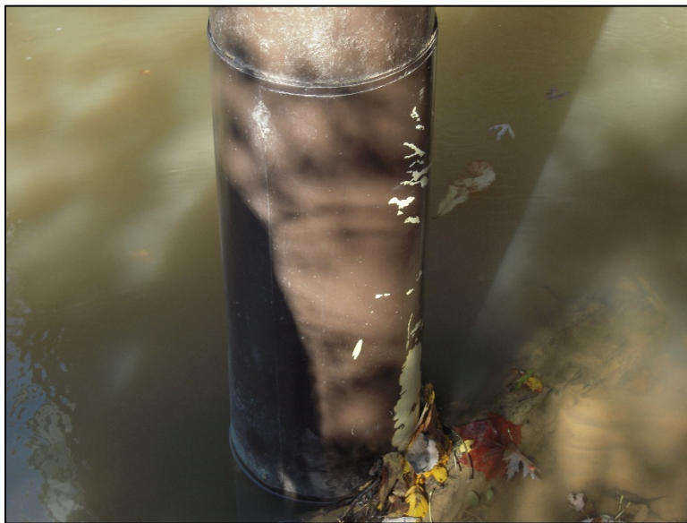
Figure B.151 Paint chipping on column wrap.
