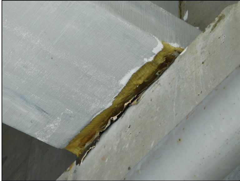
Figure B.165 Cracking/splitting of sheet at support location.
