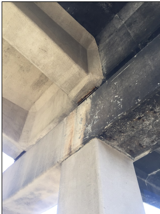
Figure B.143 FRP Repairs to column and portions of pier cap and superstructure.
