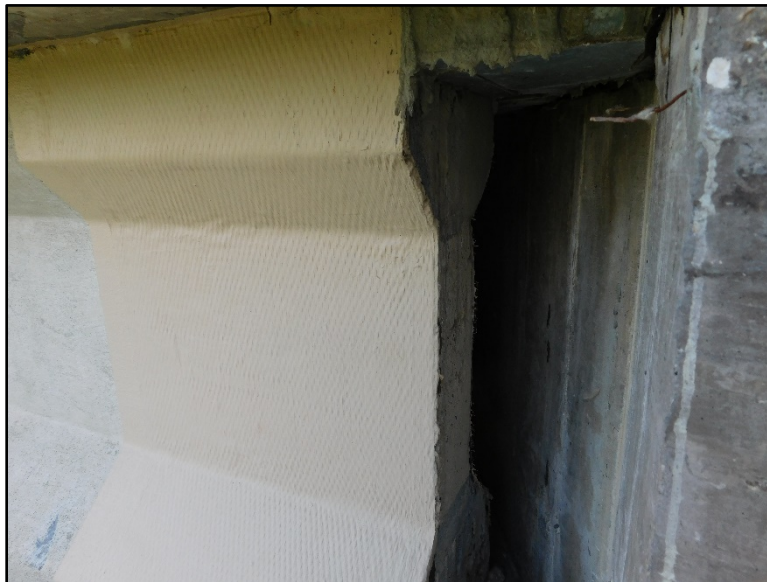
Figure B.67 Beam end repair at south end abutment of southbound bridge.
