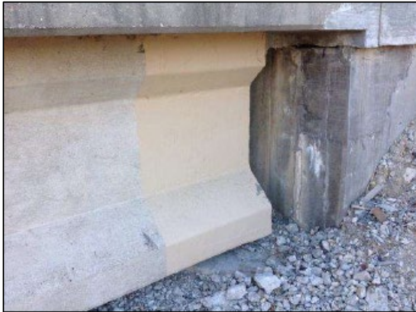
Figure B.63 Fiber Wrapped End of Beam 1 at Abutment 1 (from Schamberger (2016b) inspection report)
