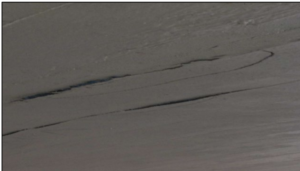
Figure B.13 Debonding of CFRP on underside of arch ring at center span (from Dittrich (2014) inspection report).
