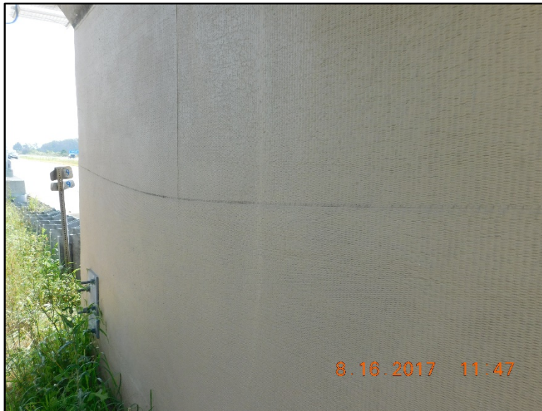
Figure B.117 Sag in transverse column wrap at northern pier.
