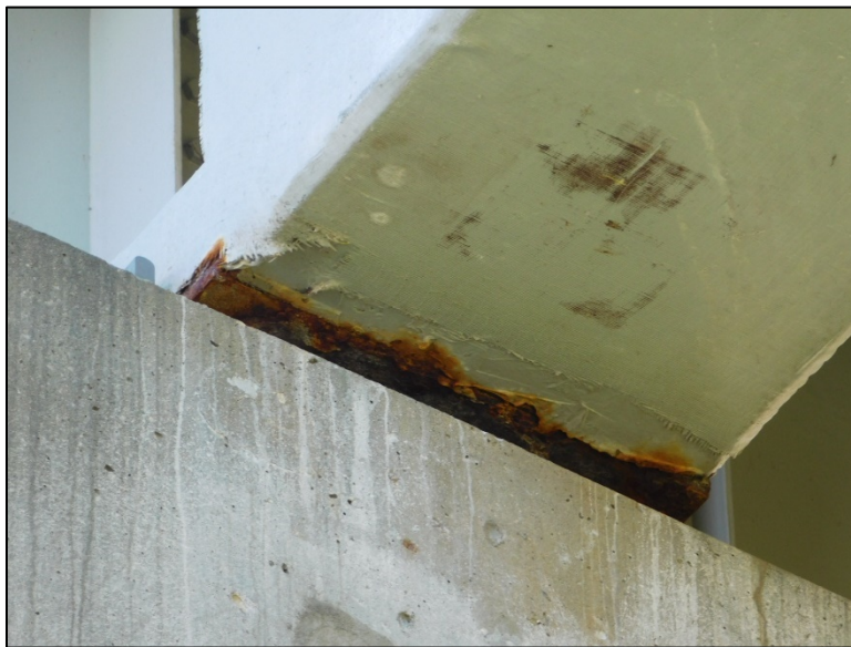
Figure B.168 Corrosion at beam end near support location.
