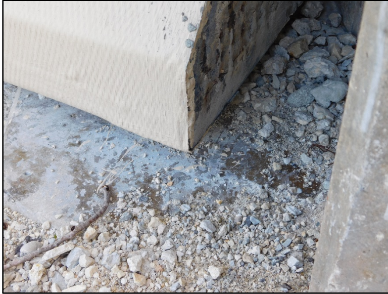
Figure B.68 Debonding of FRP at beam end.
