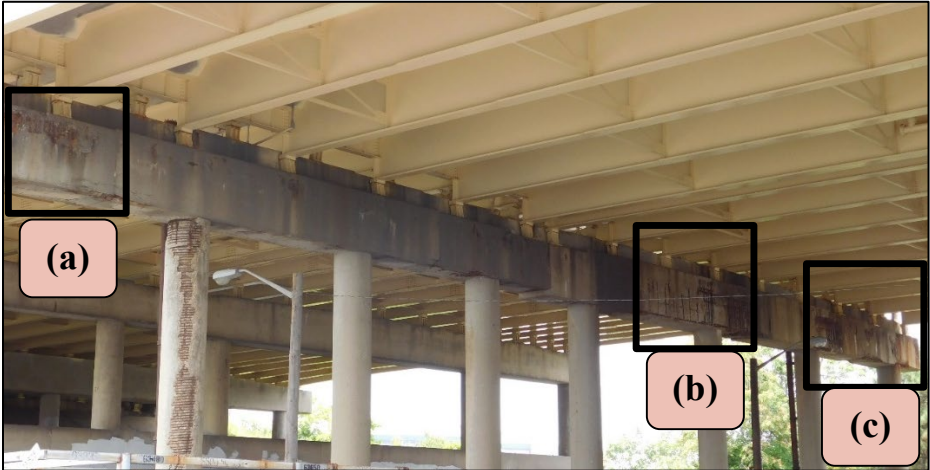
Figure B.181 Deterioration of pier caps.
