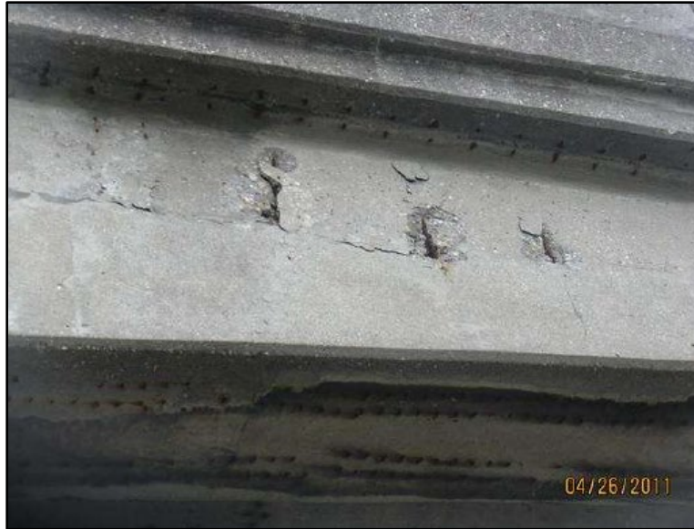
Figure B.28 Spalling and delamination with exposed rebar on girder (from Smith (2011) inspection report).
