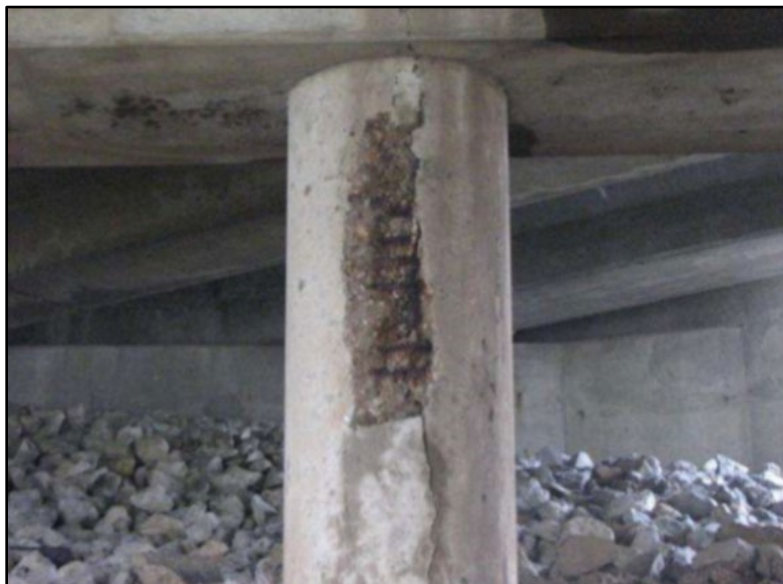
Figure B.92 Spalled column with exposed steel at Pier 2 (from Bewley (2011a) inspection report).
