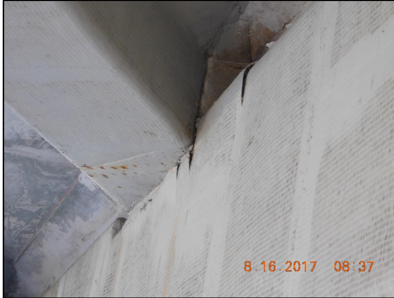
Figure B.101 Cracking and peeling of beam cap wrapping at beam end support.
