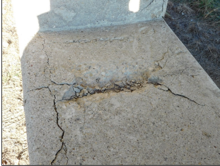
Figure B.176 Spalling of Pier 3.
