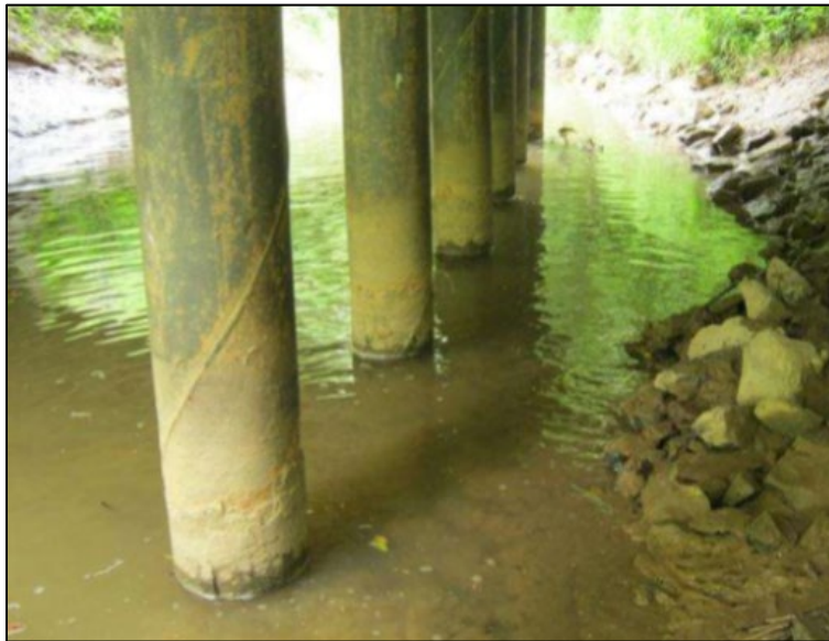
Figure B.148 Pile deterioration at eastern pier (from Conner (2011) inspection report).
