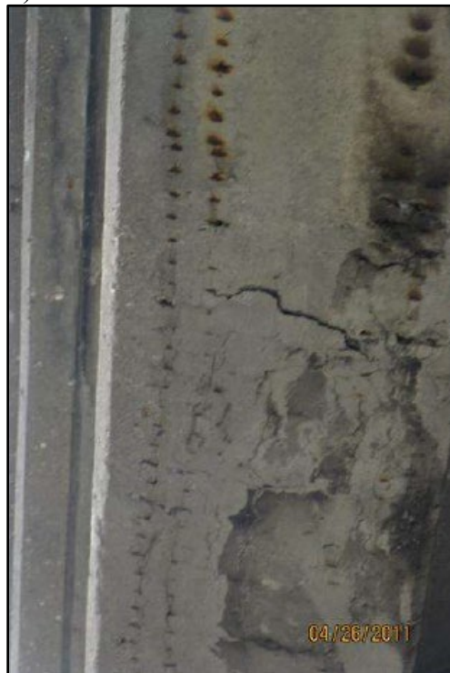
Figure B.31 Delamination at bottom of girder (from Smith (2011) inspection report).
