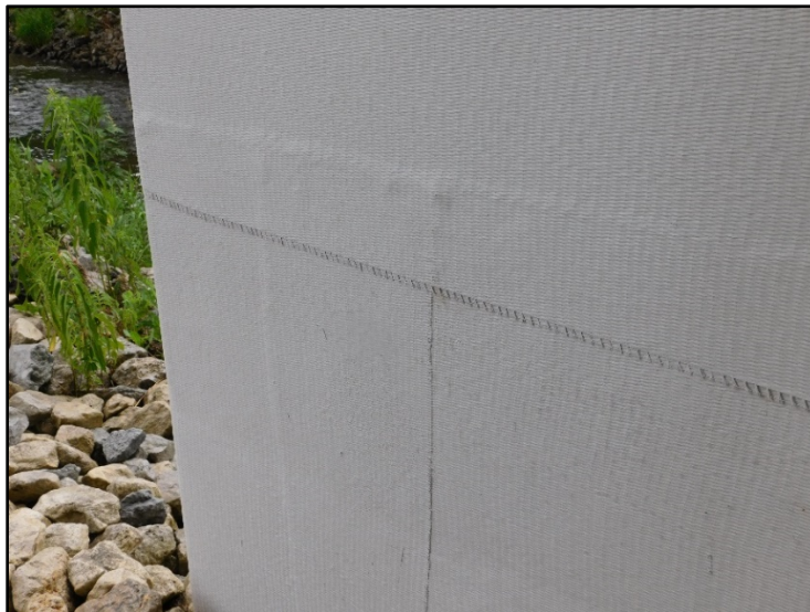
Figure B.81 Sheet overlapping of pier adjacent to Blue River.
