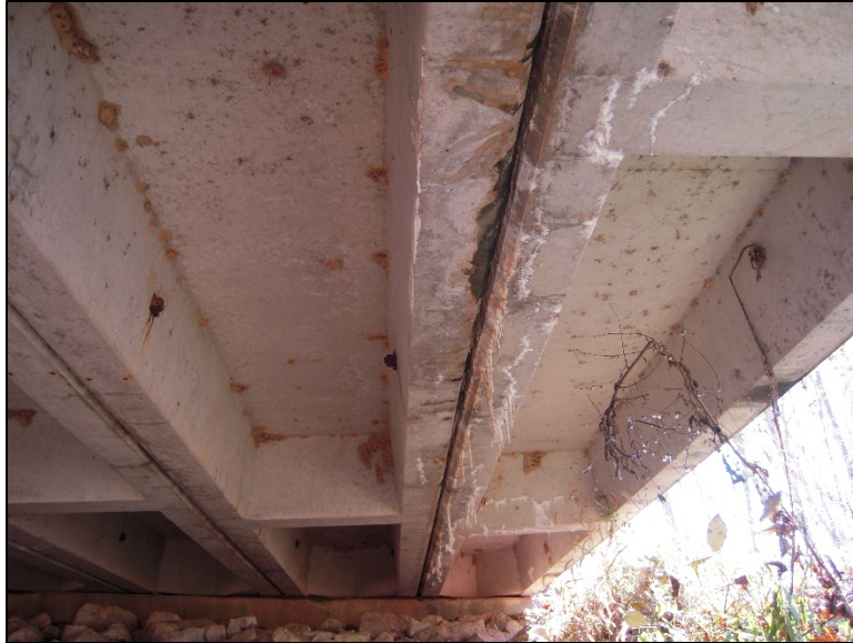
Figure B.154 Seepage at fascia beam in easternmost span.
