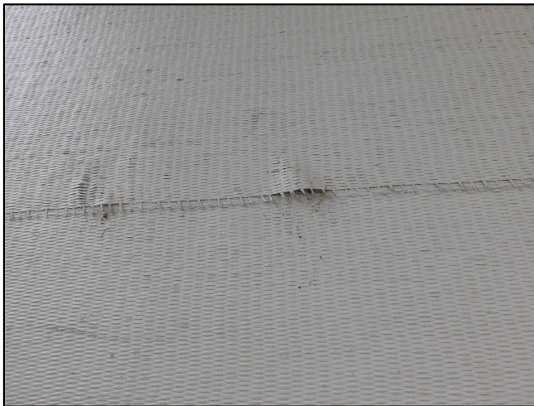
Figure B.83 Local debonding of wrap.
