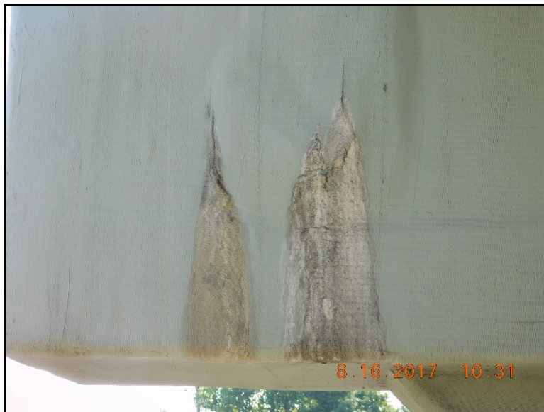
Figure B.110 Large area of void and discoloration at northwestern pier cap.
