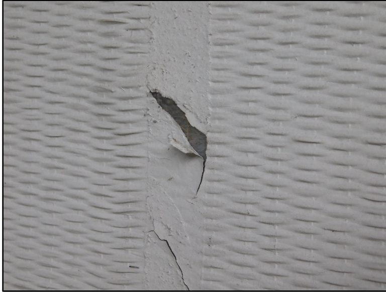
Figure B.84 Cracking and tearing of paint.
