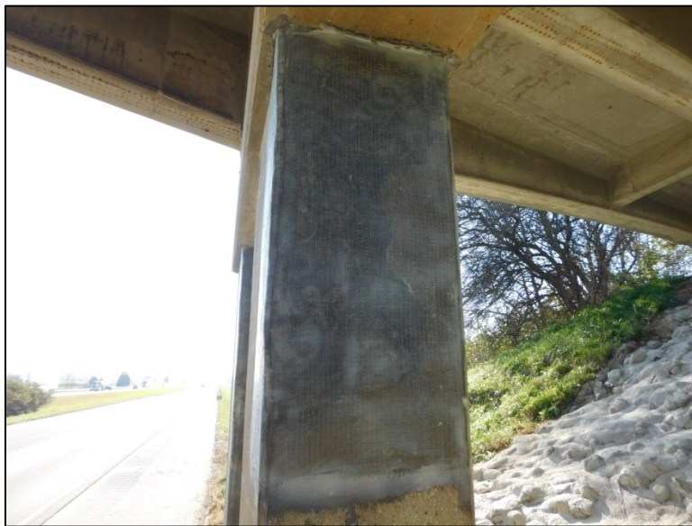
Figure B.173 Larger column patch at northern pier.
