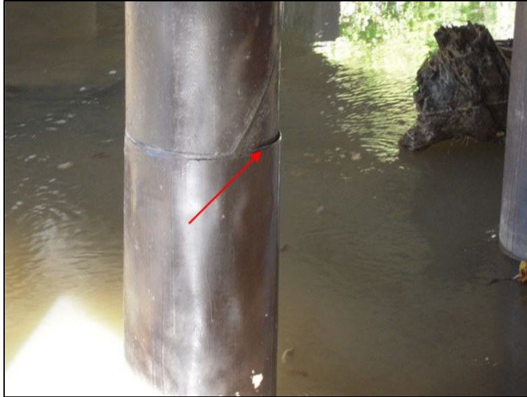
Figure B.152 Debonded area at top of column wrap.
