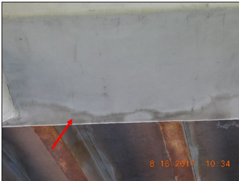
Figure B.112 Discoloration at northwestern pier cap.
