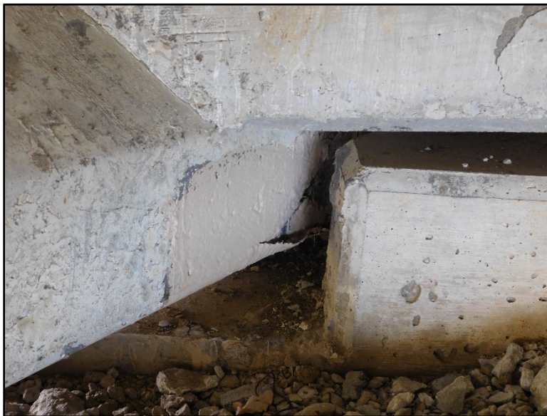
Figure B.69 Local debonding at interior beam end.
