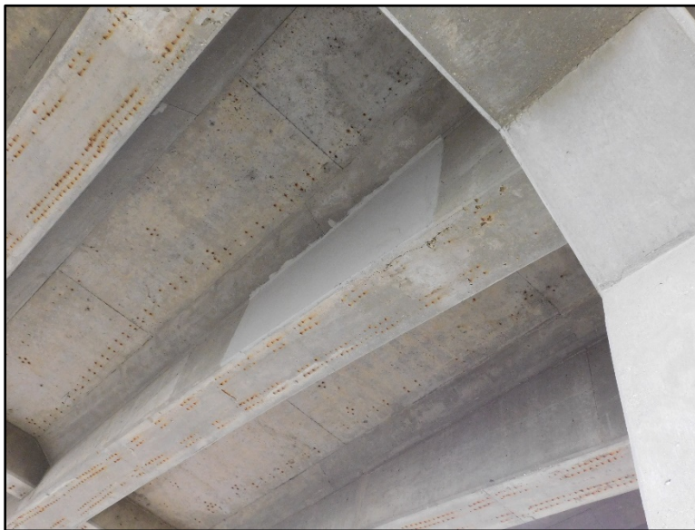
Figure B.36 One-sided repair of middle beam on eastern side of middle pier.
