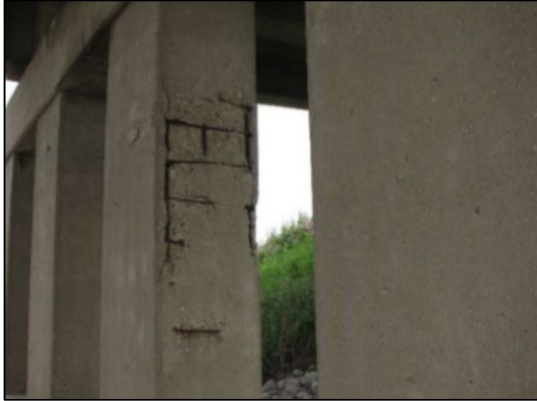
Figure B.131 Spalling and exposed rebar at Pier 4 (from Bewley (2009) inspection report).
