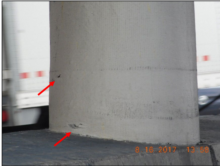
Figure B.127 Inconsistent layering of FRP sheets with signs of vehicle damages.
