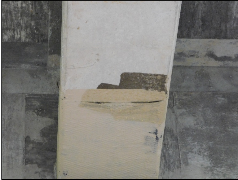
Figure B.60 Local debonding at beam ends at Pier 7.
