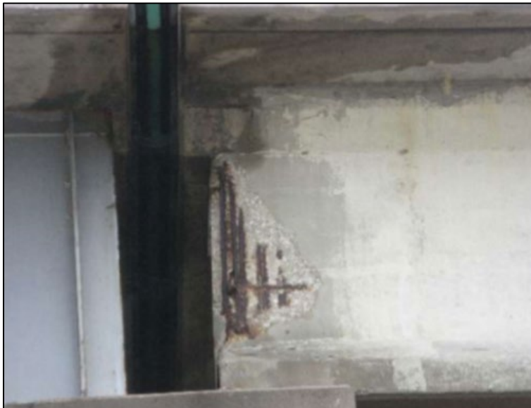
Figure B.158 Beam end deterioration at Pier 22 (from Everman (2010) inspection report).
