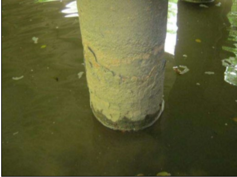
Figure B.147 Pile deterioration at eastern pier (from Conner (2011) inspection report).
