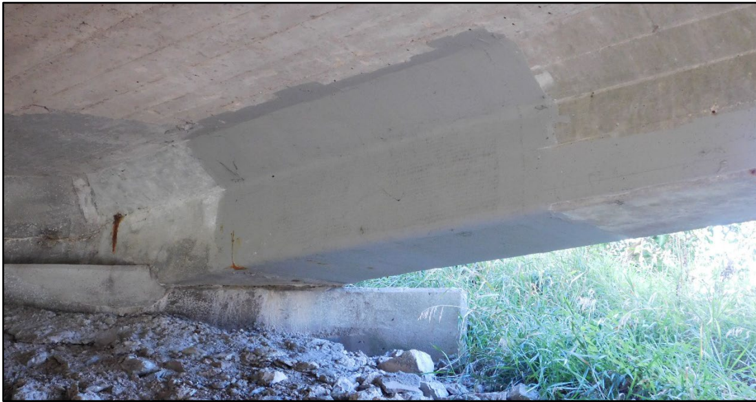
Figure B.93 Beam end repair of fascia girder at southern abutment.
