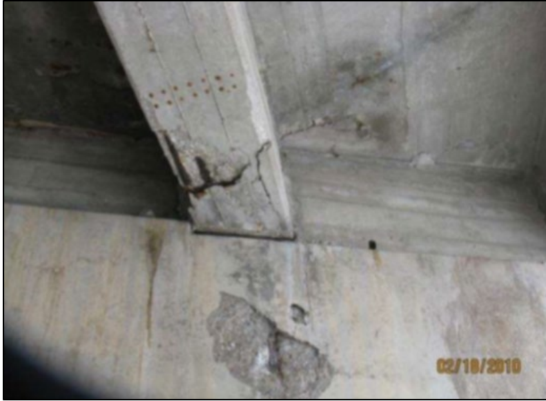
Figure B.77 Spalled beam end and exposed rebar at eastbound bridge (from Smith (2010a) inspection report).
