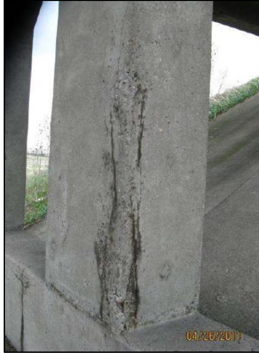
Figure B.30 Vertical delamination to the southwest corner of column at Pier 4, Span C (from Smith (2011) inspection report).
