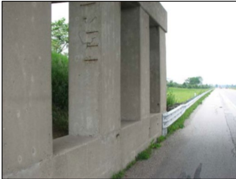
Figure B.129 Spalling and exposed rebar at Pier 2 (from Bewley (2009) inspection report).
