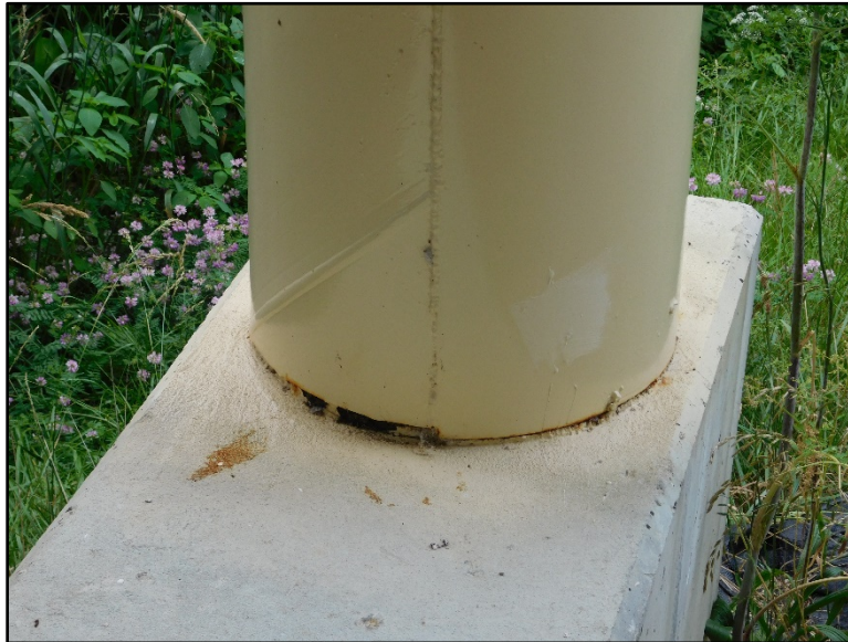
Figure B.55 Corrosion at base of steel jacket.
