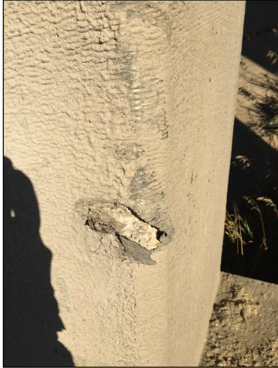
Figure B.144 Large tear in westernmost column wrap.
