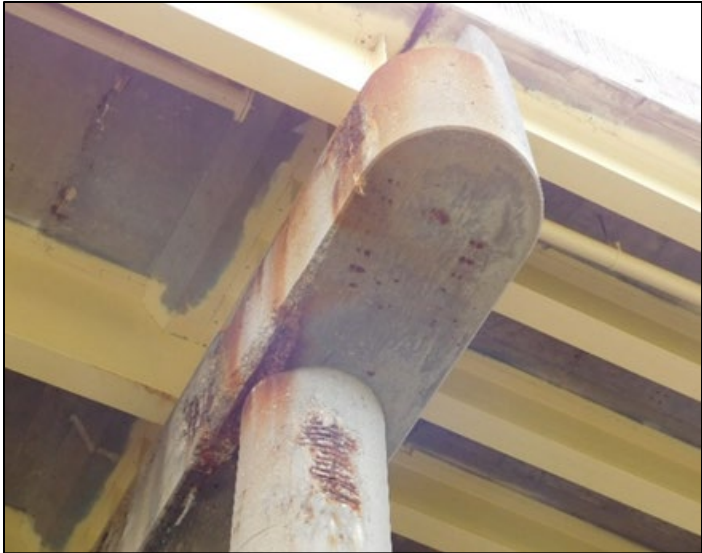
Figure B.180 Deterioration of fascia column at I-70 westbound pier.
