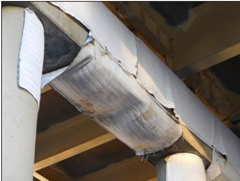
Figure B.185 Use of insulated curing blankets for temperature control after shotcrete application.
