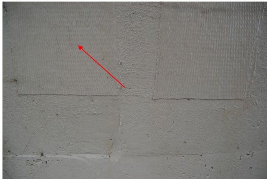
Figure B.15 Possible hairline cracks in CFRP sheet.
