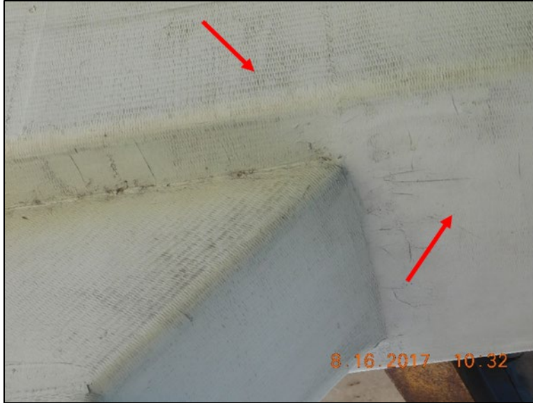
Figure B.111 Inconsistent use of epoxy at pier cap-to-column intersection.
