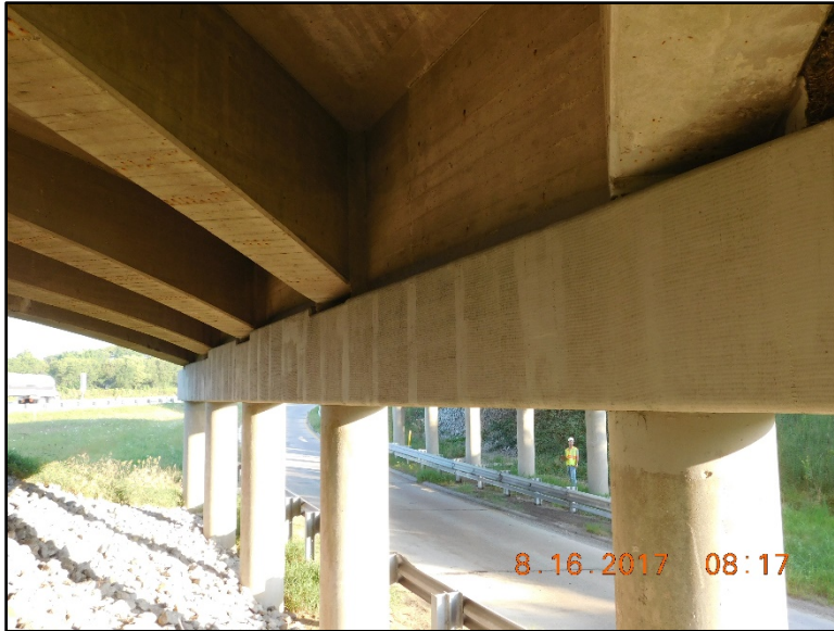
Figure B.95 Wrapped pier cap at Pier 2.
