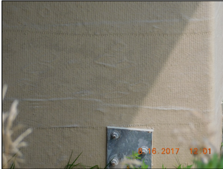
Figure B.120 Areas of voids on the repaired surface of the southern pier.
