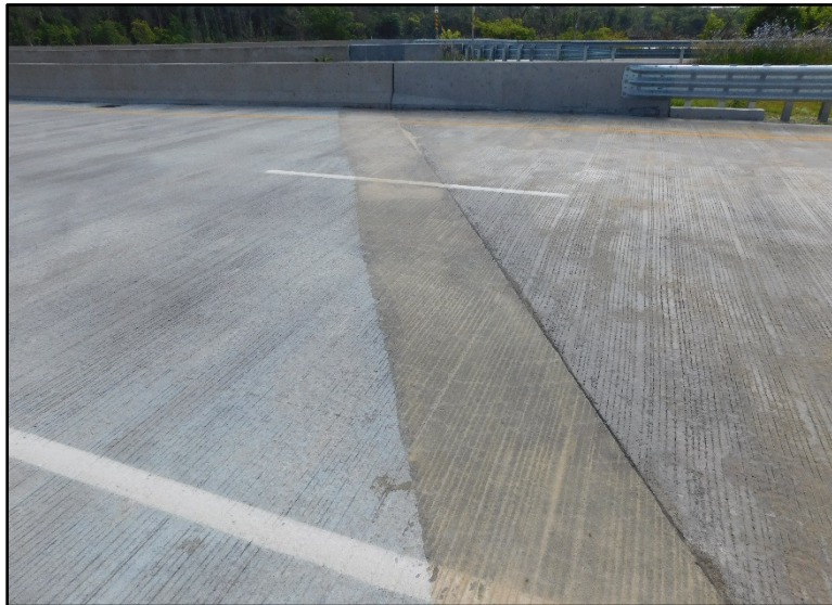
Figure B.65 Top of deck above the south end abutment of southbound bridge.
