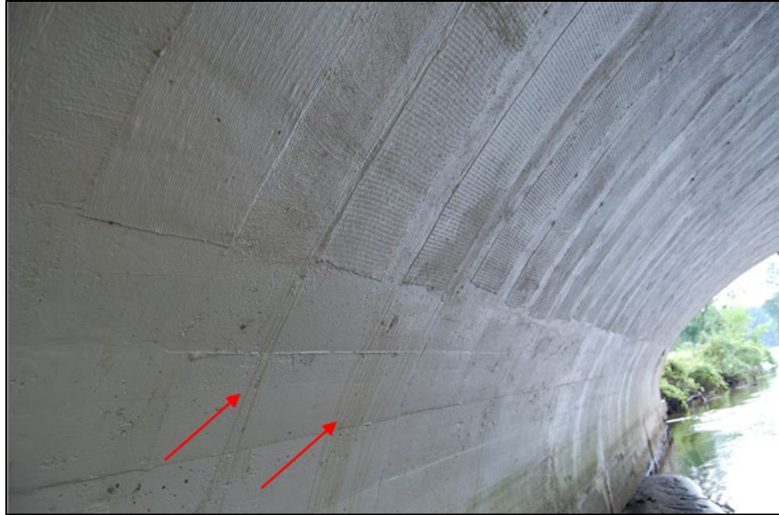
Figure B.12 Epoxy runoff.
