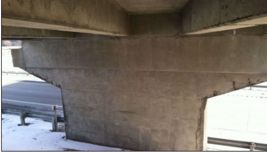
Figure B.40 Pier 2 Deterioration (from Biller (2015a) inspection report).
