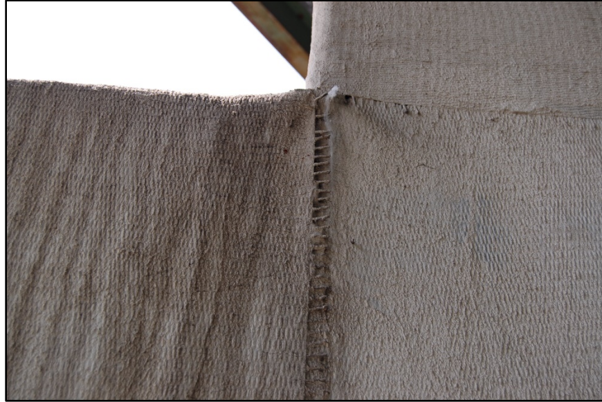
Figure B.22 GFRP sheet overlapping and sheet detail at column to crashwall intersection.
