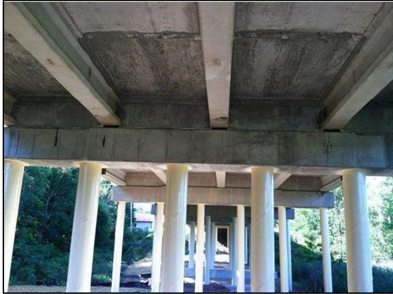
Figure B.53 Repaired beam ends, new bent cap, and encased piles at Bent 7 (from Biller & Gimbel (2014) inspection report).
