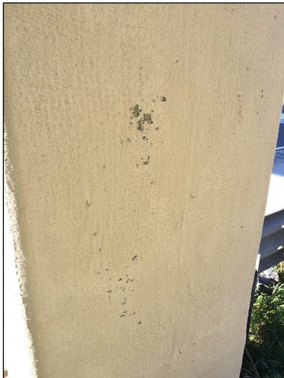
Figure B.145 Areas of chipped paint on column wraps.
