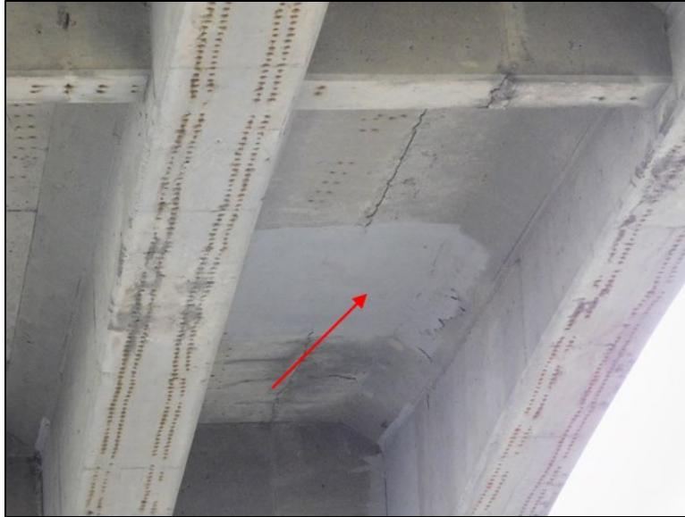
Figure B.35 Possible FRP repair to underside of deck over I-69 SB.
