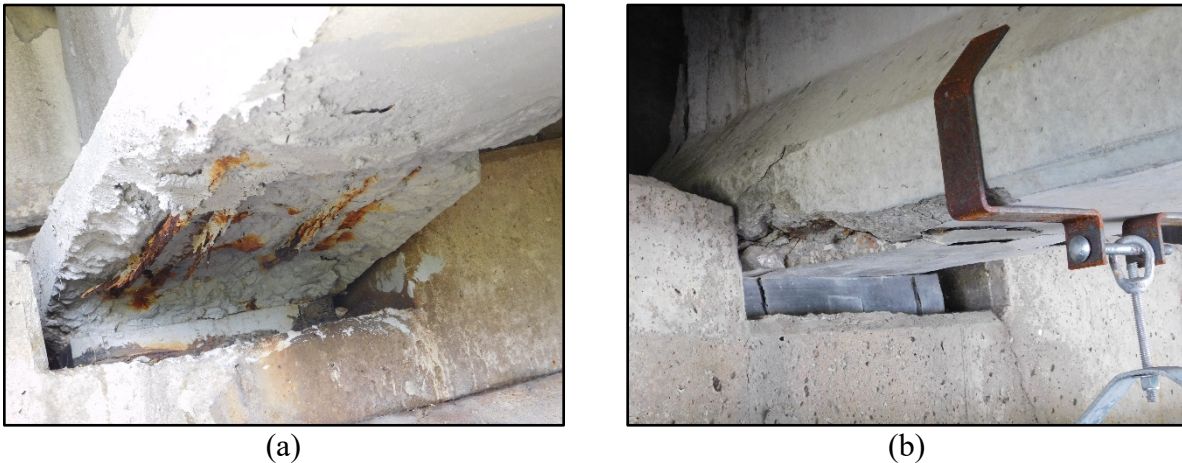
Figure C.4 Beam end region deterioration.
