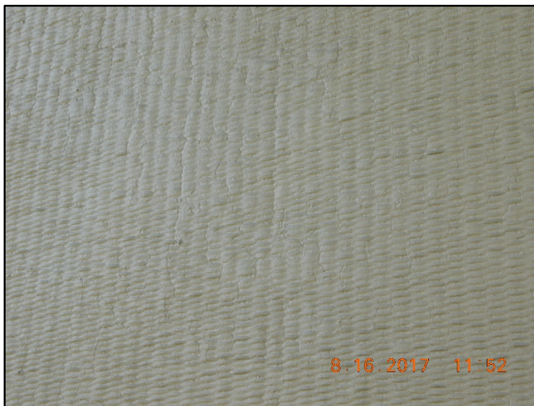
Figure B.119 Possible UV damage.
