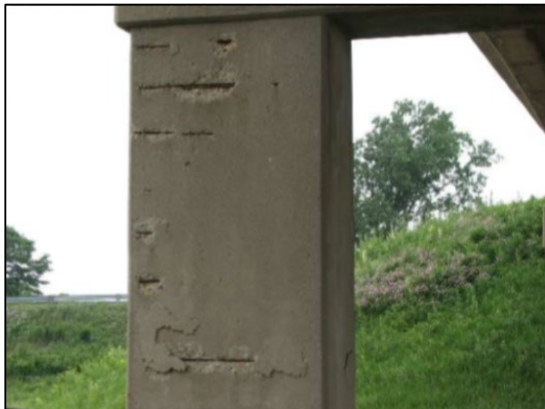
Figure B.130 Spalling and exposed rebar at Pier 3 (from Bewley (2009) inspection report).
