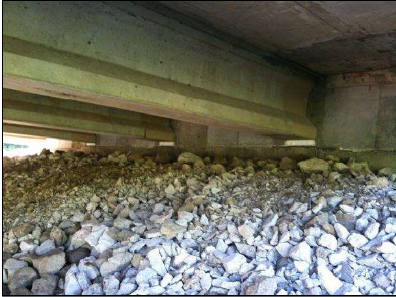
Figure B.51 Beam end region wrapping at Abutment 1 (from Biller & Gimbel (2014) inspection report).
