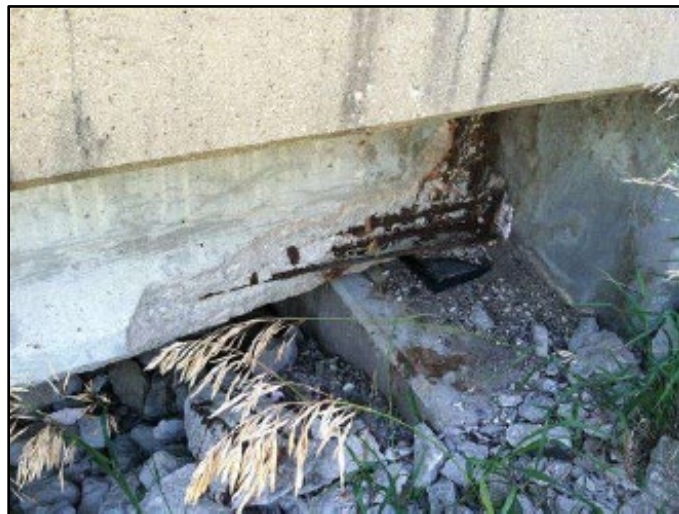
Figure B.48 Spalling and exposed strands at Beam 1 in Span A (from Biller (2013) inspection report).
