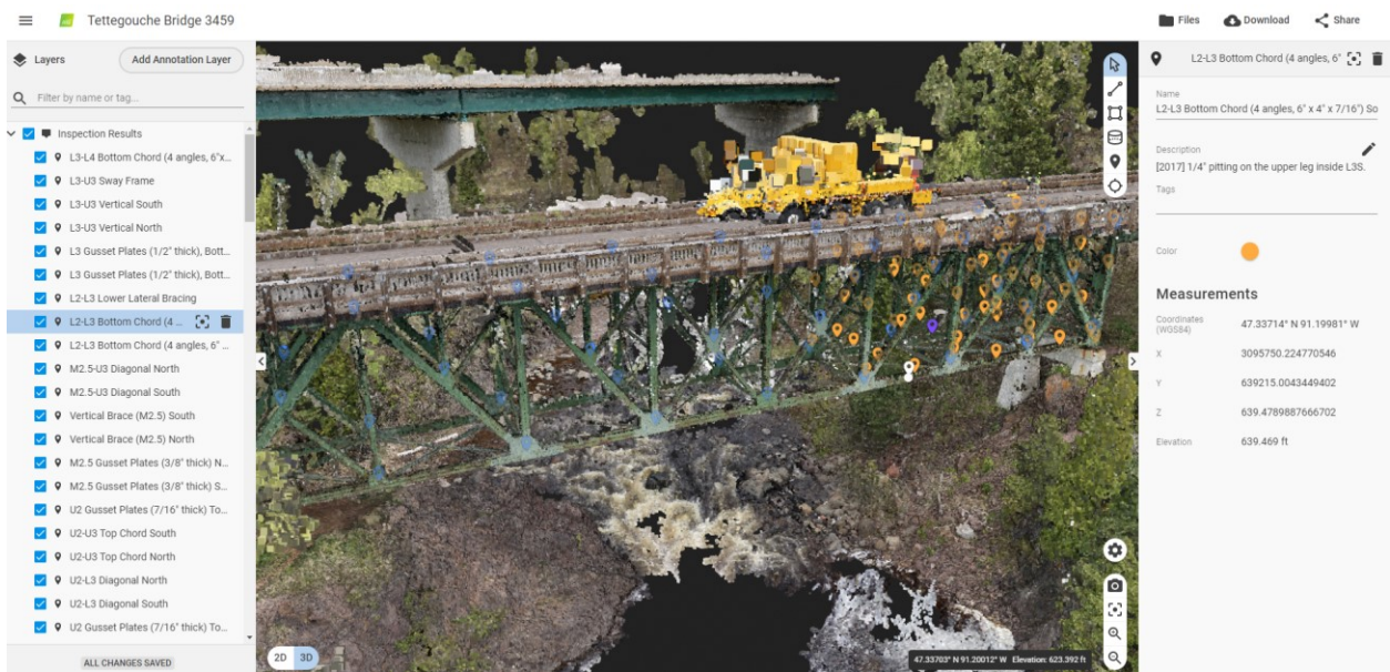
Figure 1- 10 Inspection Results Annotation
