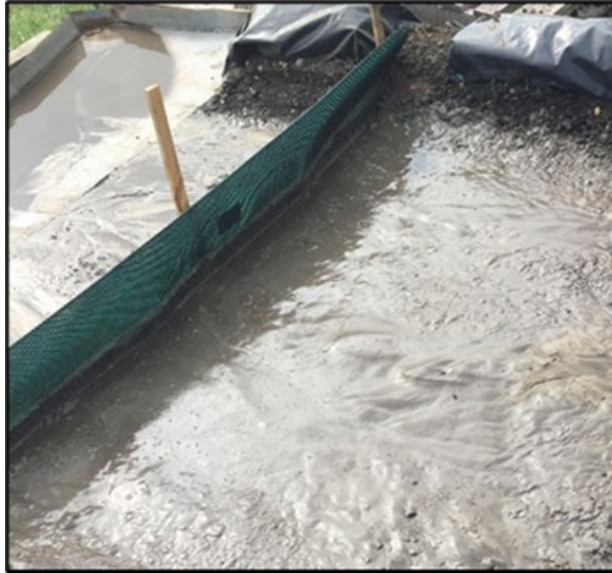
A. Ponding height upstream within 1 hour of ending the test
