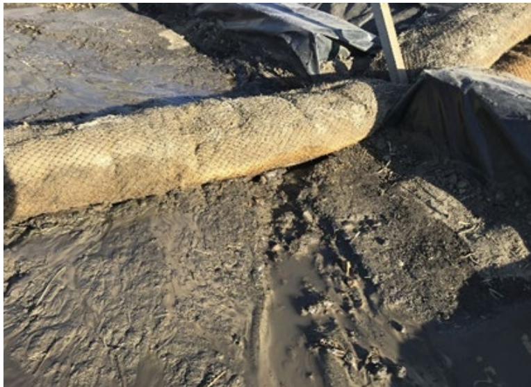
B. Undercutting downstream
