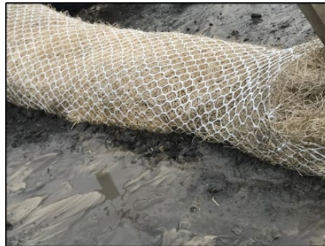
A. Undercutting still occurred in spite of 45° angle staking
