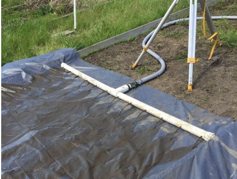
Figure 20. Photo. Dispersion pipe attached to ball valve/mixing tank.
