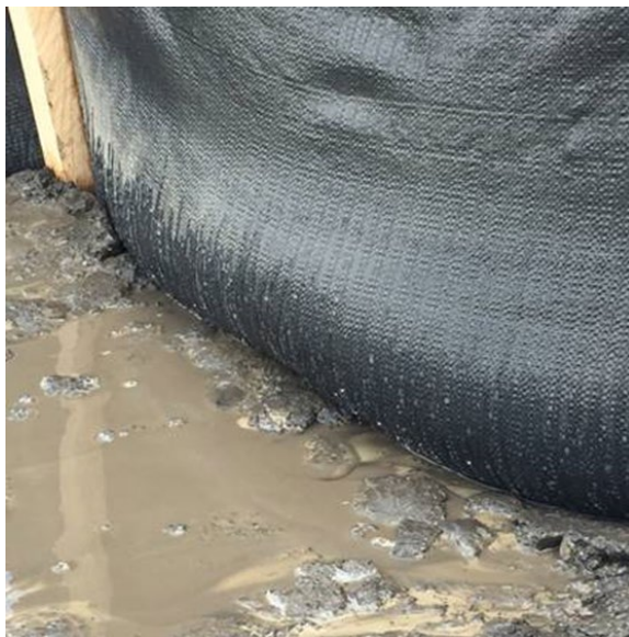
Figure 25. Photo. Clogging of silt fence during testing.
