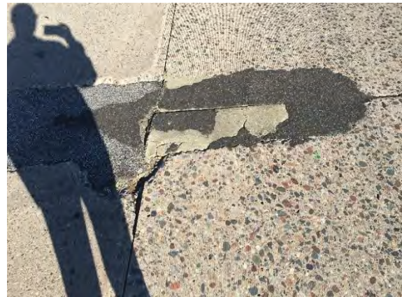
Figure 4.5 Patch Condition Rating = 1 [Linear cracks and >50% material loss]
