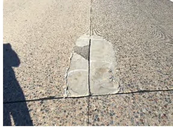
Figure 4.4 Patch Condition Rating = 2 [Linear cracks and <50% material loss]
