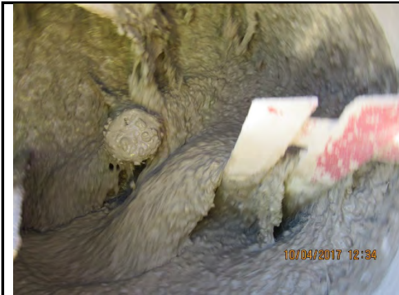
Photograph: 94013 CTS, Rapid Set and Helix Fiber Subject: Mixing of bagged product, aggregate, and fibers
