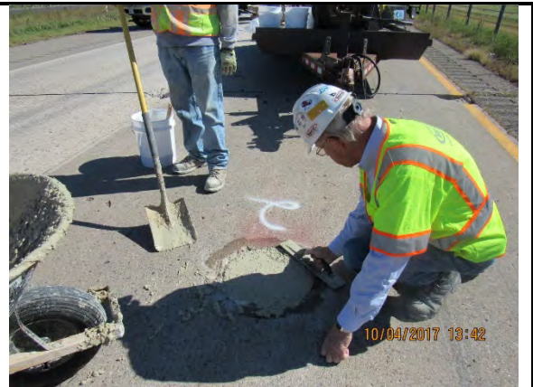
Photograph: 94013 CTS, Rapid set and Helix Fiber Subject: Finishing of products with steel fibers
