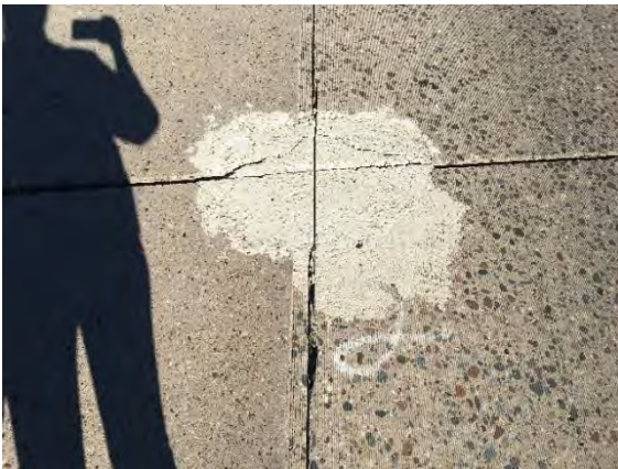
Figure 4.3 Patch Condition Rating = 3 [Linear cracks]
