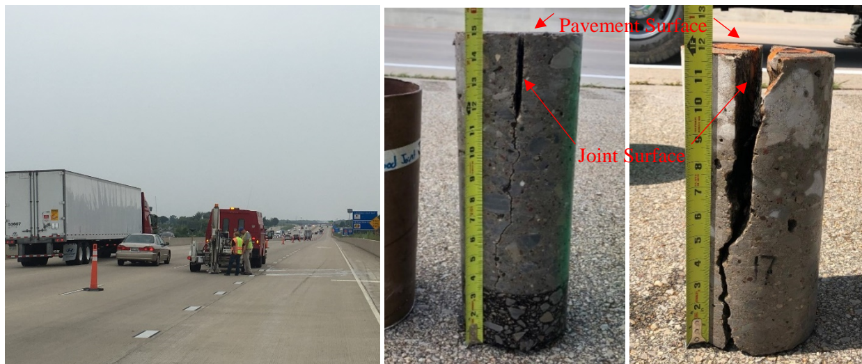
Figure 3.2 (a) Taking field cores (b) A core sample of good joint (c) A core sample of spalled joint
