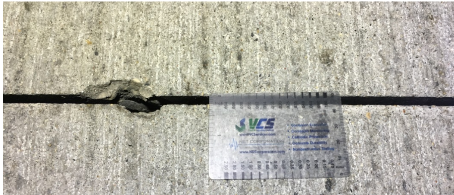
Figure 5.5 Close-up of small spalling at Joint #104
