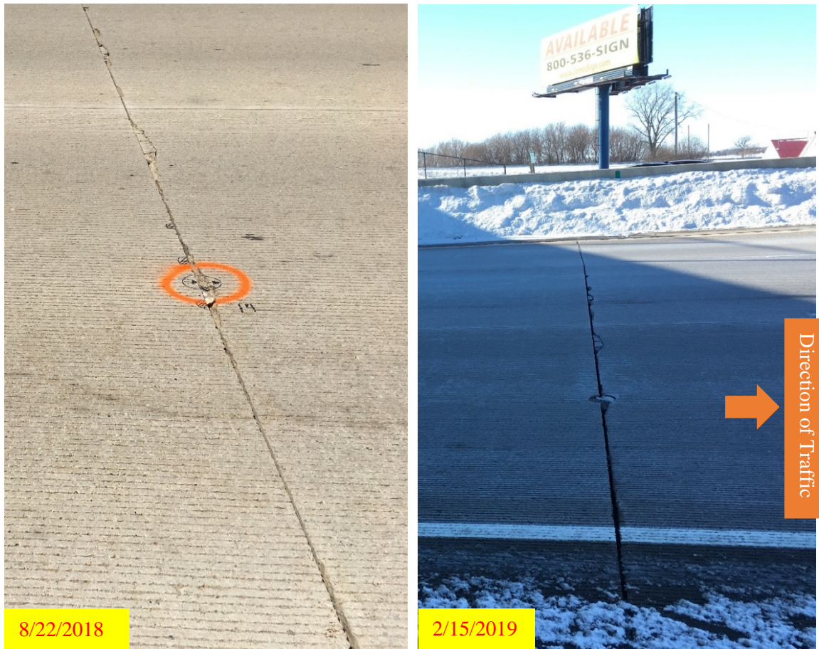
Figure 3.10 Picture Taken from Shoulder of Core #14 Joint on I-41
