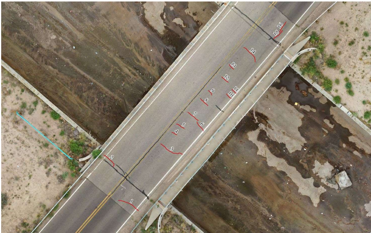
Figure 34. The locations of the cracks identified through field survey.
