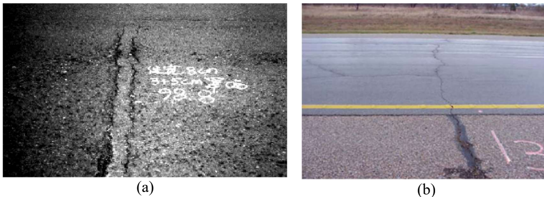
Figure 1. Types of reflective cracking, (a) double (b) single (22).
